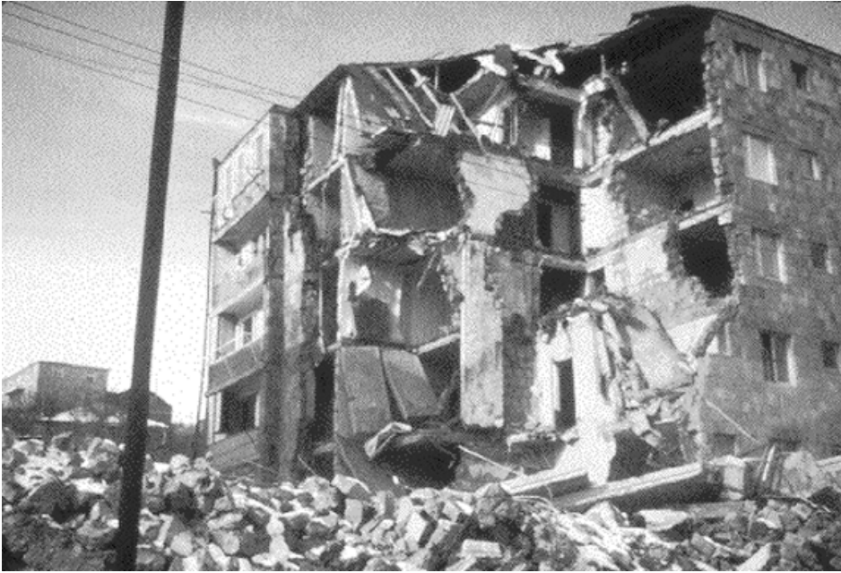
▲ Partial destruction of a five-story stone masonry bearing-wall building in Spitak.
