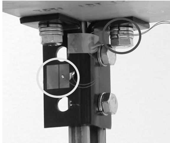
Figure 12: Close-up of a joint with bonded PZT patch (light circle) and loosened bolt in damage case (dark circle)
