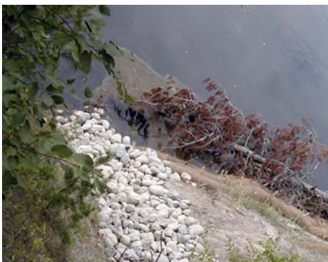
-USFWS/Heather Rawlings The addition of large woody debris adds the finishing touch to repair a stream bank erosion site on the AuSable River in Michigan.
