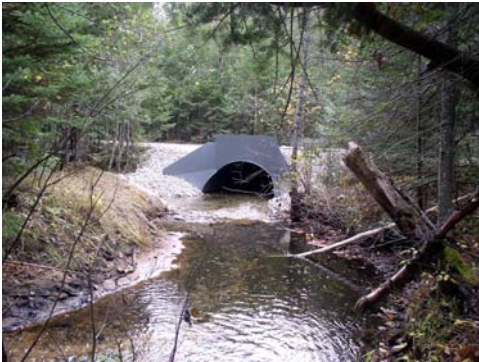
-USFWS photo by Susan Wells This bottomless culvert replaced two undersized, perched culverts on the Little Ocqueoc River.
