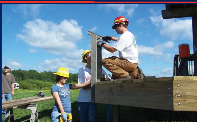
Above: YCC crew putting up the railings for the disabled access viewing deck at Rice Lake NWR. Photo by Peter Rea;
