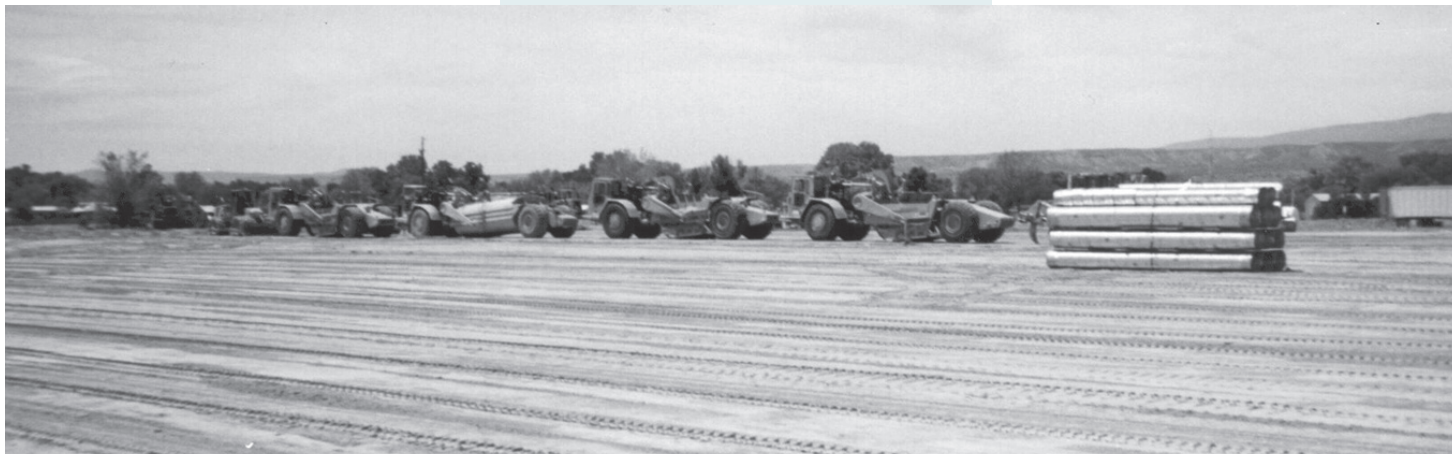
One of Tsay Corporation's most recent development initiatives is its new airport which, when complete, will have a 5,200-foot runway. Both Governor Salazar and Lovato hope to use the airport as a catalyst for increased economic development in Northern New Mexico.
