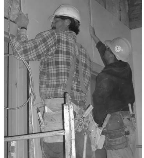
Darnell Tsosie (pictured on the right) works on the EOC building as an apprentice drywaller.
