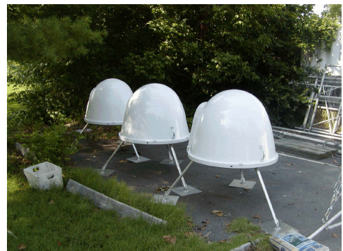
Figure 3. Enclosures that will contain the ET probe computers and batteries.
