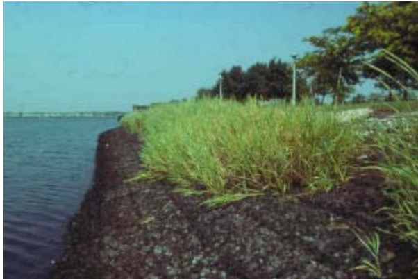
Figure 12. Installation of wire mesh baskets filled with small stone can alleviate the undercutting associated with many docks. It has the additional benefit of providing habitat for Spartina and is an improvement over bulkheads.
