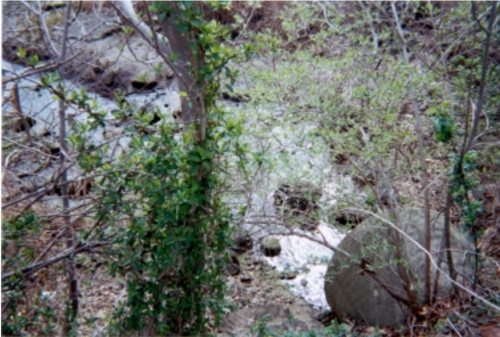
Photograph 15: The 24 stormwater outfall that discharges into the Bar Beach Lagoon that runs under Shore Road and the trail way discharges into the lagoon once it enters the lagoon. This photograph was taken at low tide in the lagoon and on a clear non-rainy day, thus the outfall appears to have a continuous discharge. The discharge appears to have created the channels that meander throughout the tidal flats. The County, according to Denise Herrington of the town of North Hempstead, apparently owns the outfall.
