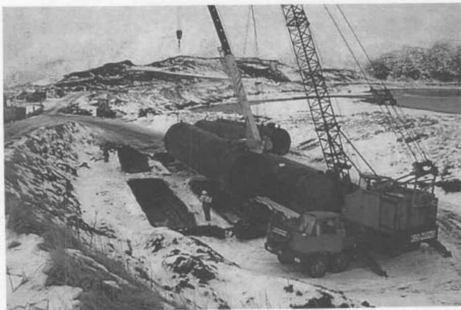
Figure 8: Temporary Tank Farm at Summer Bay Beach
