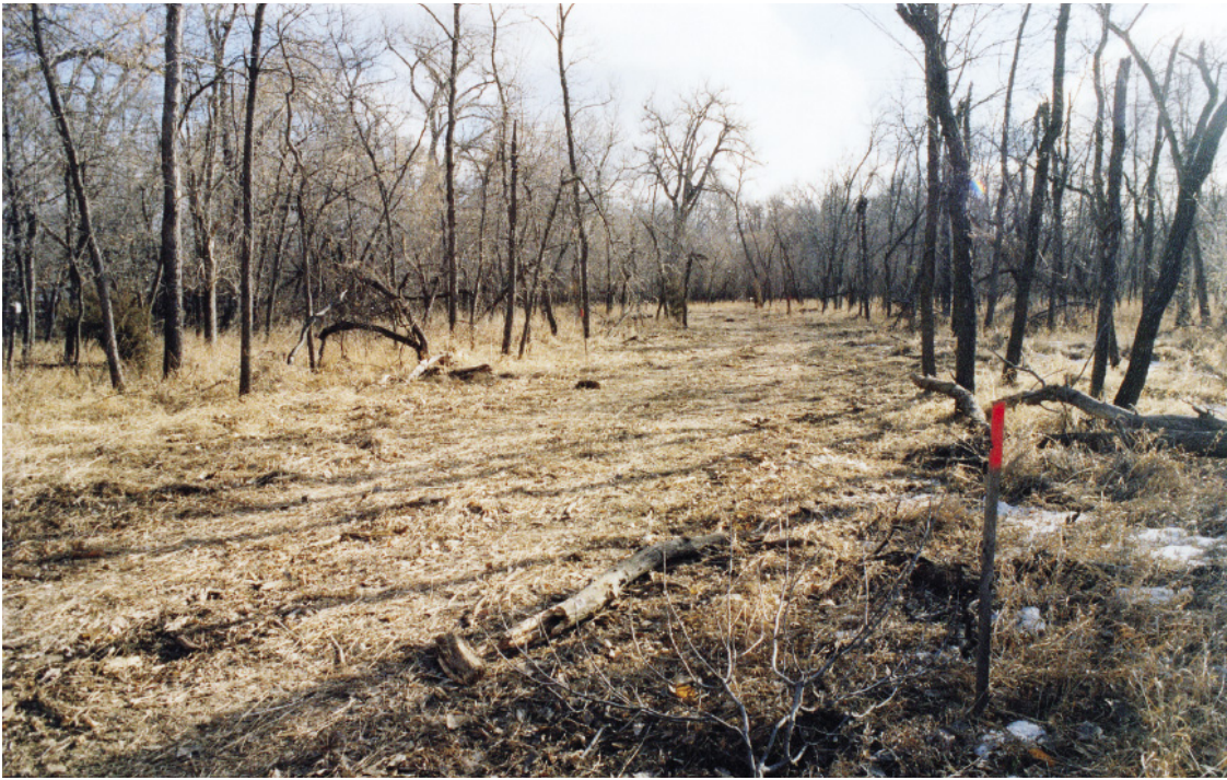
A finished section of fire trail, its edge marked by the orange-tipped stake
