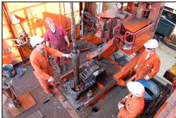
Figure 3: Drill floor on board REM Etive, with the FPC being loaded into the drillstring prior to lowering and coring.
