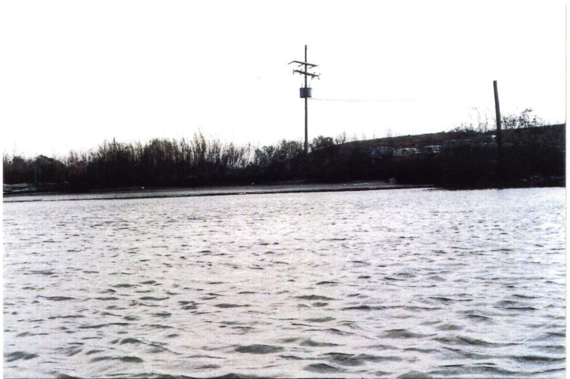
PHOTO NO. 23 - RECEEDING EAST SIDE BANK CAUSED BY EROSION.
