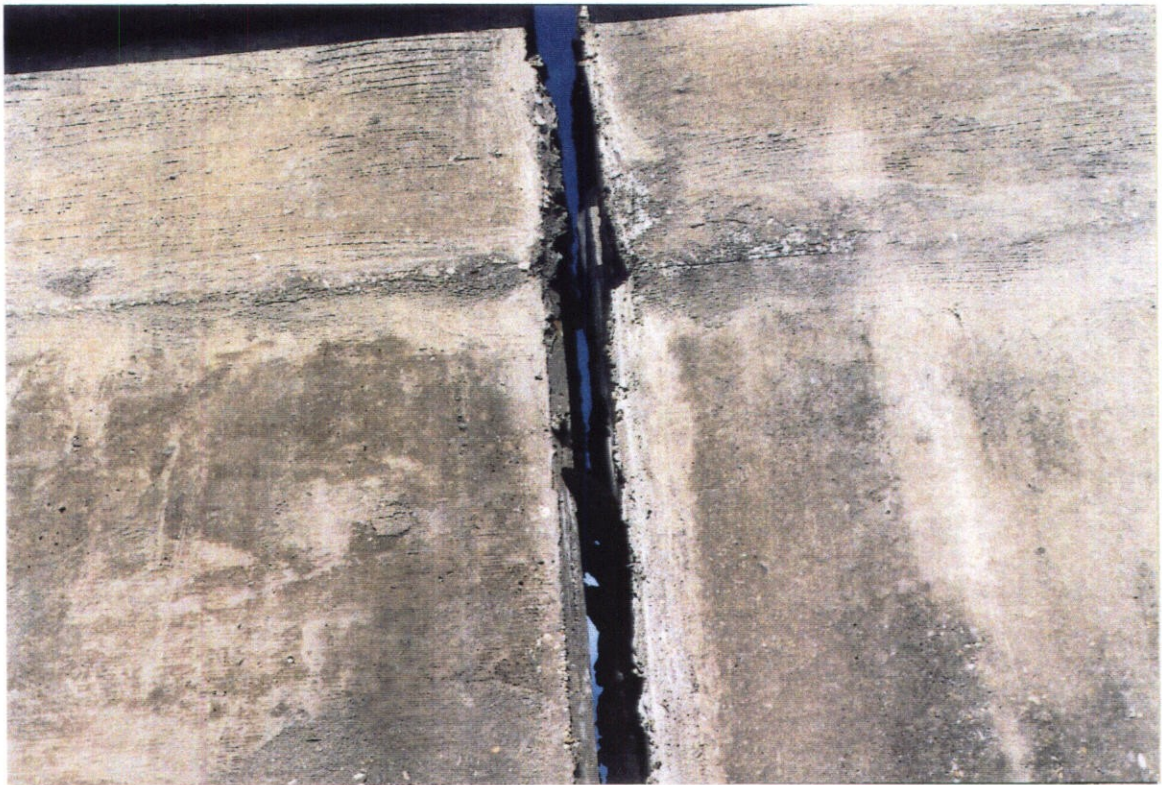
PHOTO NO. 3 - JOINT BETWEEN FLOODWALL MONOLITHS T-3L AND T-4L. NOTE TORN WATERSTOP.
