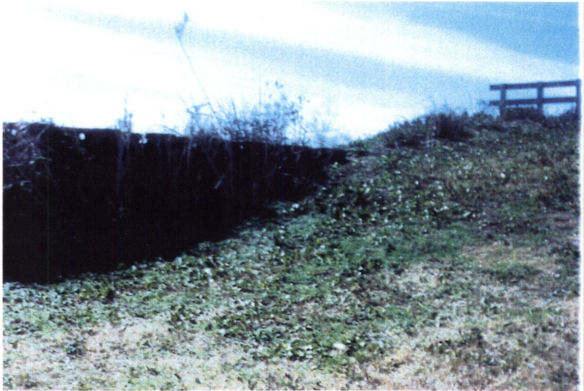
PHOTO NO. 26 - WEST END OF WEST SHEET PILE FLOODWALL. NOTE SETTLEMENT.
