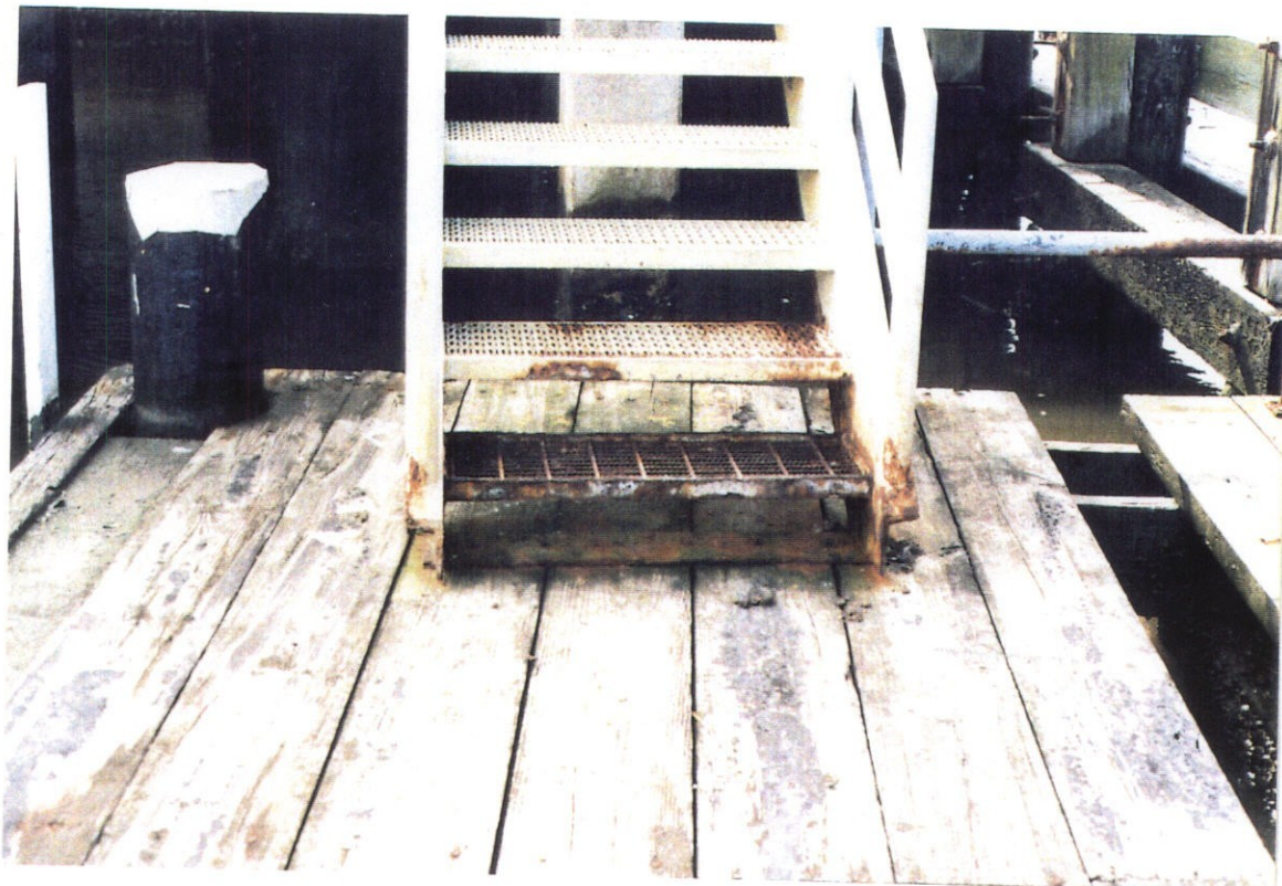
PHOTO NO. 5 - BADLY CORRODED BOTTOM TREAD AND ATTACHMENT PLATE ON STAIRWAY TO BOAT DOCK. NOTE MISSING DECK BOARD.
