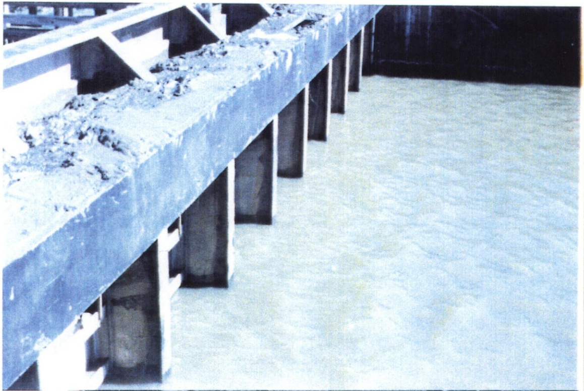
PHOTO NO. 8 - VIEW LOOKING EAST AT THE UNDERSIDE OF THE GATE. GATE IS IN THE FULLY CLOSED POSITION. NOTE LINES ON VERTICAL MEMBERS MADE BY SILT LINE WHEN THE GATE WAS OPEN (LOWERED INTO ITS RECESS).
