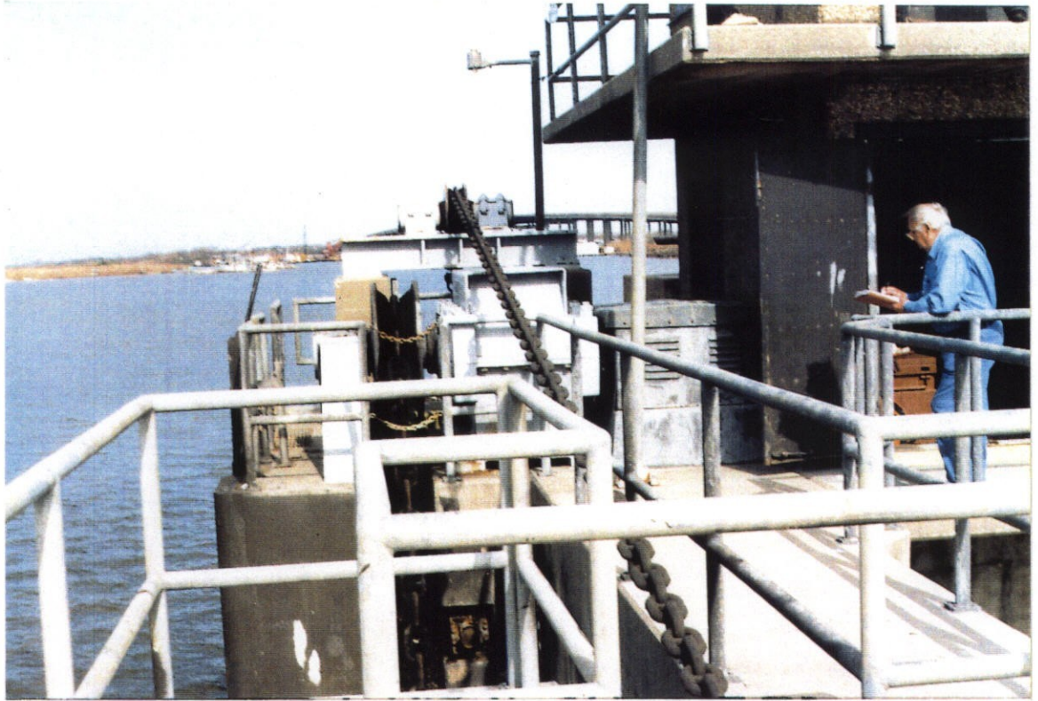
PHOTO NO. 10 - GATE OPERATING MACHINERY ON THE EAST SIDE.
