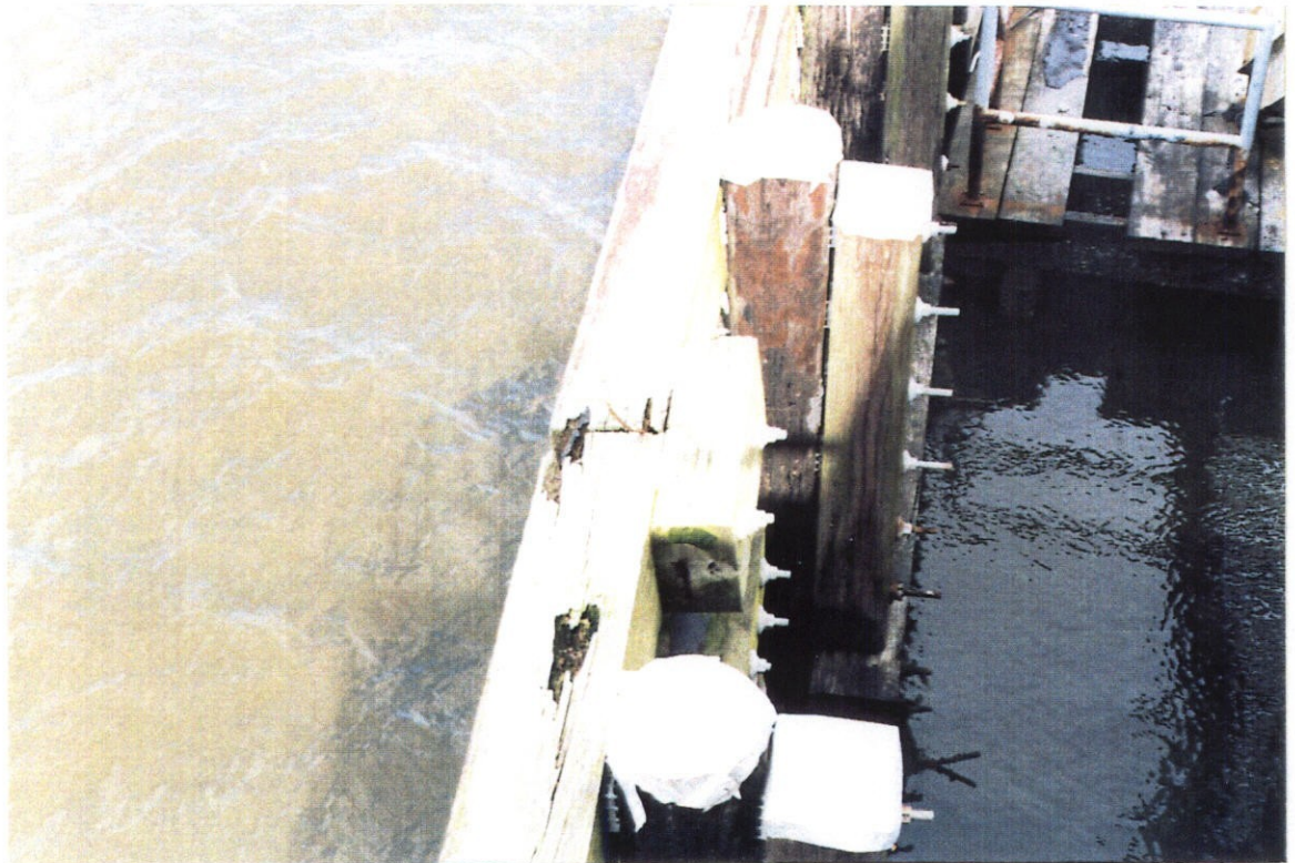
PHOTO NO. 21 - NORTHWEST GUIDEWALL. NOTE DETERIORATED TIMBERS.
