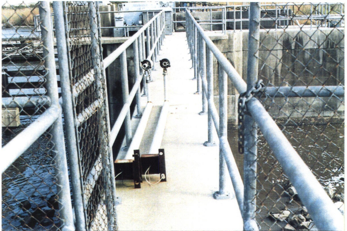
PHOTO NO. 17 - LIGHT POLES REMOVED AND STACKED ON THE ACCESS WALKWAY ON TOP OF THE WEST FLOODWALL.
