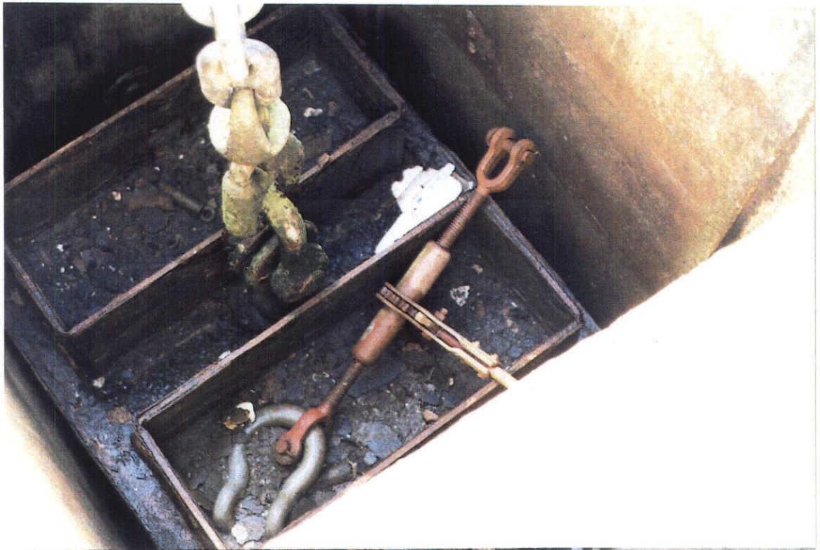
PHOTO NO. 13 - TOP OF WEST SIDE COUNTERWEIGHT. NOTE DISCONNECT LOAD BINDER RATCHET LYING ON TOP OF THE COUNTERWEIGHT.
