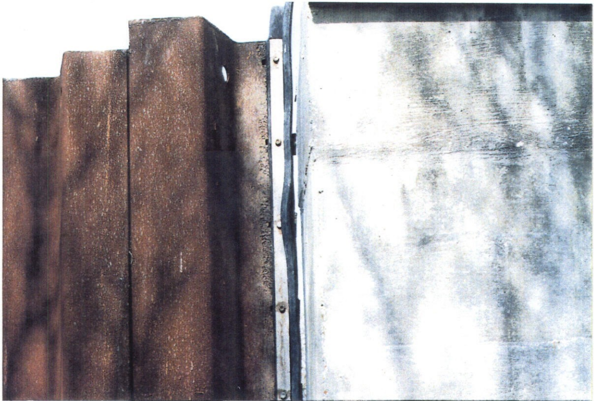
PHOTO NO. 2 - JOINT BETWEEN FLOODWALL MONOLITH T-4L AND THE WEST SIDE SHEET PILE FLOODWALL SHOWING THE GAP BETWEEN THE L TYPE SEAL AND MONOLITH T-4L.
