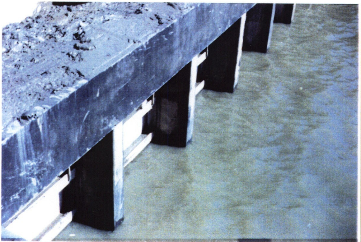
PHOTO NO. 15 - VIEW SHOWING SLIGHT AMOUNT OF TURBULENCE FROM GATE RECESS FLUSHING SYSTEM WITH GATE FULLY CLOSED (RAISED) DURING THE SUPPLEMENTAL GATE INSPECTION ON 13 FEBRUARY 1996.
