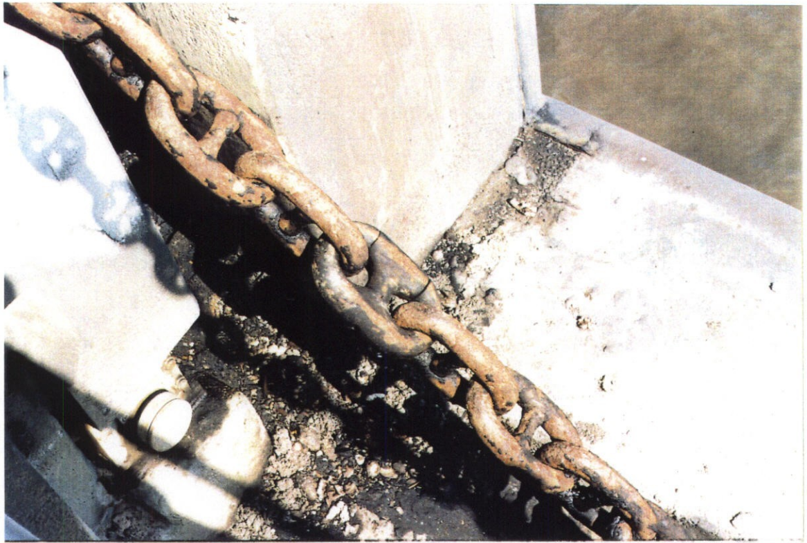
PHOTO NO. 12 - WEST SIDE HOIST CHAIN. NOTE CORROSION AND CONNECTING LINK INSTALLED TO REPLACE A FAILED LINK.
