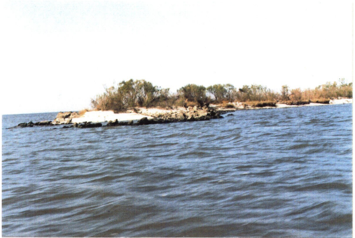
PHOTO NO. 22 - STONE BREAKWATER AT THE SOUTHWEST END OF THE CHANNEL. NOTE LOSS OF STONE FROM THE END OF THE BREAKWATER.
