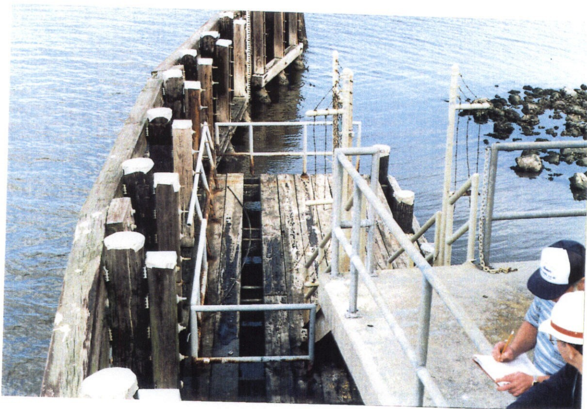
PHOTO NO. 6 - BADLY DETERIORATED HANDRAILS ON THE BOAT DOCK.
