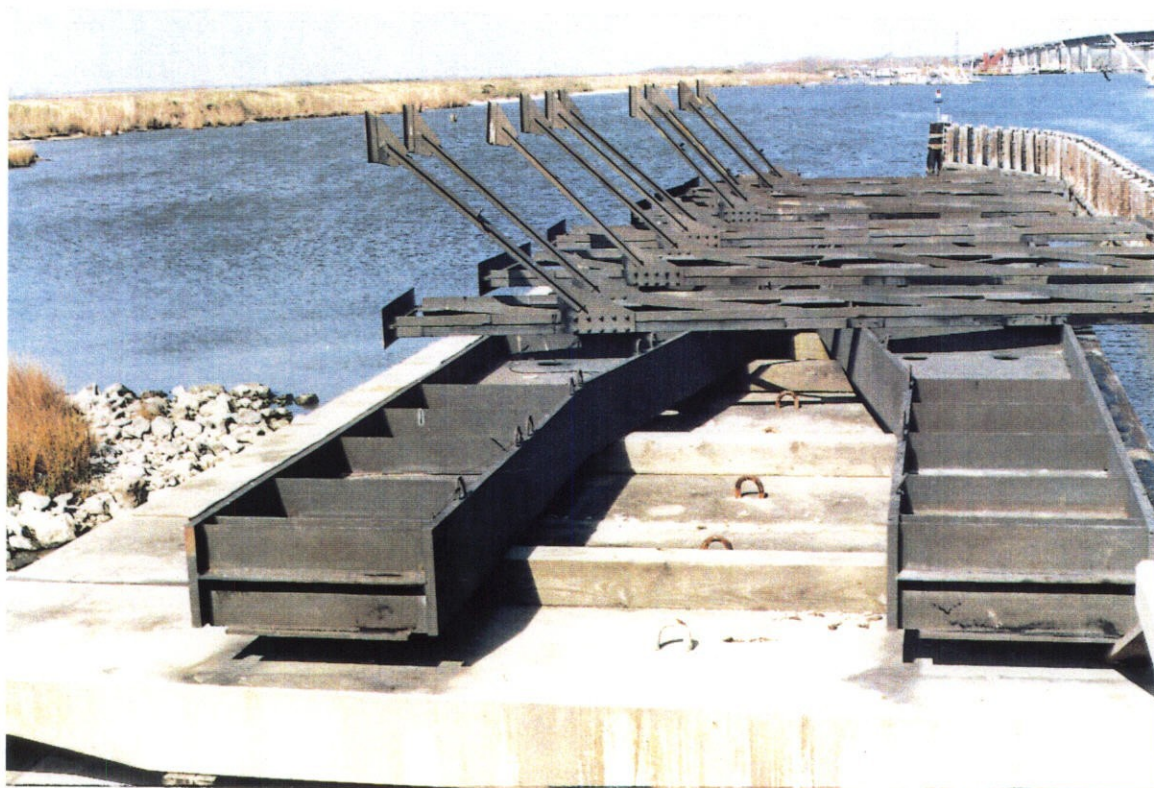
PHOTO NO. 19 - VIEW OF STORED NEEDLES, NEEDLE GIRDERS, AND SUPPORTS. NOTE GOOD CONDITION OF PROTECTIVE COATING SYSTEMS.
