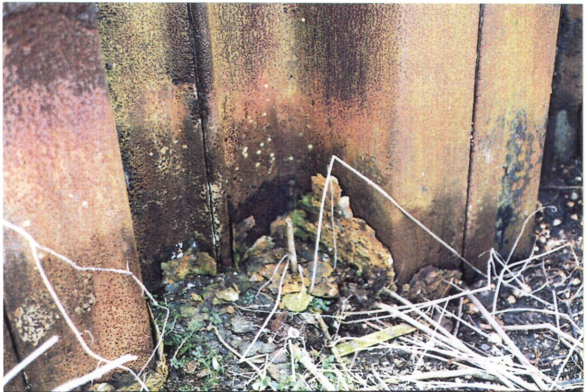
PHOTO NO. 27 - VIEW OF SHEET PILE FLOODWALL SHOWING COMPLETELY DETERIORATED COAL TAR EPOXY.
