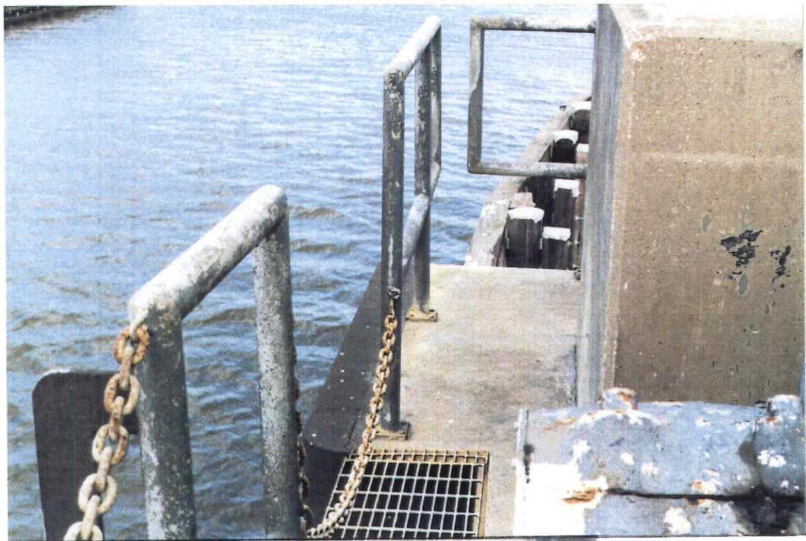
PHOTO NO. 4 - VIEW SHOWING DETERIORATED PAINT ON HANDRAIL AND MISSING EYE FOR CONNECTING THE SAFETY CHAIN.
