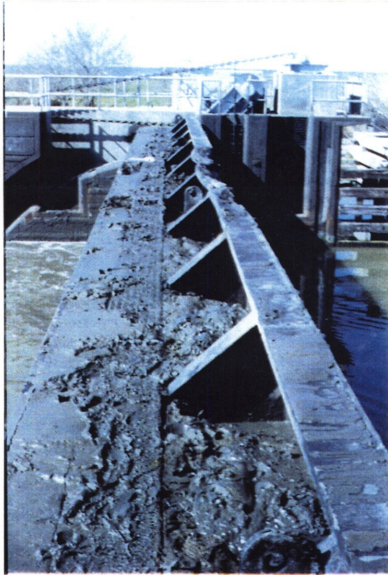
PHOTO NO. 9 - VIEW LOOKING WEST SHOWING DAMAGE TO THE TOP OF THE GATE. NOTE SILT ON TOP OF GATE.
