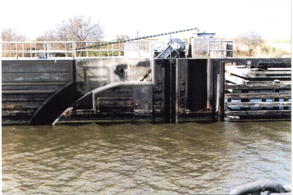
PHOTO NO. 11 - GATE OPERATING MACHINERY ON THE WEST SIDE.
