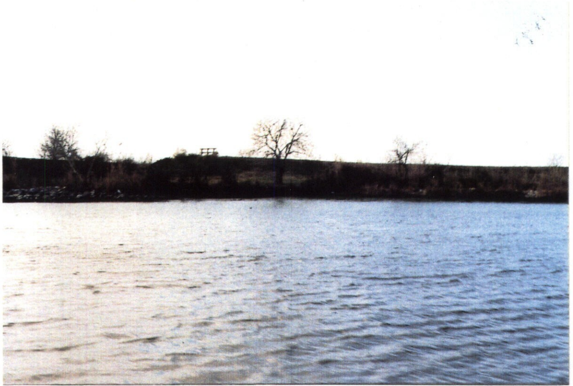
PHOTO NO. 24 - RECEEDING WEST SIDE CHANNEL BANK CAUSED BY EROSION.
