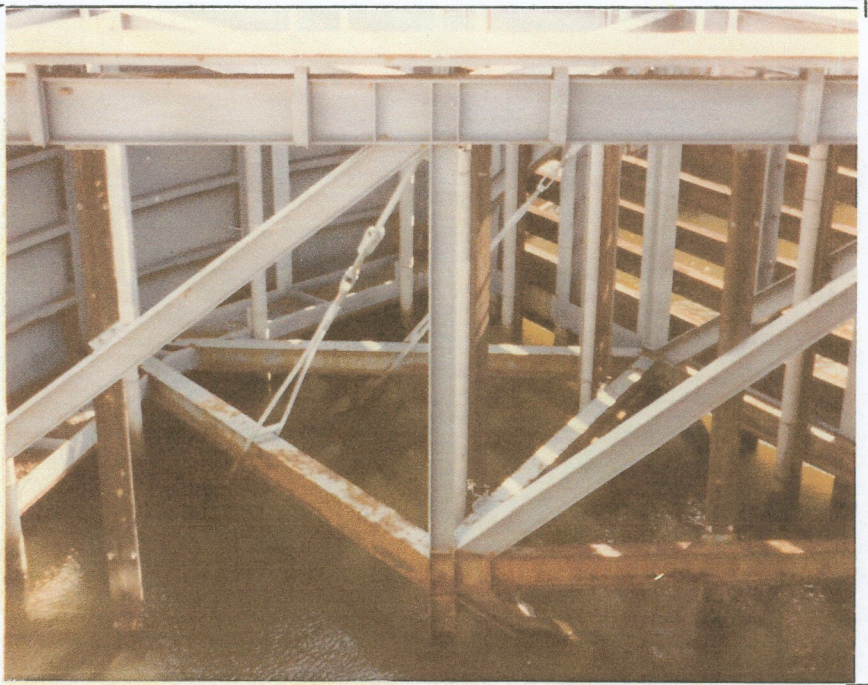
Photo No. 3, Para. 5-03, b(4) - East Sector Gate Corrosion
