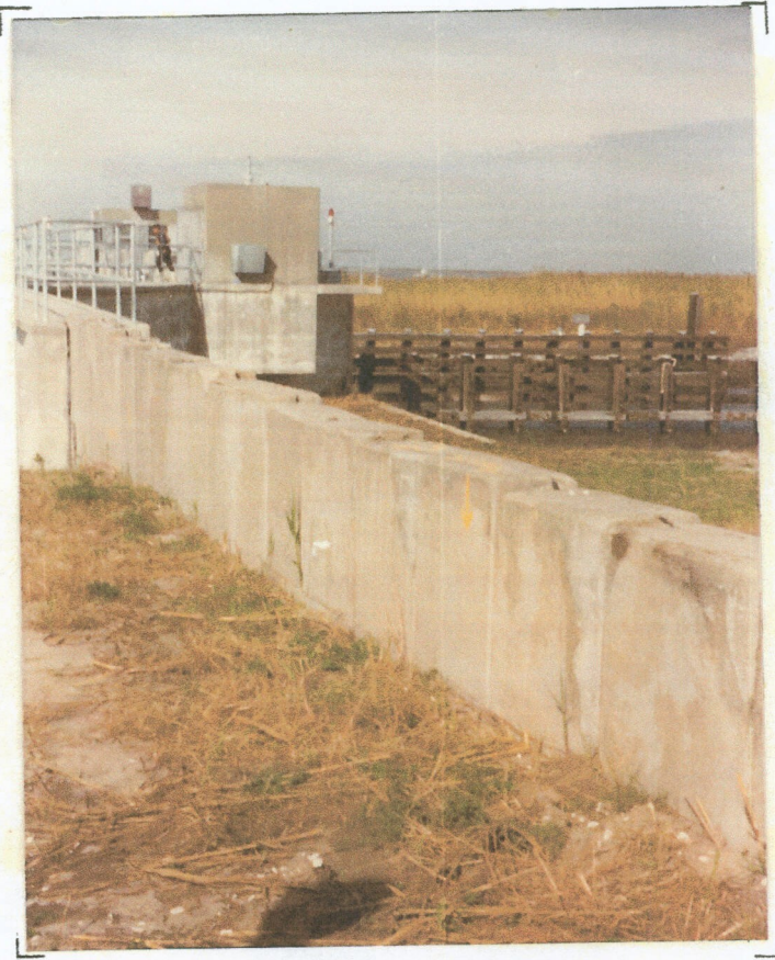
Photo No. 1, Para. 5-03, a(4) - Differential Settlement
