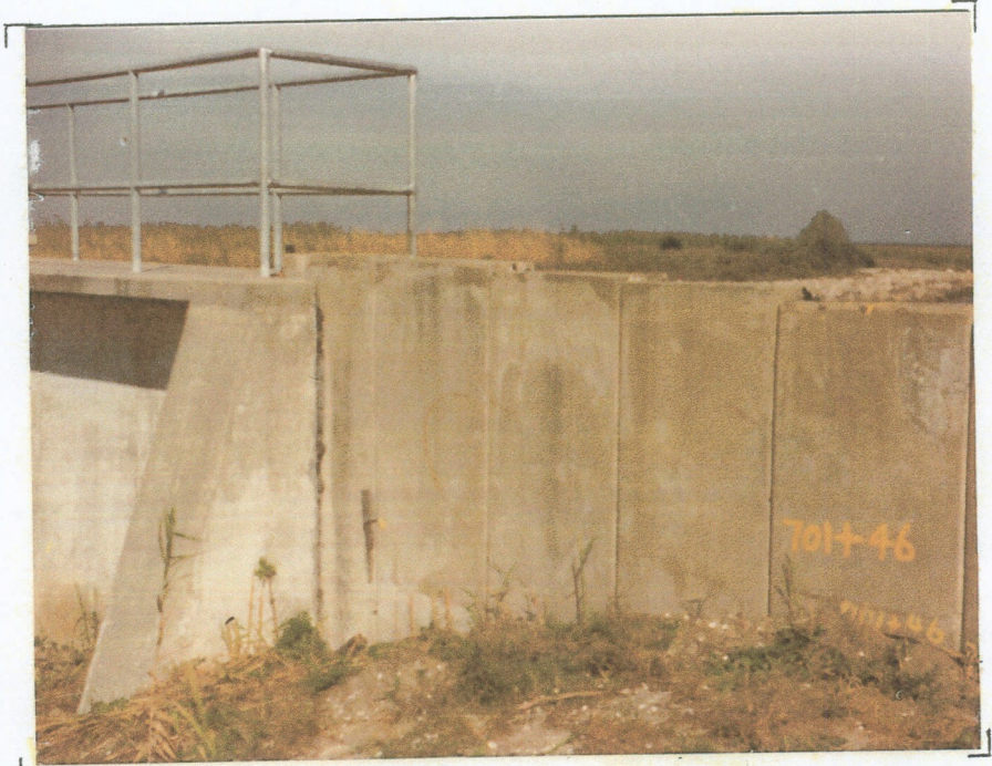
Photo No. 2, Para. 5-03, a(4) - Closeup of Above View
