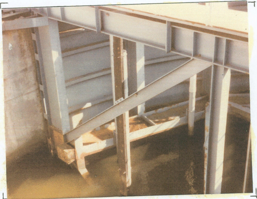
Photo No. 4, Para. 5-03, b(4) - West Sector Gate Corrosion
