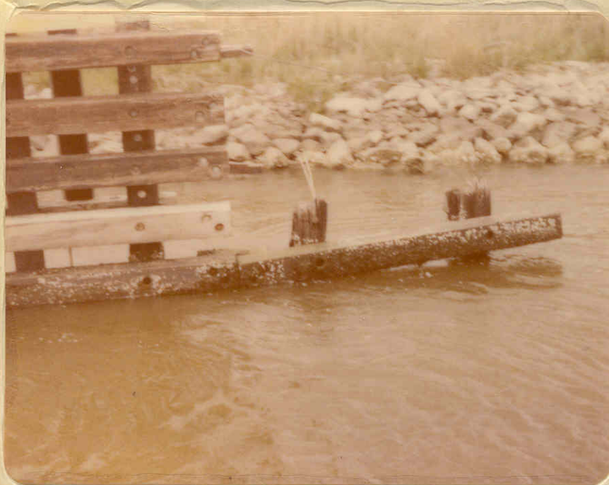
PHOTOGRAPH NO. 2 - Damaged pile bents on the N.W. Guide Wall.
