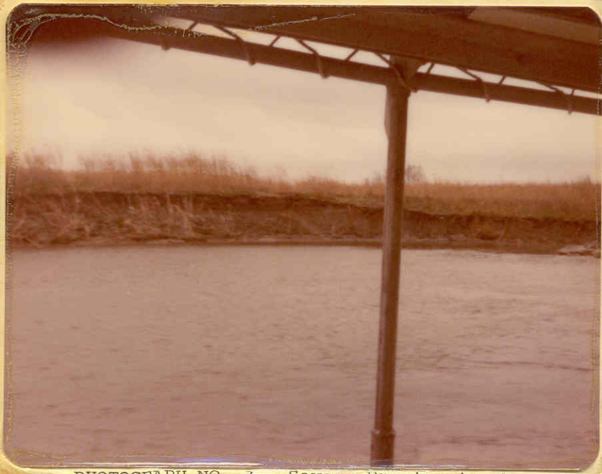
PHOTOGRAPH NO. 3 - Severe Erosion in the west bank on the north approach channel.
