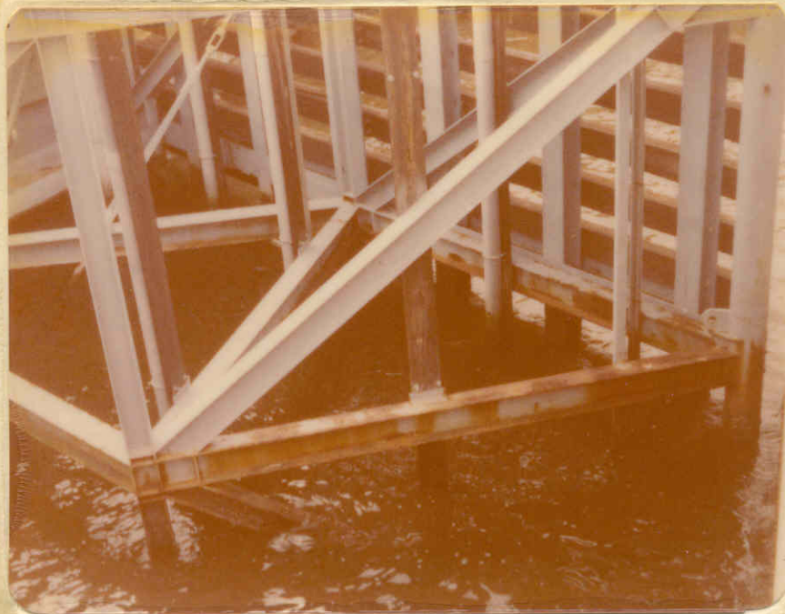
PHOTOGRAPH NO. 1 - Rust Corrosion on Structural Steel Members of Sector Gate.
