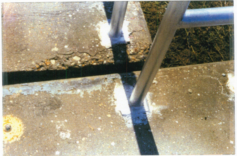
PHOTO 5 - Typical small spalls at the joints on the east side
