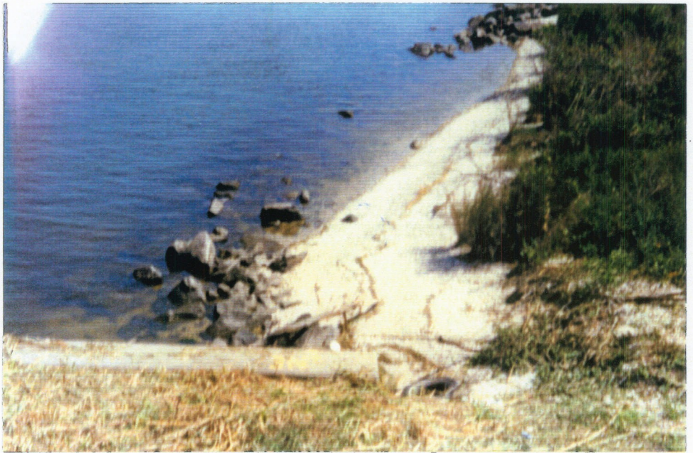
PHOTO 1 - Deficient Rip-Rap along banks of the north and south approach channels (Typical)
