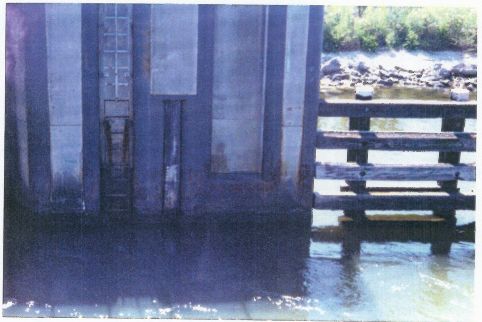
PHOTO 2 - Rusting steel members
