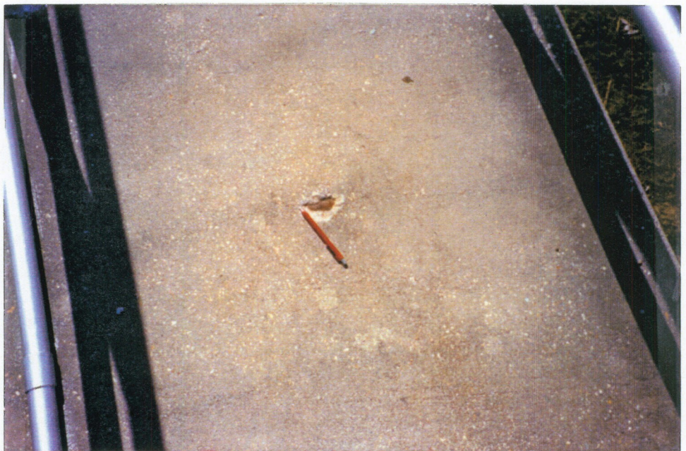
PHOTO 4 - Small spall with exposed rebar on the west side by monolith B-2
