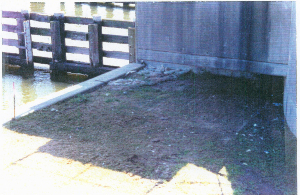
PHOTO 6 - Depression filled with sandbags behind wingwall at northwest corner of structure
