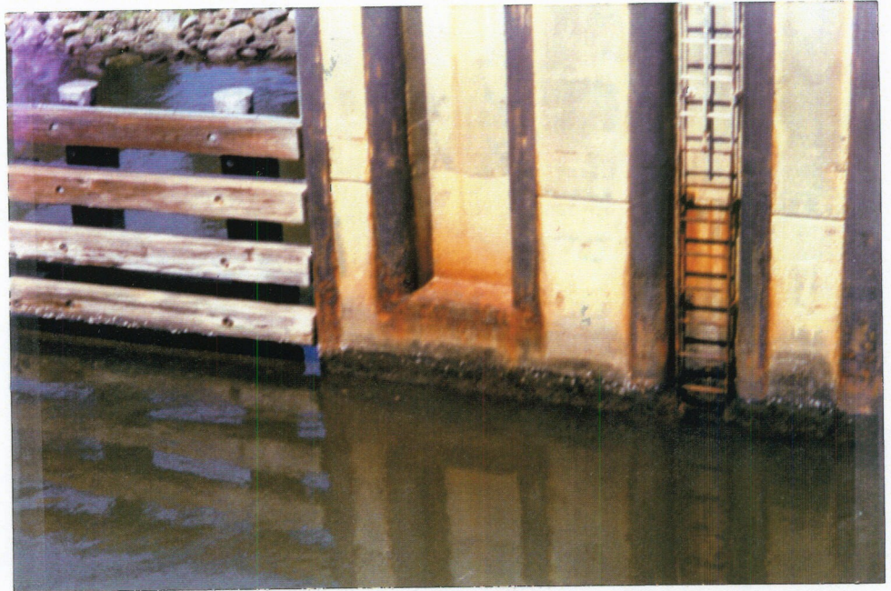
PHOTO 3 - Rusting Steel Members
