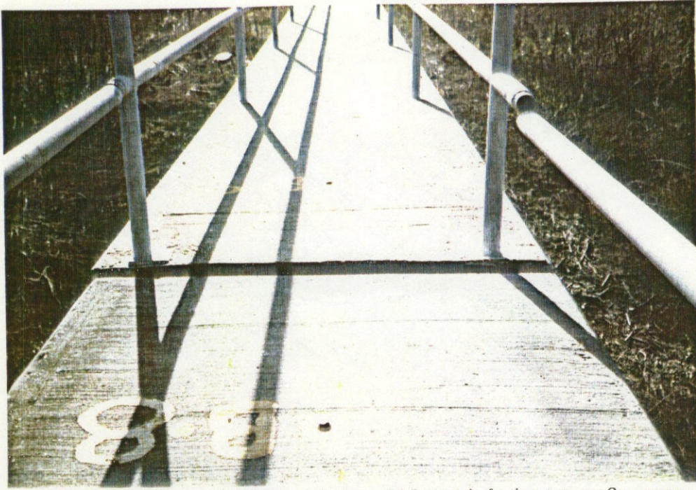
PHOTO 3: Minor differential settlement between reference marks B8 and B9
