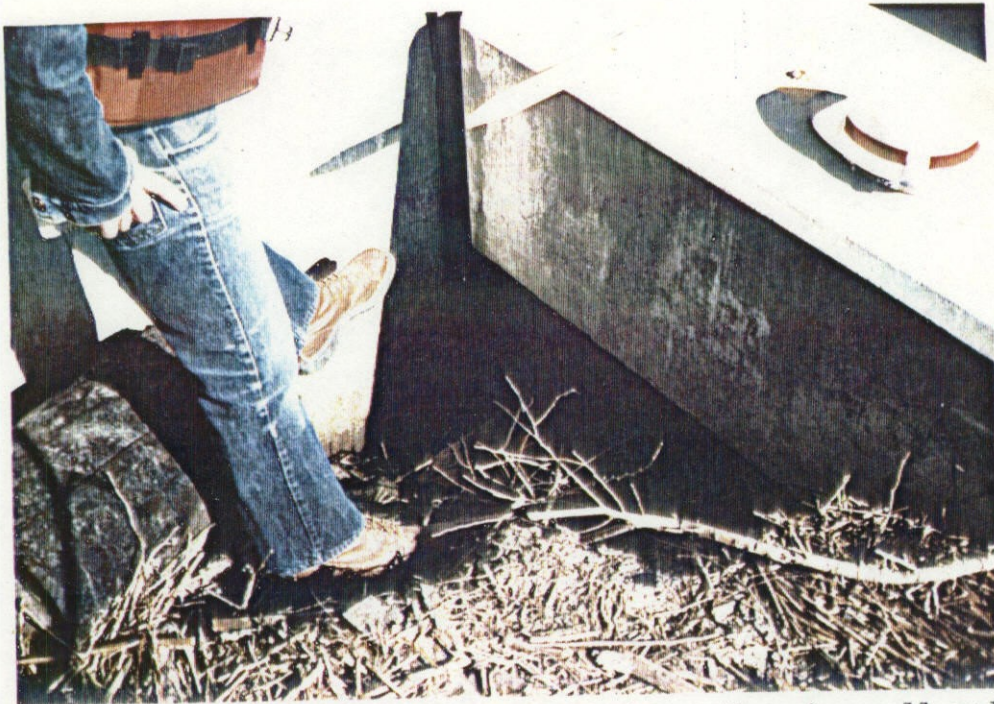
PHOTO 1: Voids behind the joints between the wing wall and main structure (Typical)
