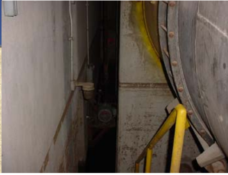
Photo No.2-SELA Equipment Damage
