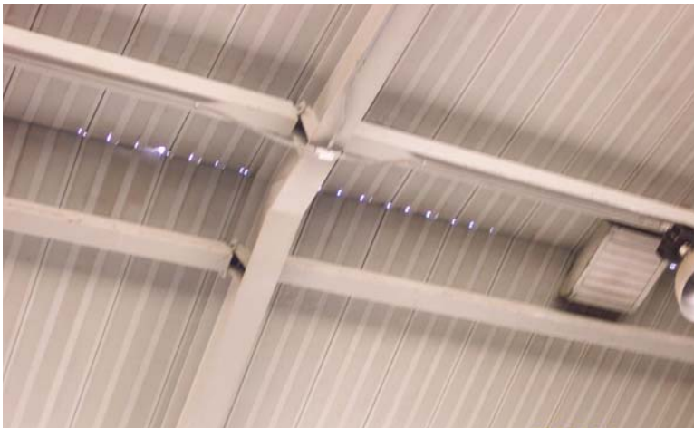
Photo 3 – Ridge cap missing from roof.
