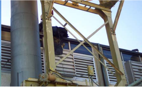
Photo 2 – Roof covering hanging off side of building.
