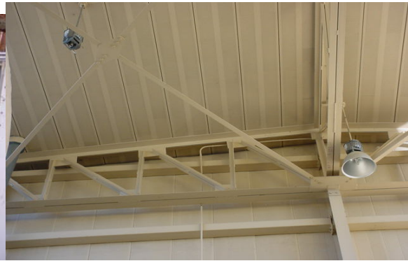
Photo No.4- Damaged overhead lighting
