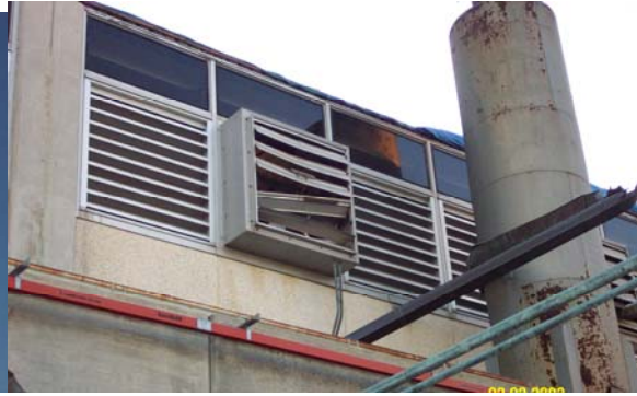
Photo 2 – Damaged exhaust fan louvers.
