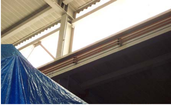
Photo 1 – Vertical wall skylight panels leaking.
