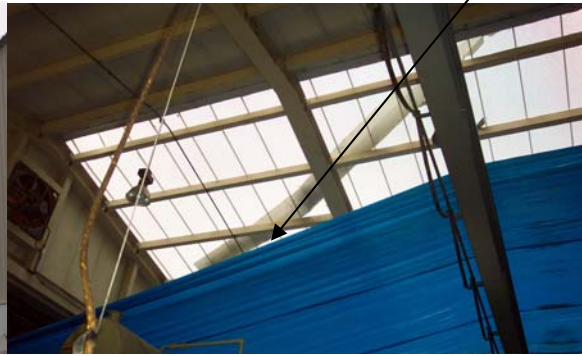
Photo 2 – Inside view of roof damage.
