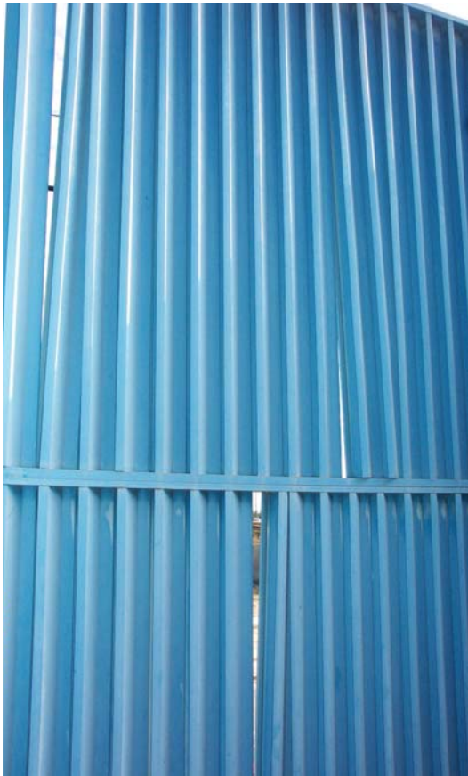
Photo 1 – Louvers in wall missing or damaged.
