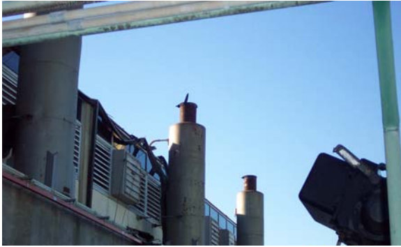
Photo 1 – Steel exhaust cover damaged; gutter damaged.
