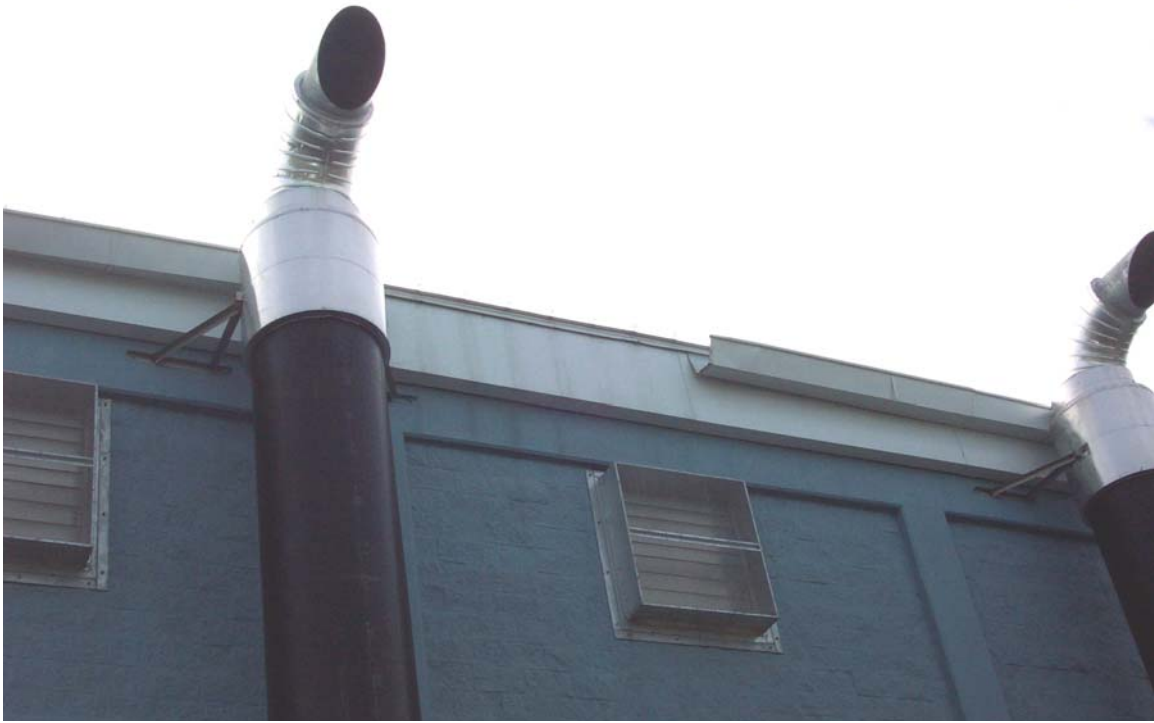
Photo 1 – Portion of gutter missing.
