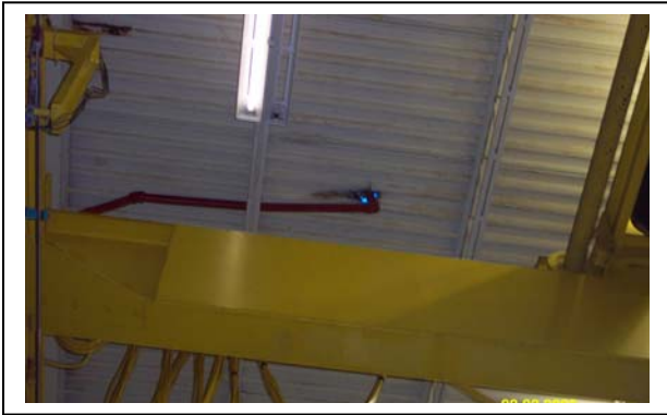
P Photo 3 – Bent vent pipe for fuel day tank
