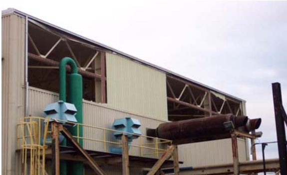
Photo 1 – Vertical corrugated skylight panes missing.
