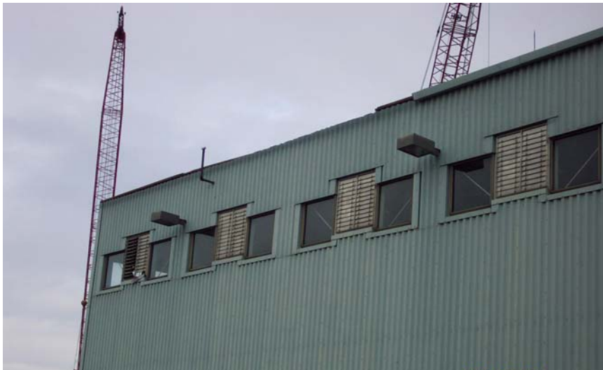
Photo 2 - Damaged lightning protection system and portion of gutter missing.
