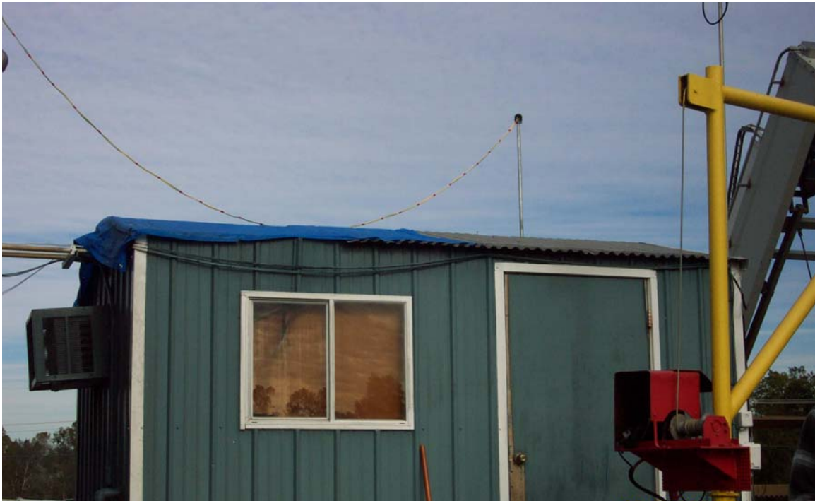
Photo 1 – Half of corrugated metal roof missing on office building.
