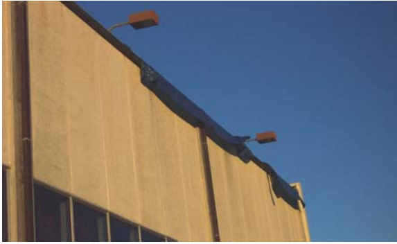
Photo 1 – Roof covering displaced.
