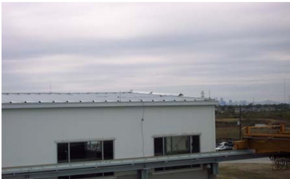
Photo No.4- Damaged lightning protection conductors .
