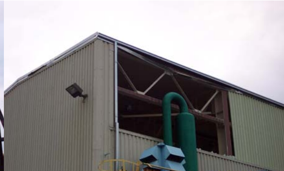
Photo 2 – Flashing missing or damaged.
