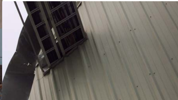
Photo No.4, Damaged aluminum cable tray cover
