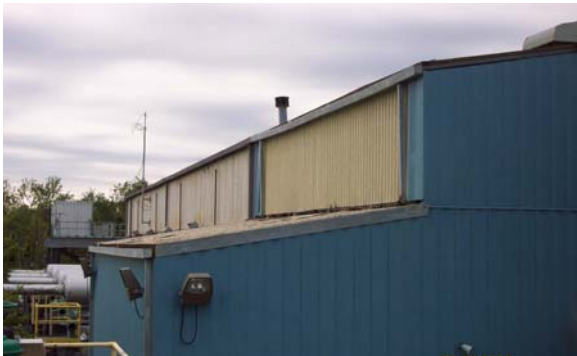
Photo 2 – Flashing missing from vertical wall skylight panels.
