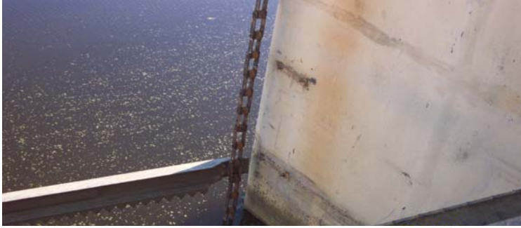
Photo 1—Missing guide for trash rack.
