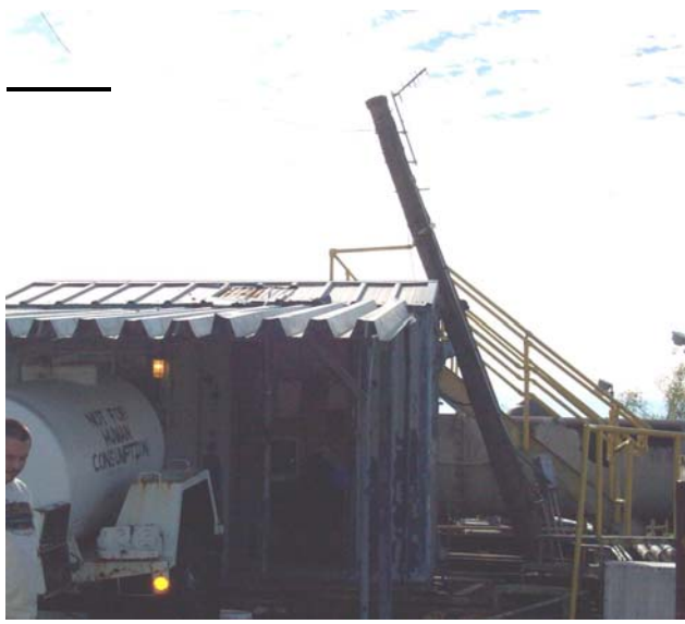
Photo 1 – Damage to roof of office and pole resting on office.
