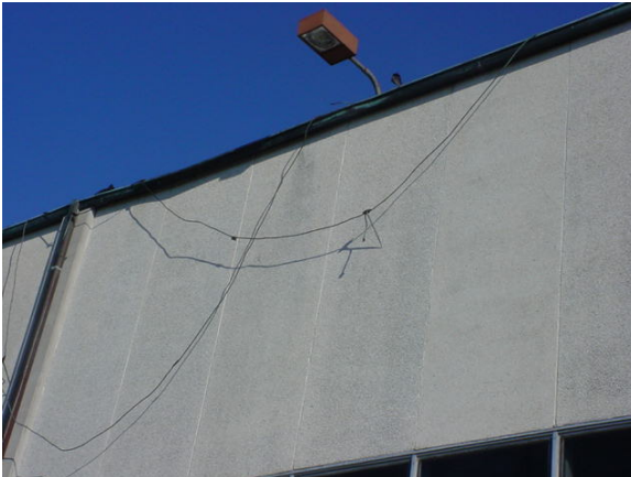
Photo No. 5- Damaged Lightning Protection System
