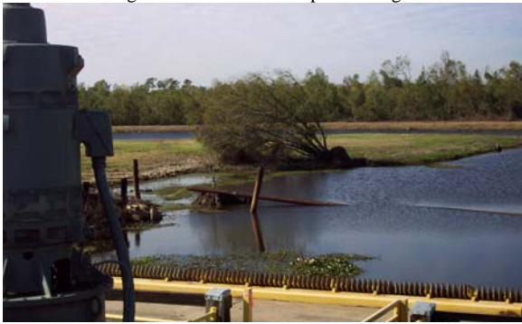
Photo 2 – Horizontal timber in timber trash rack needs re-alignment.
