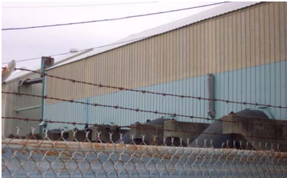
Photo 3 – Exhaust stacks missing
