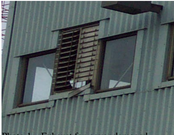
Photo 1 – Exhaust fan cover damaged.
