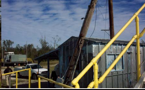
Photo No. 4- Damaged electrical service pole
