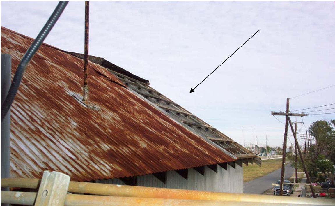
Photo 1 – Portion of corrugated metal roof missing.
