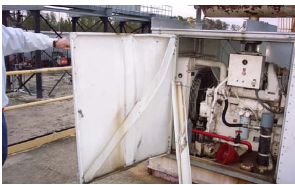
Photo No.3- Damaged GenSet enclosure
