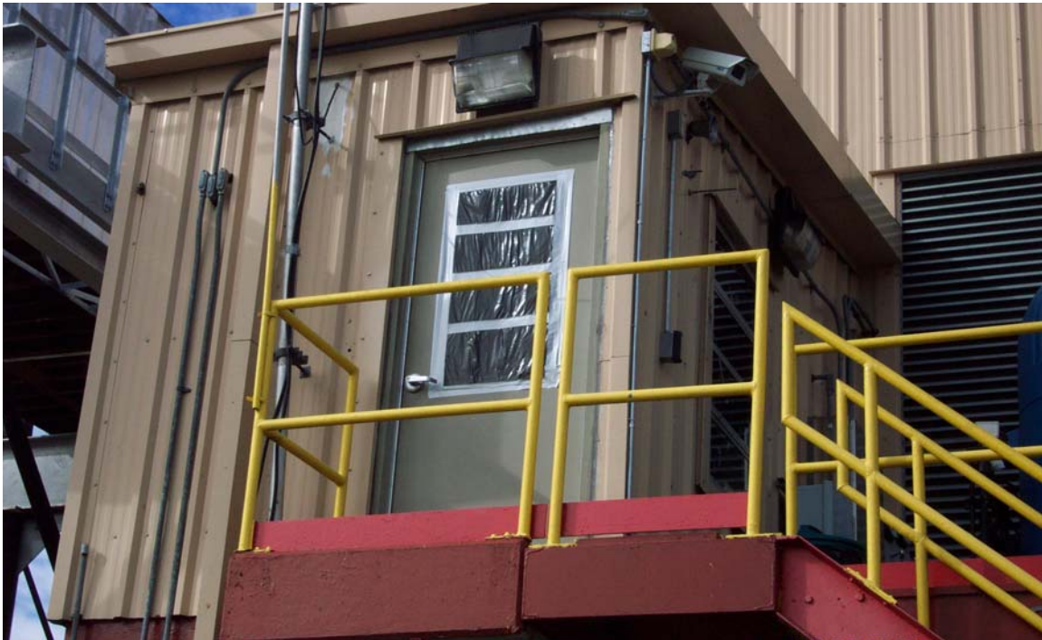
Photo 1 – Glass broken in door.
