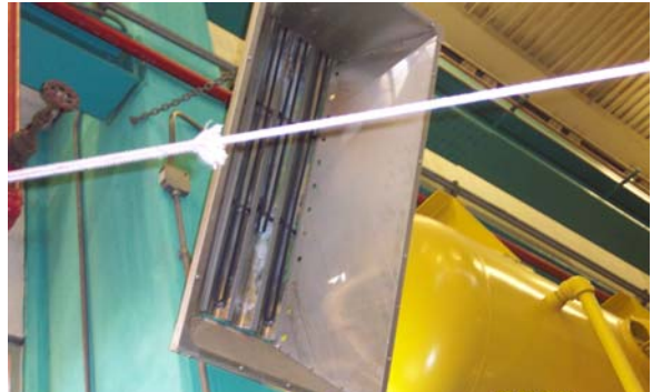
No. 4- Damaged Heater Elements
