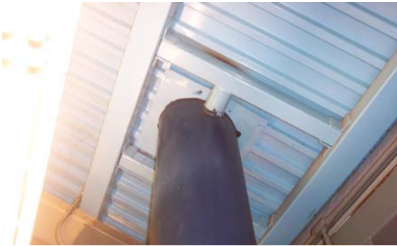
Photo 2 – Leak in roof at vent stack.
