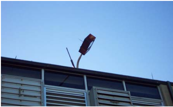
Photo No.3- Damaged light and lightning protection
