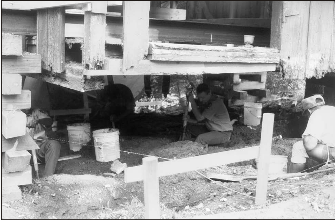
Figure 9. Excavation of the area under the Chicken House (HS-5) took place in 1998.
