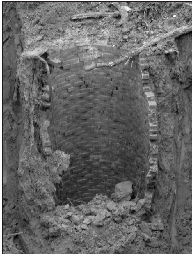
Figure 14. The shaft and the lining of the Barn Well in profile after the collapse of the west wall. Vertical scale is approximately 14 feet from ground surface to the base of the well; view is to the east.
