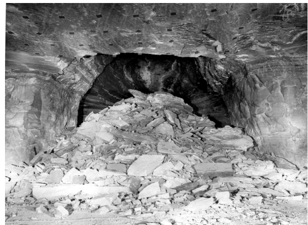
Figure 3. Massive roof fall measuring 45 ft wide by 20 to 30 ft high and extending for approximately 200 hundred feet.
