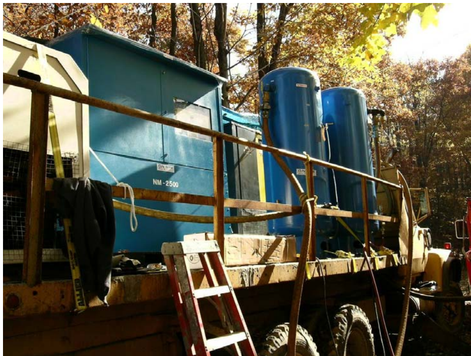
Figure 3. Nitrogen membrane separation plant.
