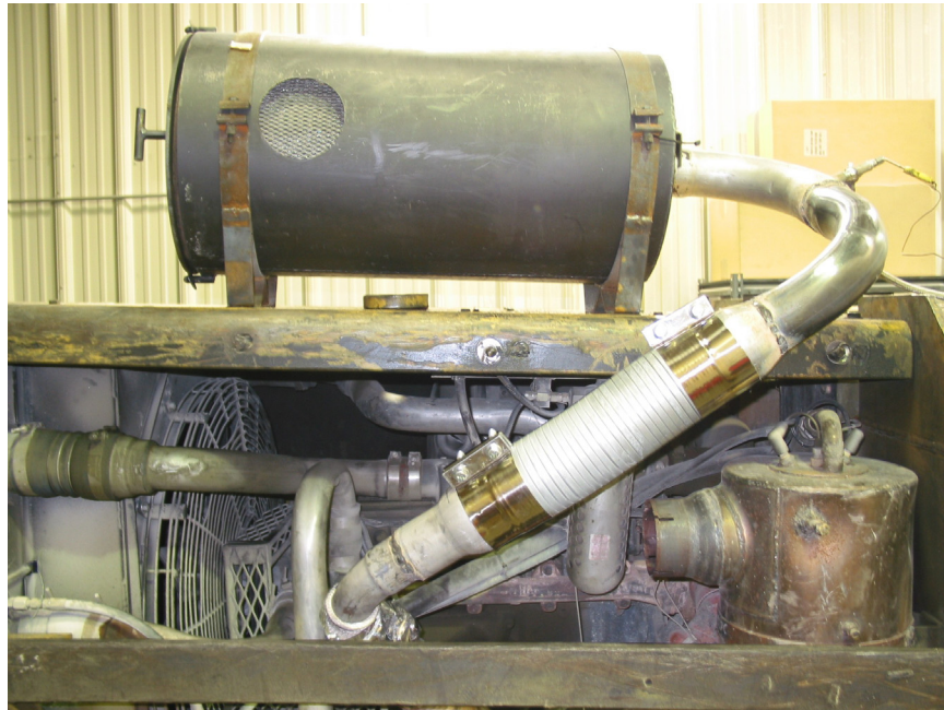
Figure 3.—Filtration system used in testing high-temperature disposable elements from Donaldson and Filter Service.
