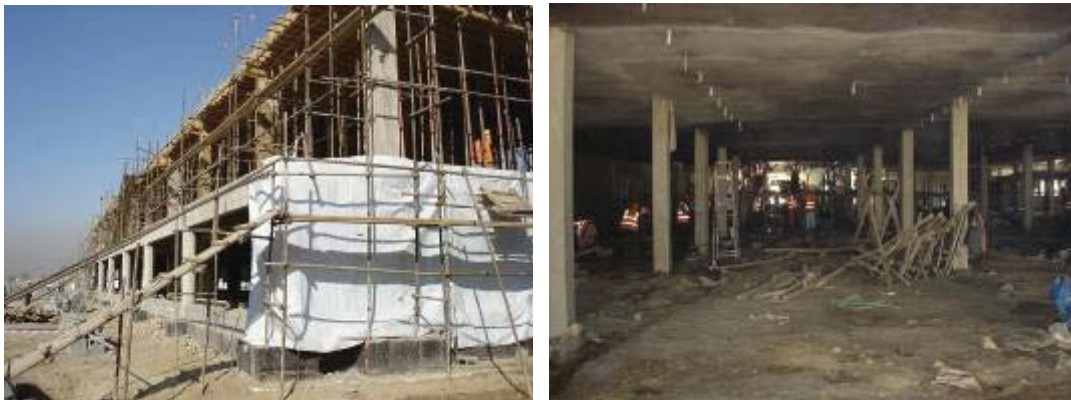
Figure 2. Classrooms (left) and Dining Facility (right) under construction at Kabul Military Training Center
