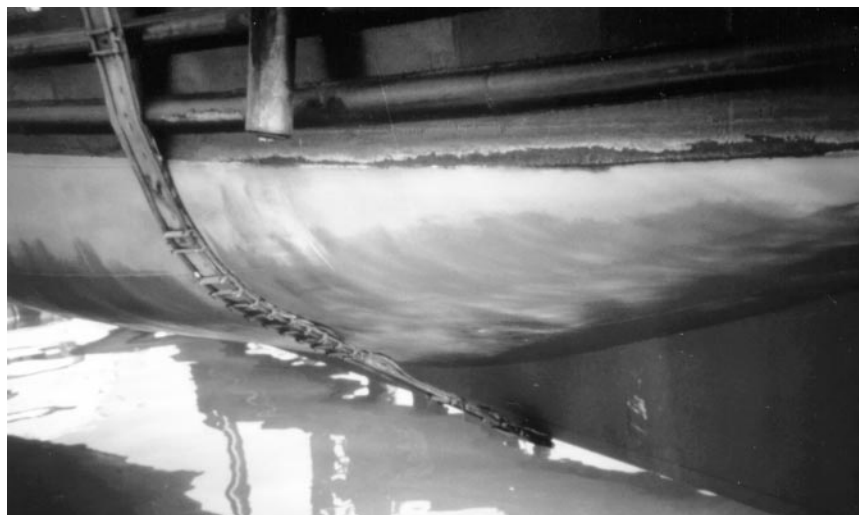
Figure 2. Close up of the copper containing epoxy material
