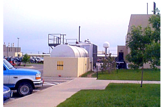
Service equipment needs additional screening.
