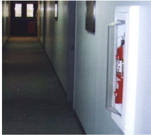
Recessed fire extinguisher cabinet finished to match wall.
