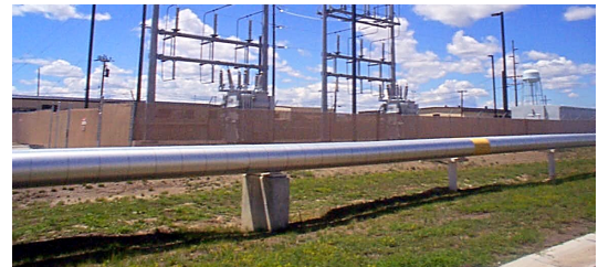
Existing unscreened above-ground utility lines.
