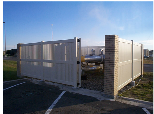
Utility equipment enclosure.
