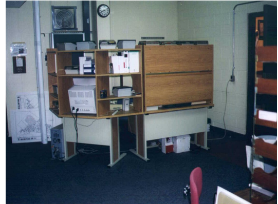
Exposed wires are unsightly and present a hazard.
