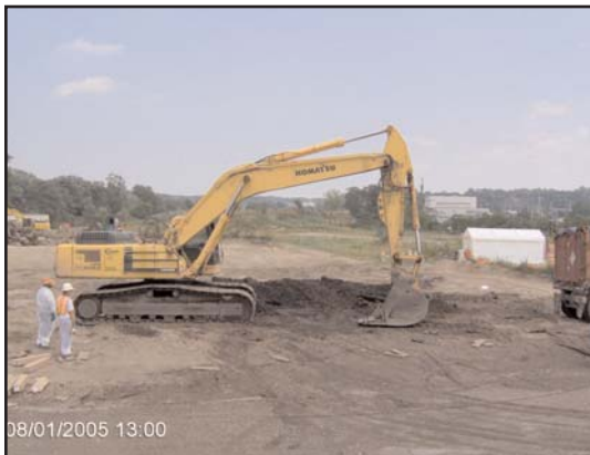
Contractors supervise an excavator loading radioactive soil for off site removal and disposal. Photo credit: Richard Dabal, USACE.
