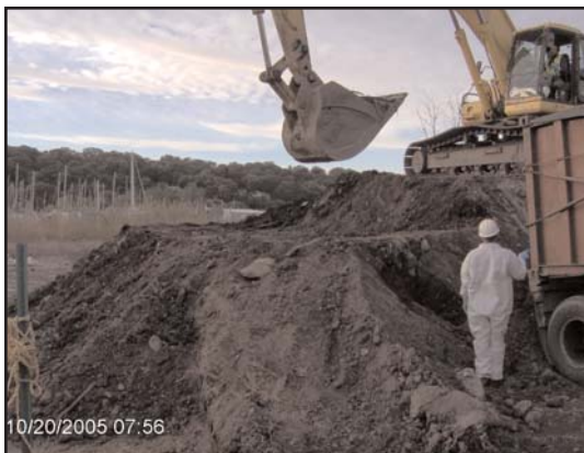
Contractor using excavator to load low level radioactive soil. Photo credit: Richard Dabal, USACE.
