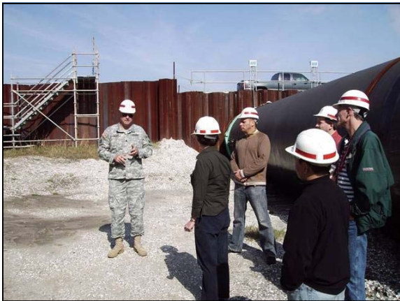
Planning Associates with LTC Zillmer of the Hurricane Protection Office at a construction site in New Orleans
