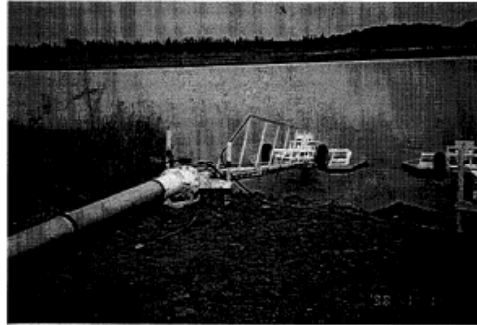
Example of an Electric Pump
