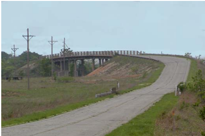
The Galena viaduct is an important feature of the Kansas Route 66 cultural landscape and traveling experience. The bridge is in need of critical repairs to retain its historic character and keep it safe for transportation.
