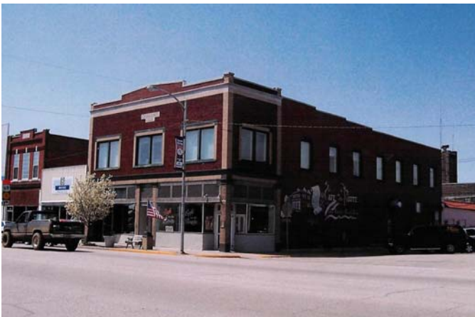
The Café on the Route is a 19 th century Main Street building that has served as a diner on Route 66 since the 1950s. Structural problems will be addressed through the preparation of Preservation Plan.
