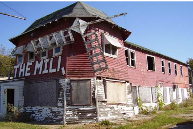
The Route 66 Heritage Foundation of Lincoln County purchased the Mill to save it from demolition. The Mill was placed on Illinois' "Ten Most Endangered Places" list by Landmarks Illinois in 2008.
