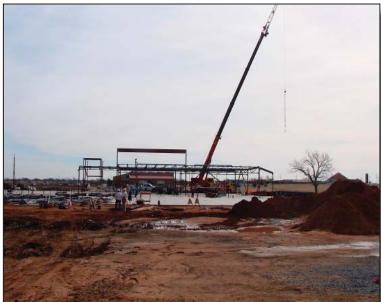
Photo courtesy of Tulsa District New Air Defense Artillery School dining facility under construction at Fort Sill.
