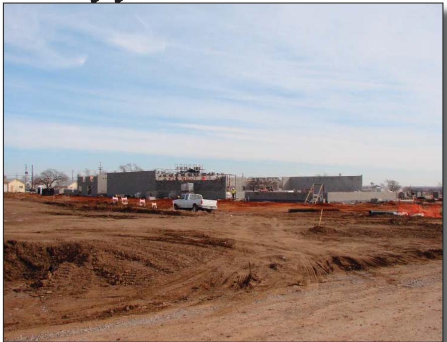
Photo courtesy of Tulsa District Air Defense Artillery School Instructional building being constructed at Fort Sill.
