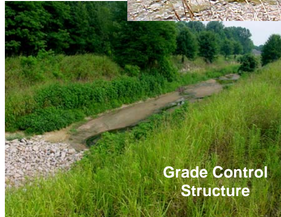
Lateral D Failure at Sewer Siphon Protection
