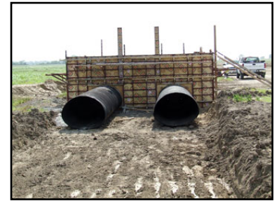
Pipes and concrete forms for one of the sediment containment outlet structures
