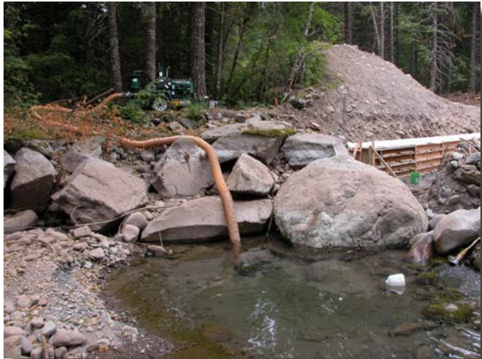
Figure 8.6—Lower sump collects water bypassing the construction. The hose on the right is discharge from the upper sump. The water is pumped from the sump to a treatment area where the water is dispersed in the vegetation.
