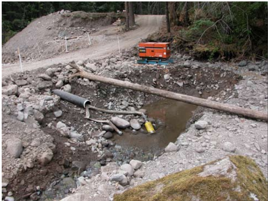
Figure 8.5—Upper sump collects water that bypasses or seeps through the diversion dam.
