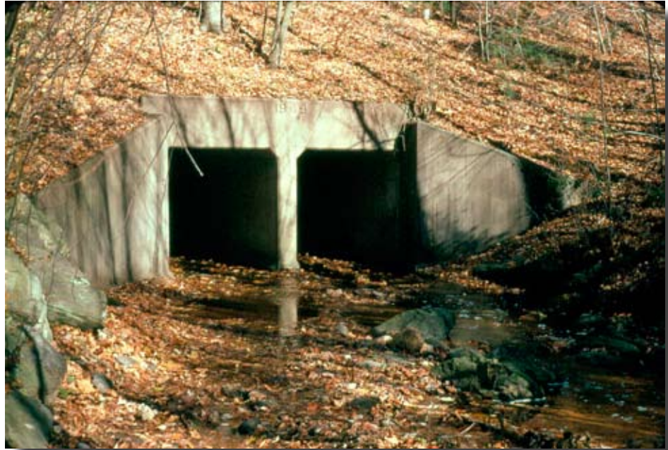
Figure 1.23—Lack of a low-flow channel results in insufficient water depth in these box culverts. Photo: Scott Jackson, University of Massachusetts.
