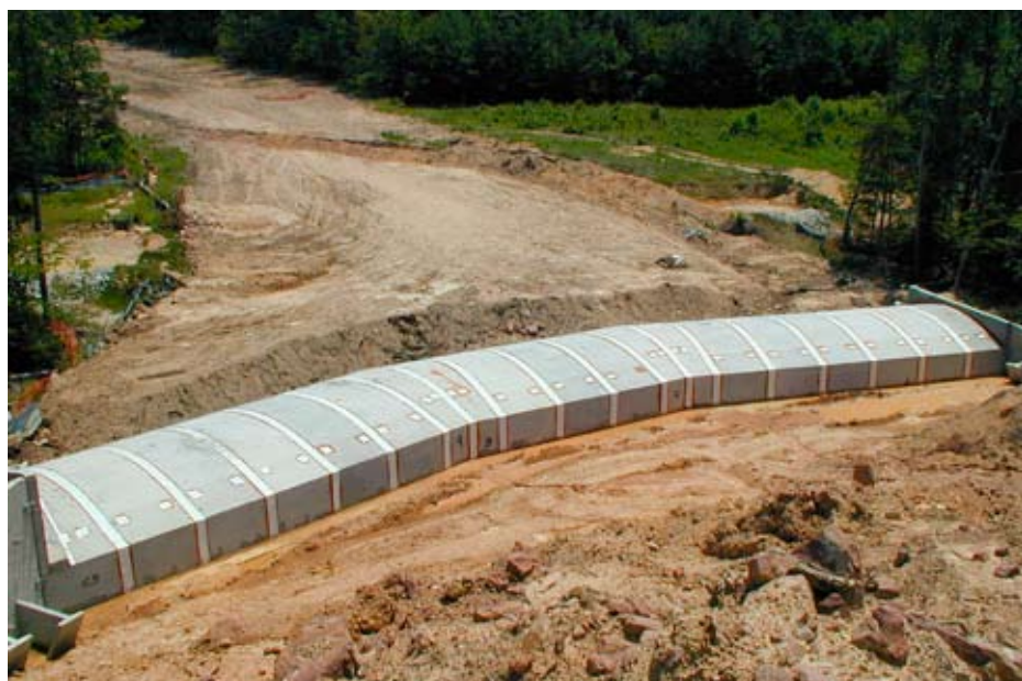
Figure 6.5—Curved concrete pipe installation at Arrington Development, Durham, North Carolina, June 2001. (Pipe is 142 feet long, with a 24-foot span and a 7-foot rise.) Courtesy of CON/SPAN Bridge Systems.
