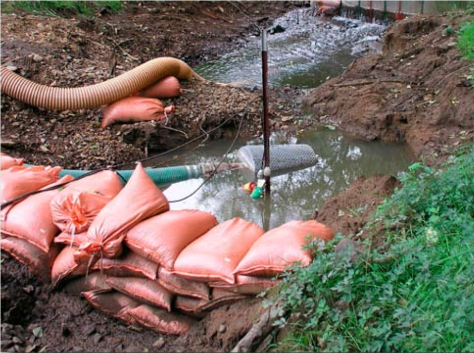
Figure 8.7—Pump controls: float switches are attached to stake in sump.
