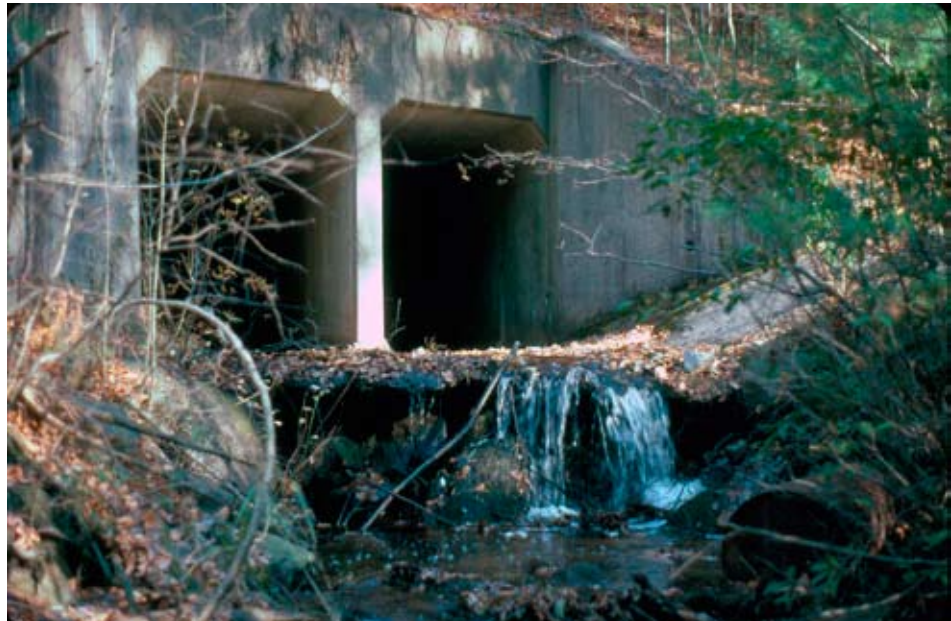
Figure 1.21—Outlet drop formed by scour at the downstream end of an asphalt apron. Photo: Scott Jackson, University of Massachusetts.
