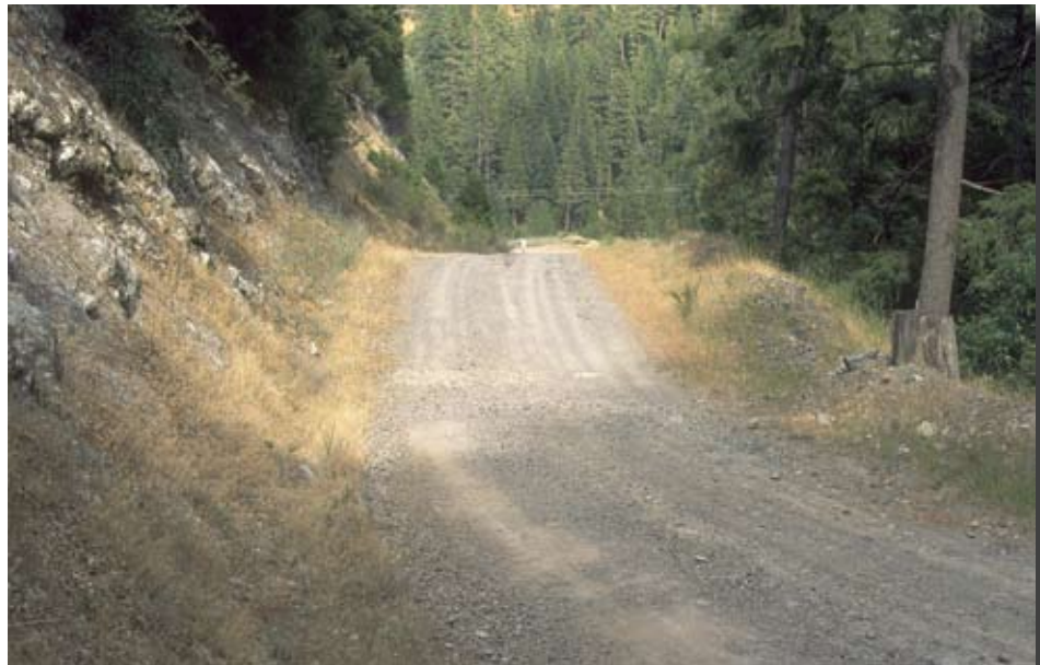
Figure 7.20—Diversion-prevention dip on the Plumas National Forest, California. The diversion dip is located just down the road from the stream crossing because the crossing is on a tight curve.
