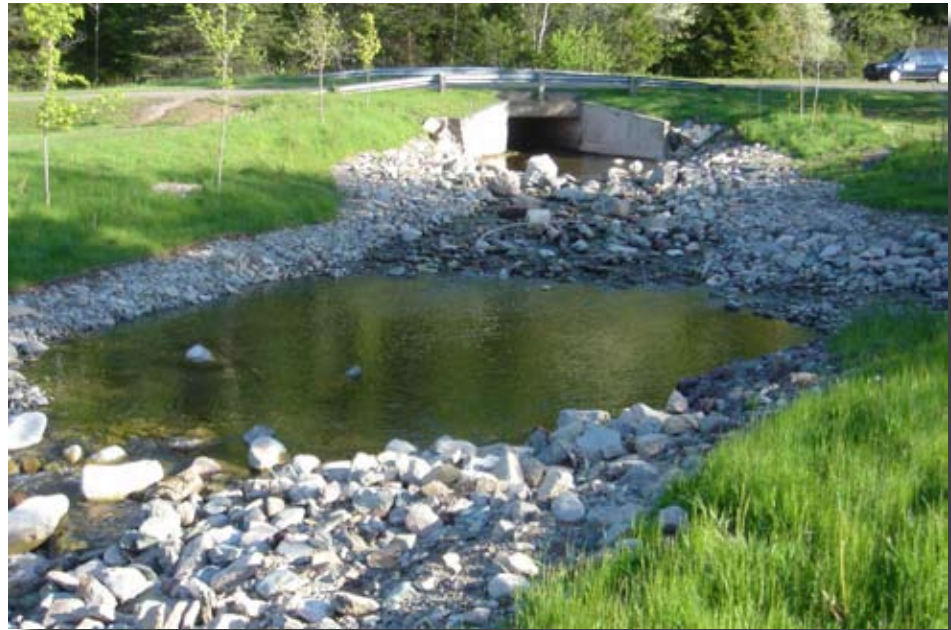
Figure F.3—Rock riffle used to backwater the outlet of a box culvert on Dickson Brook, Bay of Fundy, New Brunswick, Canada. Photo courtesy of Dr. Robert Newbury, Newbury Hydraulics, Okanagan Centre, British Columbia, Canada.
