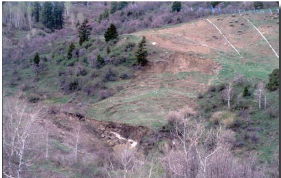
Figure A.27—Stream eroding the toe of a slump is likely to transport large volumes of sediment that may plug downstream culverts.
