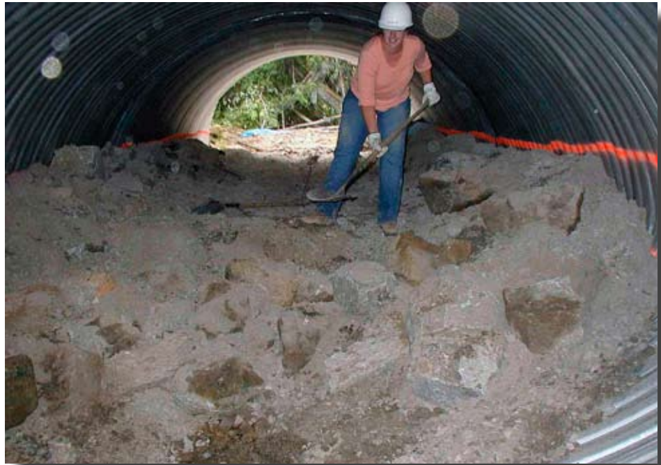
Figure 8.16—Assuring proper cross-section shape, rock-band spacing and placement of channel rocks and footers often require hand work.
