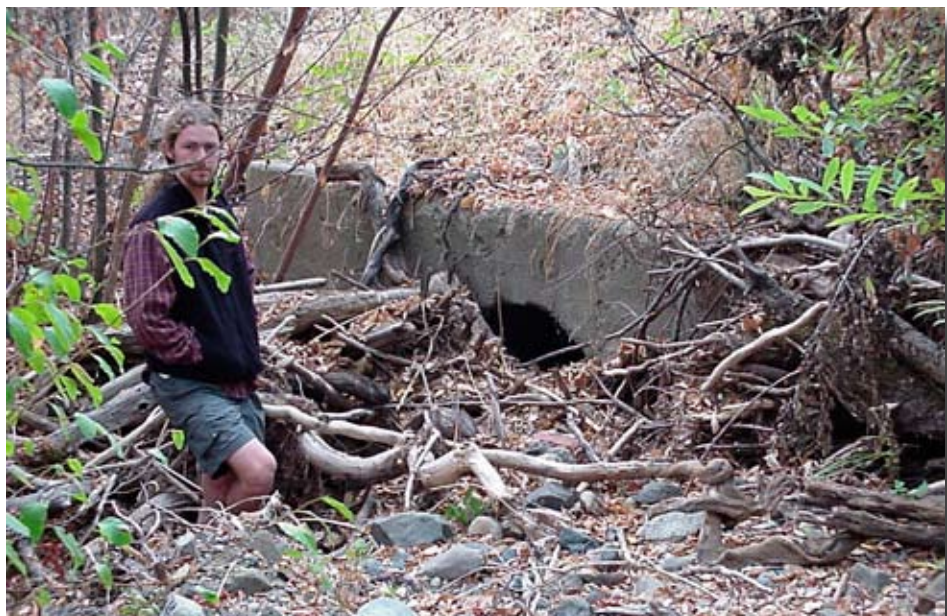
Figure 1.16—Debris and sediment at culvert inlet can be a fish barrier. Photo courtesy of Ross Taylor and Associates, McKinleyville, California.
