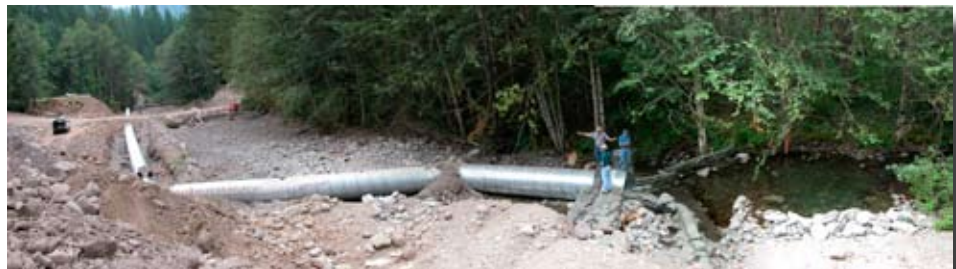
Figure 8.4. Diversion dam and gravity pipe bypass system. Bypass road is visible in the background, and excavation in main road is just beyond it.
