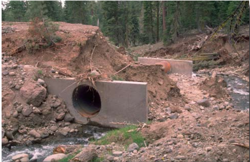
Figure 1.18—Culvert-crossing failure after flooding, Plumas National Forest, California.
