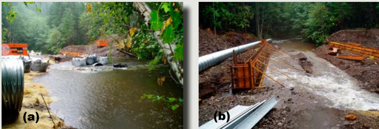
Figure 8.9—Unusual summer storm overwhelms bypass system. (a) Looking downstream at bypass pipe, now in mid-channel. (b) Looking downstream through the open excavation.
