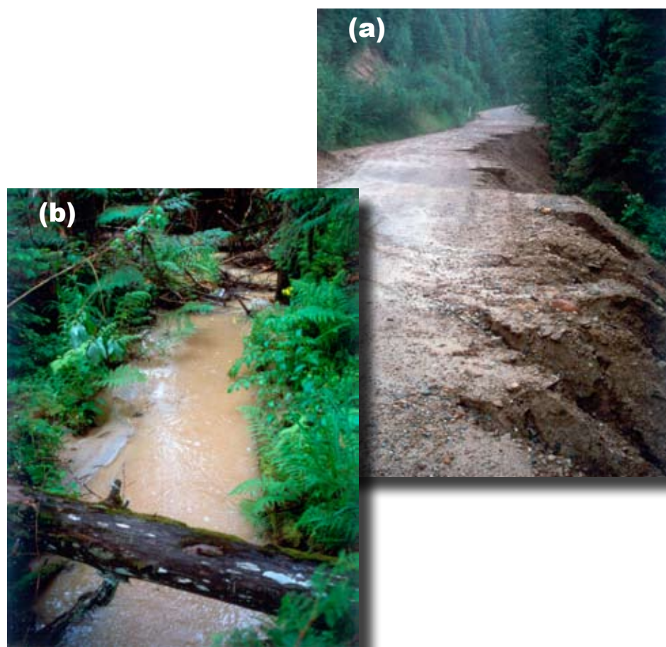
Figure 4.2—Flood-damage surveys can provide historical context for stream condition. (a) On Gap Creek in northeastern Washington, extensive erosion occurred on a riparian road in unconsolidated glacial sands during a 1993 flood. (b) Sediment filled the channel for several years but this transport channel remained stable and the sediment progressively cleared out during subsequent high flows.
