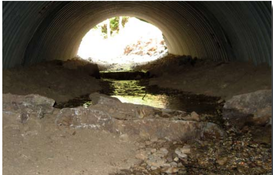
Figure 8.12—Newly constructed (2007) step-pool channel inside culvert on Eustache Creek, Lolo National Forest, Idaho. Two visible rock weirs (steps) have their lowest points offset to provide some sinuosity at low flow. The top of the sloped banks is bankfull elevation.
