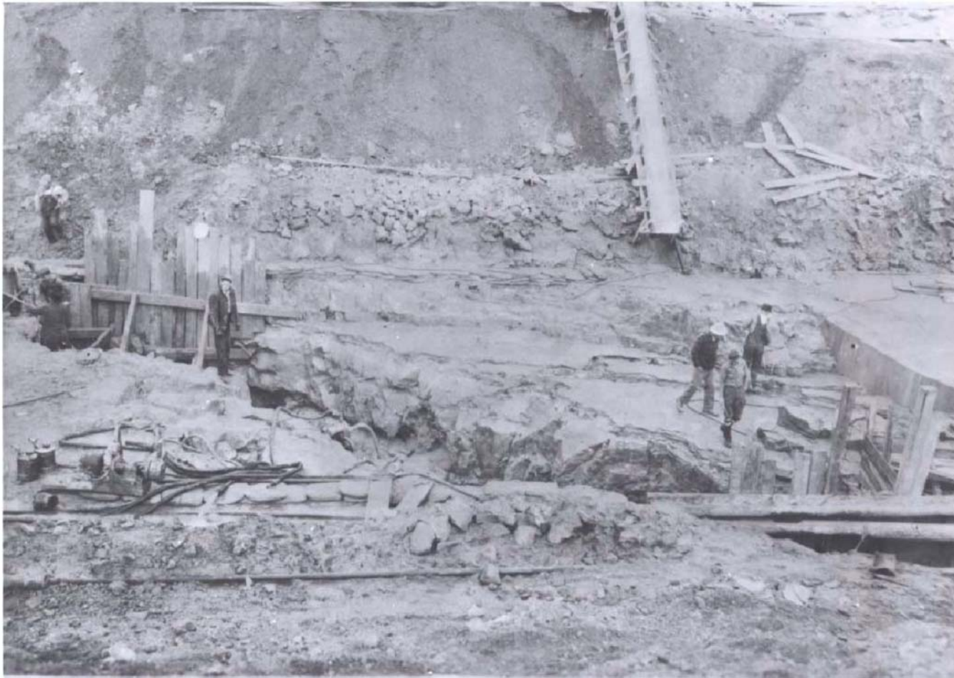
Looking NW from 35' U.S. of station 40 / 15: Open joint in cut-off trench foundation.
