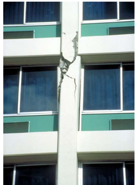
Figure 2. Damage to older, reinforced concrete building in the 1994 Northridge Earthquake. © 1994 by Peter W. Clark and Regents of the University of California.
