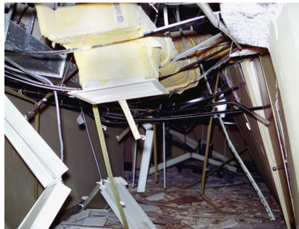
Figure 11. Nonstructural damage (fallen ceiling, partitions, piping, and ducts) to the basement of the Olive View Medical Treatment Building caused by the 1971 San Fernando earthquake in California. © 1971 by Earthquake Engineering Research Center and Regents of the University of California.
