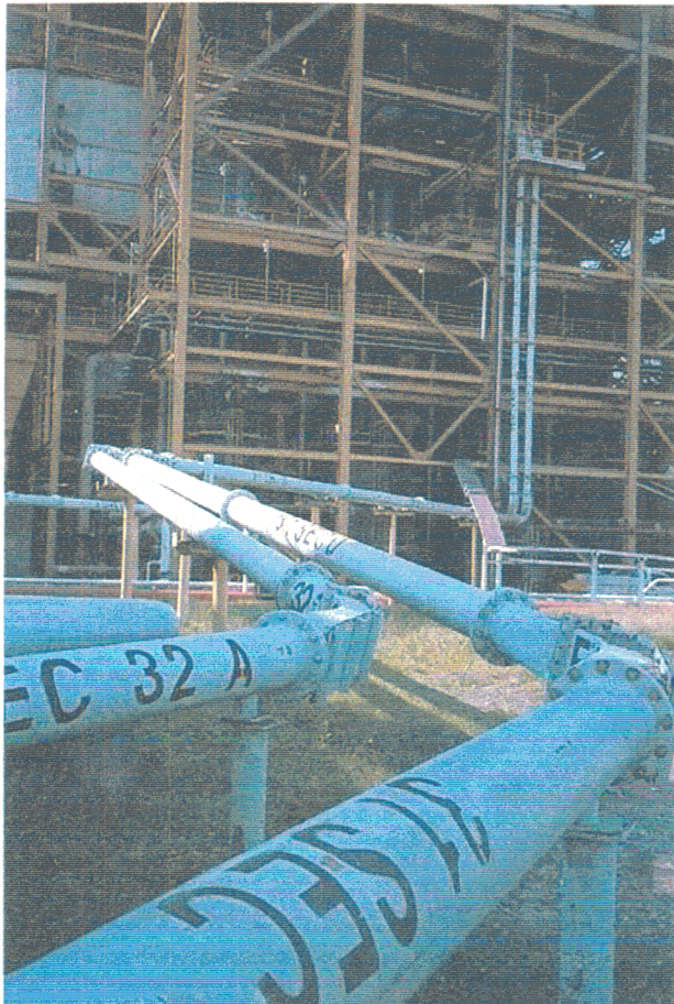
PHOTO 11 Fuel Transport Pipes
