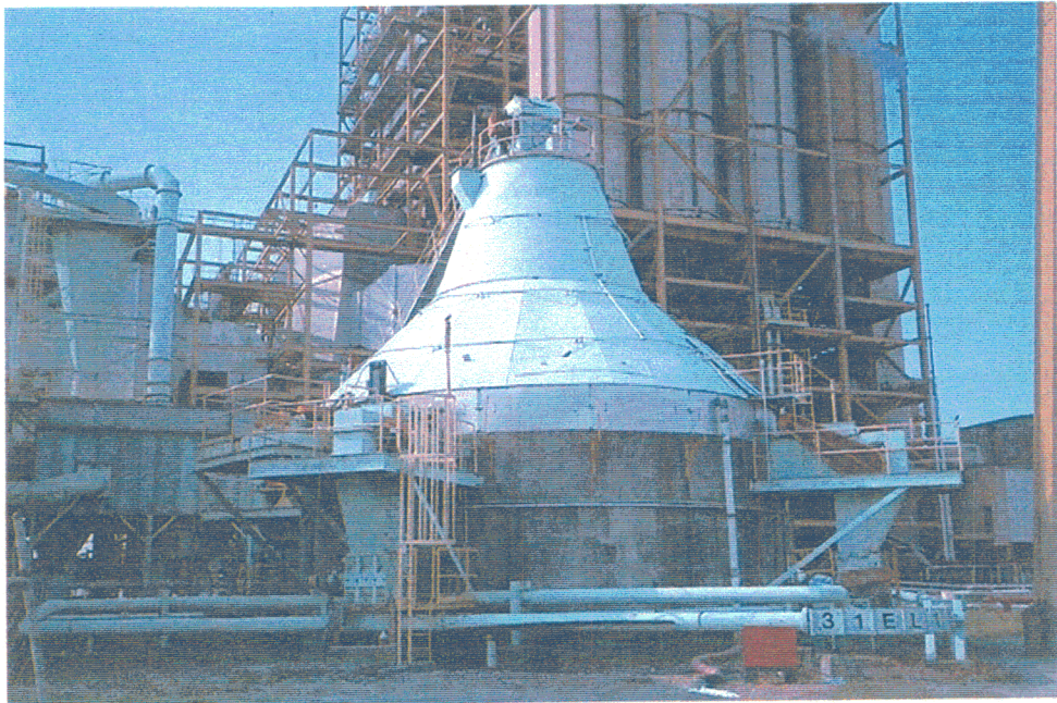
PHOTO 4 Atlas Storage Bin with Drag Chain Discharge Conveyors and Pneumatic Transport Lines
