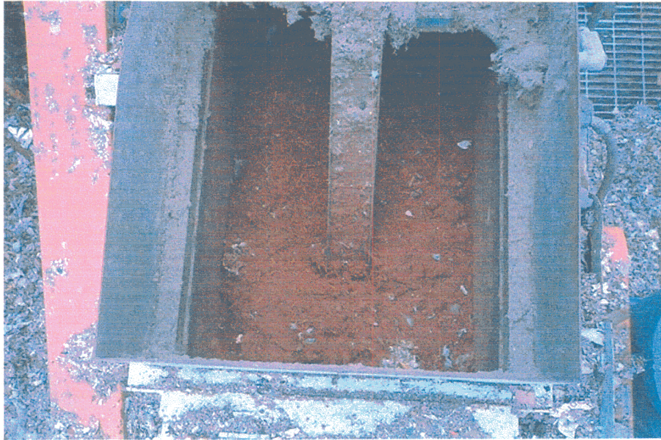
PHOTO 9 Top View of Drag Chain Discharge While Conveying Eucalyptus Chips
