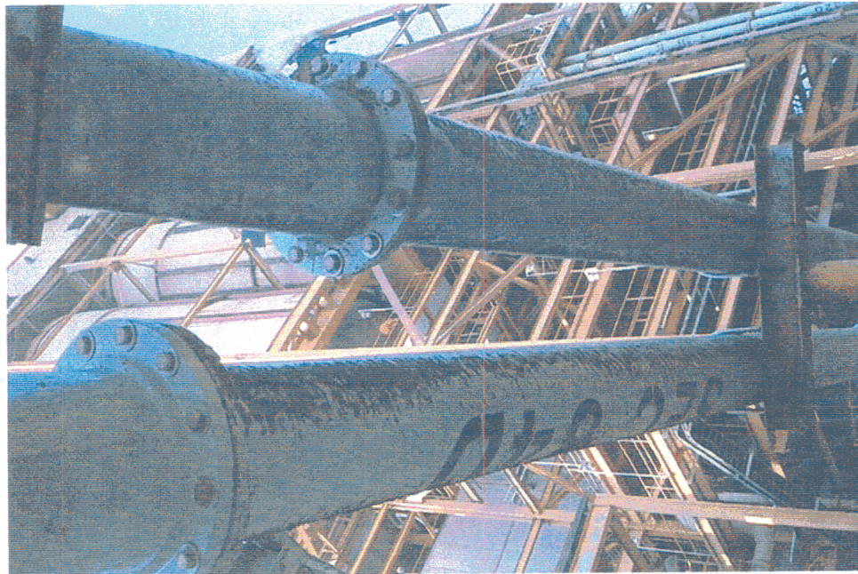
PHOTO 10 Fuel Transport Pipes
