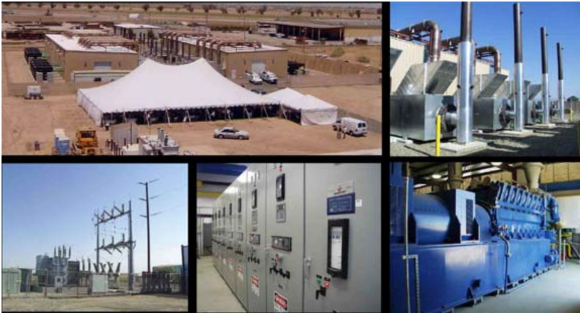
Figure 5: Chowchilla 48-MW Power Plant
