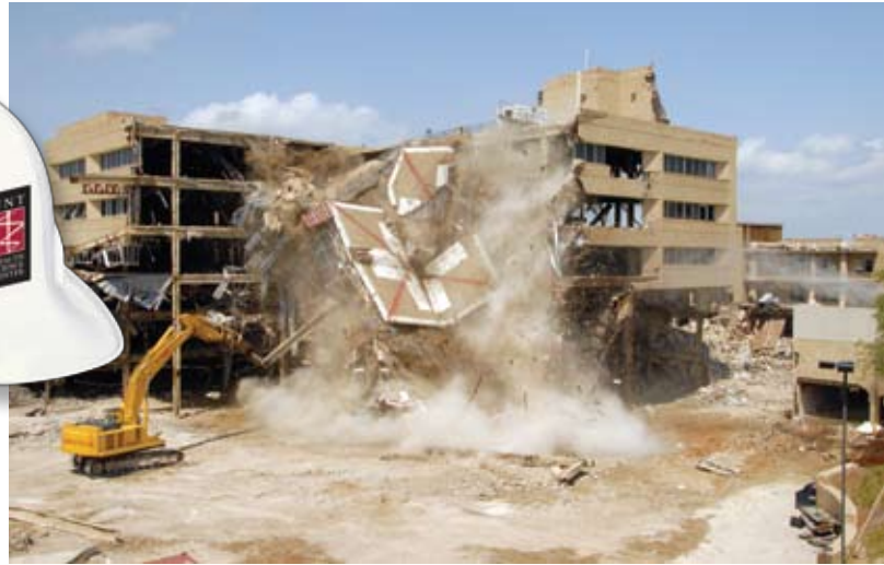
Crews demolish the center tower of the OMCT building, which included part of the emergency room, surgical and medical suites, and the helicopter landing pad on the roof.
