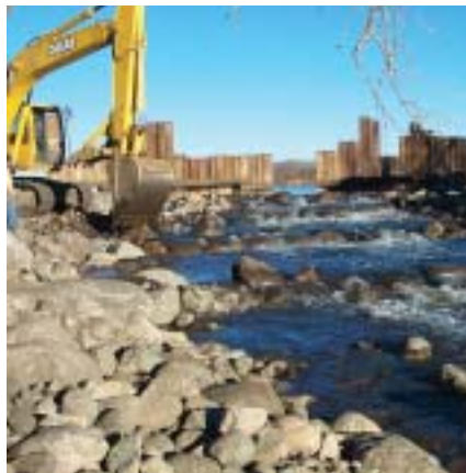
Removal of the Dutton Locks and installation of step pools on the Pelican River (MN DNR photo).
