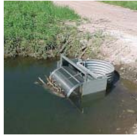
Rotary drum fish screen on East Canal
