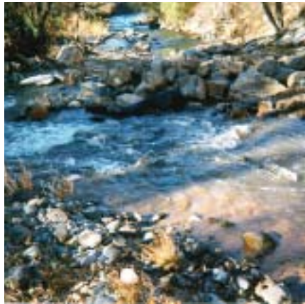
Inadequate conditions at Geronimo's Cave irrigation diversion, preventing fish passage
