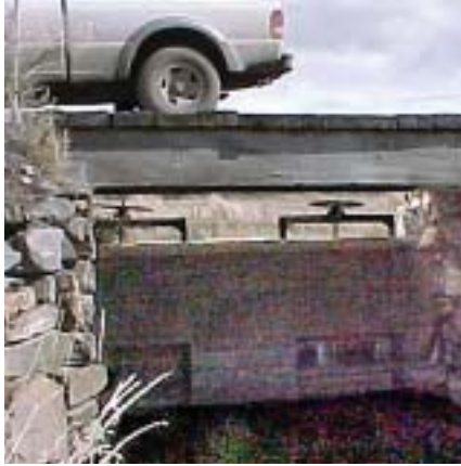
Headgate at the Bridge Creek/East Canal Bridge creates a barrier at high flows
