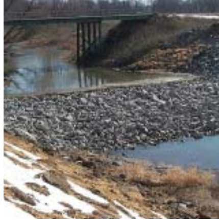
Streambed grade control preventing fish passage
