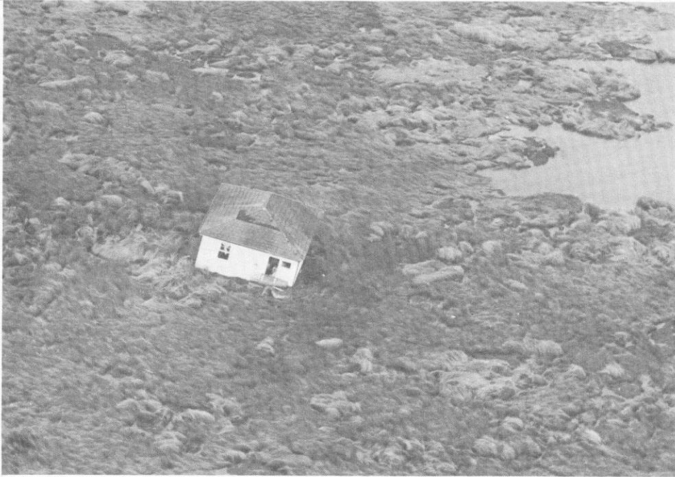
HIGH TIDE AND WIND, DELACROIX ISLAND, LA. (THIS HOME IS APPROXIMATELY 7 MILES FROM ITS ORIGINAL LOCATION.) 22 SEPTEMBER 1965
