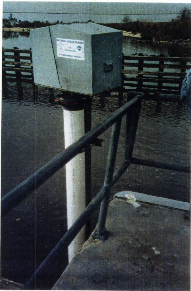
PHOTO 3 - Damaged concrete and bent south handrail on the east half of structure
