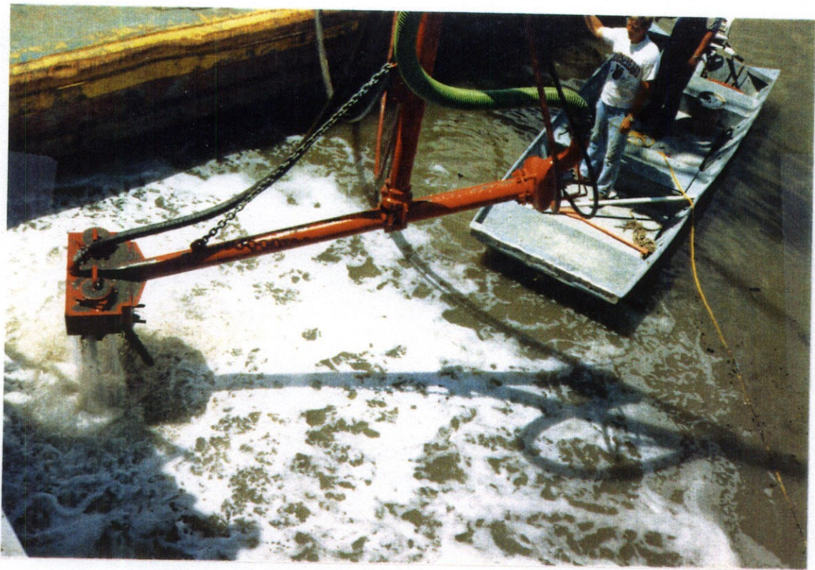
JET DREDGE WITH ACCUMULATED DEBRIS
