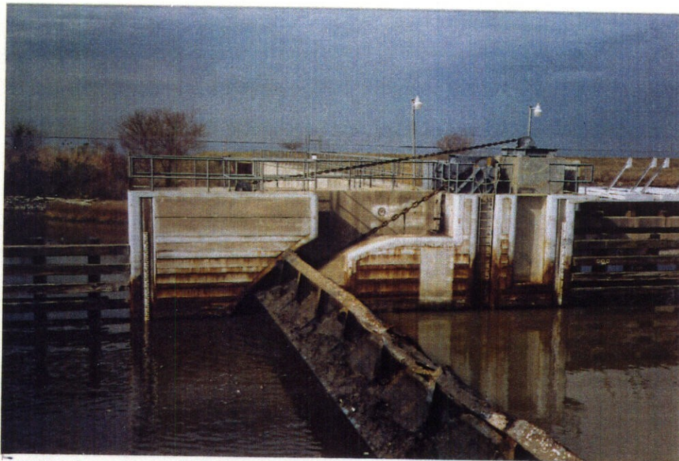
PHOTO 2 - Corroded protective wall armor, corner plate, ladder and damaged flap gate
