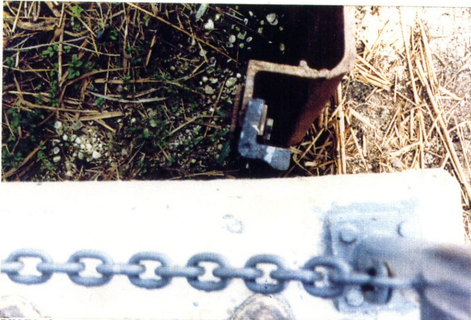
PHOTO 1 - One-half inch separation between L-Type waterstop and T-Wall monolith
