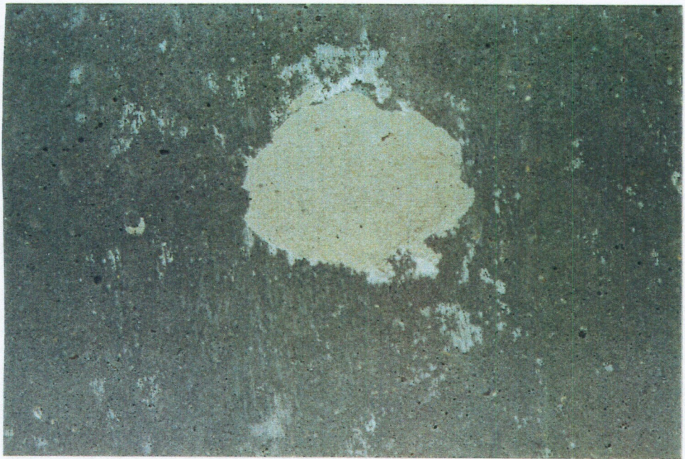
PHOTO 9: TIE ROD PATCH THAT WAS APPARENTLY REPAIRED. THE GENERAL CONDITION OF THE PATCHES IS GOOD.
