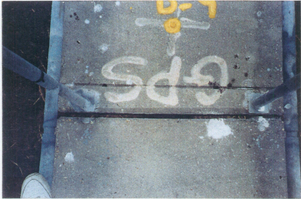
PHOTO 7: TYPICAL CONDITION OF EXPANSION JOINT BETWEEN THE T-WALL MONOLITHS. FILLER MATERIAL IS DESICCATED AND SHRUNKEN, SOME IS MISSING. NO DEBRIS IN JOINTS.
