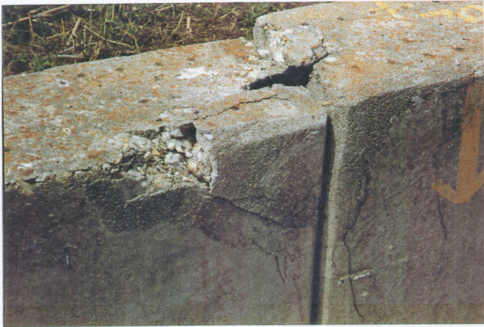
PHOTO 11: TYPICAL SPALL AT THE CORNER OF CONCRETE SHEET PILE WALL DUE TO DIFFERENTIAL VERTICAL AND HORIZONTAL MOVEMENT.
