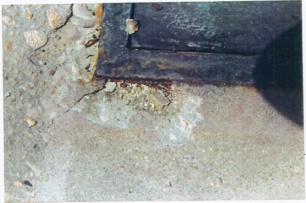
PHOTO 3: CORROSION OF METAL HATCH ON TOP OF THE SOUTH END OF THE EAST GATE MONOLITH. NOTE CONCRETE SPALLS DUE TO EXPANSION OF THE METAL.
