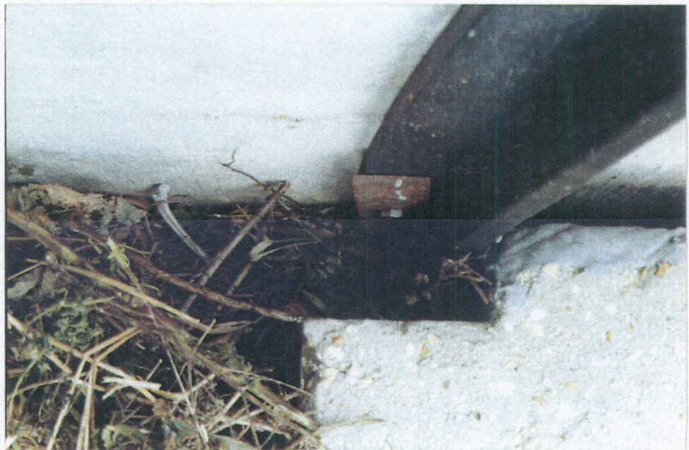
PHOTO 10: L-SHAPE WATERSTOP AT THE GATE MONOLITH AND WINGWALL JOINTS. NO EVIDENCE OF MORE SOIL LOSS THRU JOINTS.
