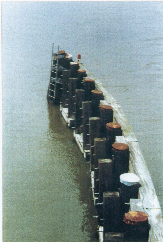
PHOTO 12: TIMBER GUIDEWALL WITH RUSTED PILE CAPS AND UNCAPPED WALERS. THE GUIDEWALL HAVE BEEN IN PLACE FOR 18 YEARS AND ARE IN GOOD CONDITION.
