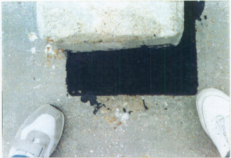
PHOTO 1: JOINT BETWEEN T-WALL AND CONCRETE SHEET PILE WALL ON WEST SIDE. THE SHEET PILE WALL HAS SEPARATED APPROX 6" TO THE WEST. THE TOP SEALANT IS MISSING LEAVING A VERY DEEP AND WIDE OPENING.
