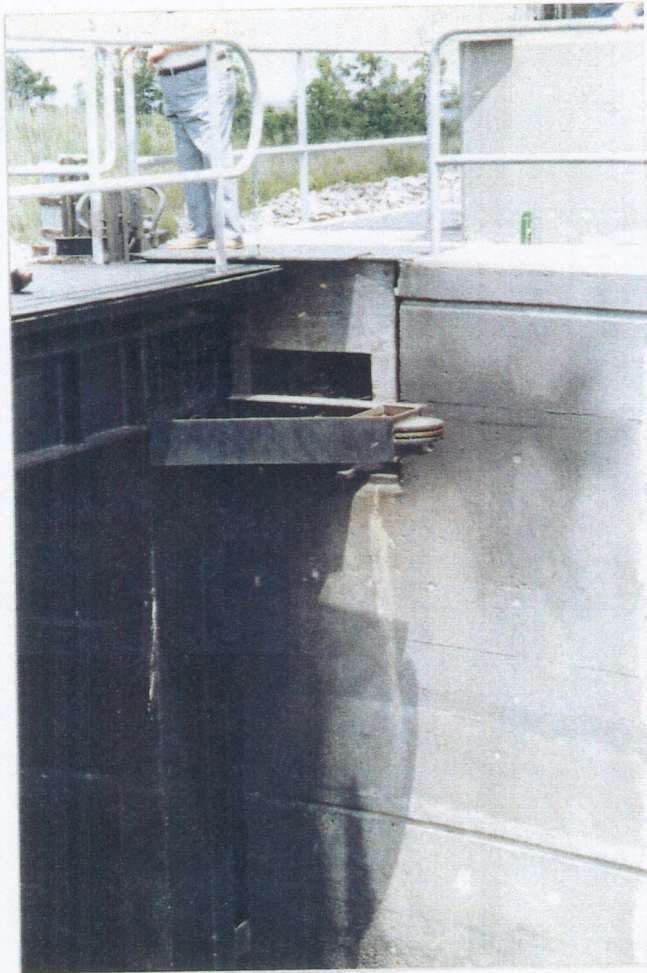
PHOTO 5: VERTICAL SHRINKAGE CRACK OFF THE EAST GATE HINGE RECESS. NOTE EFFLORESCENCE. NO APPARENT CHANGE SINCE INSPECTION NO. 4.
