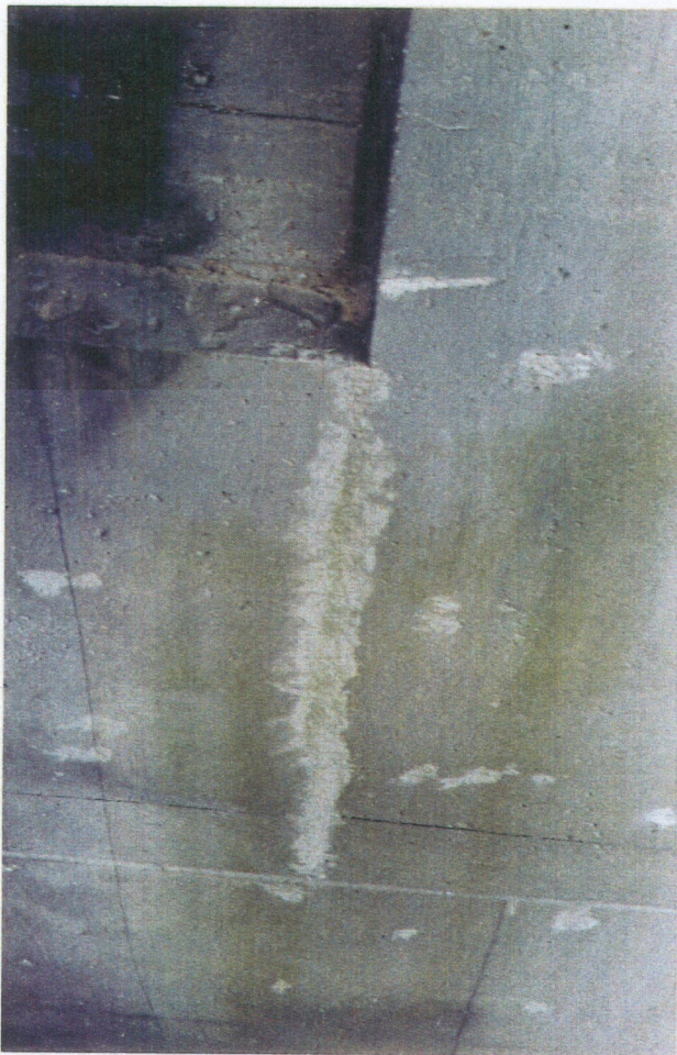
PHOTO 2: VERTICAL SHRINKAGE CRACK OFF THE WEST GATE HINGE RECESS. NOTE EFFLORESCENCE.
