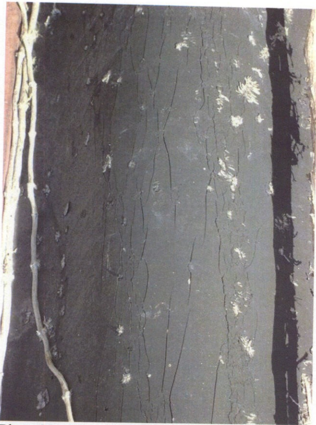
Photo No. 25 – Weathering condition of a monolith joint seal. (Typical).
