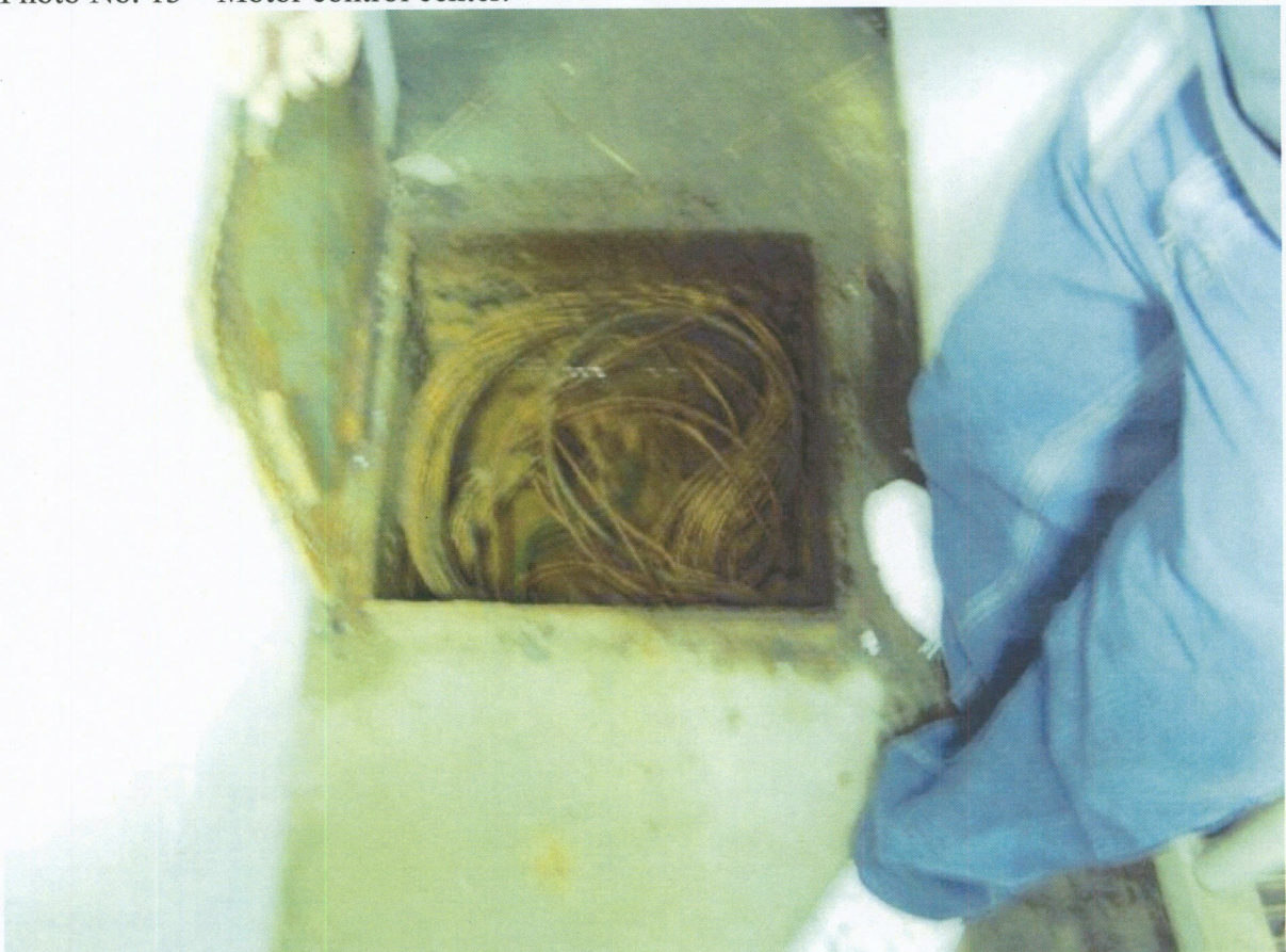
Photo No. 14 – Conductor junction box.
