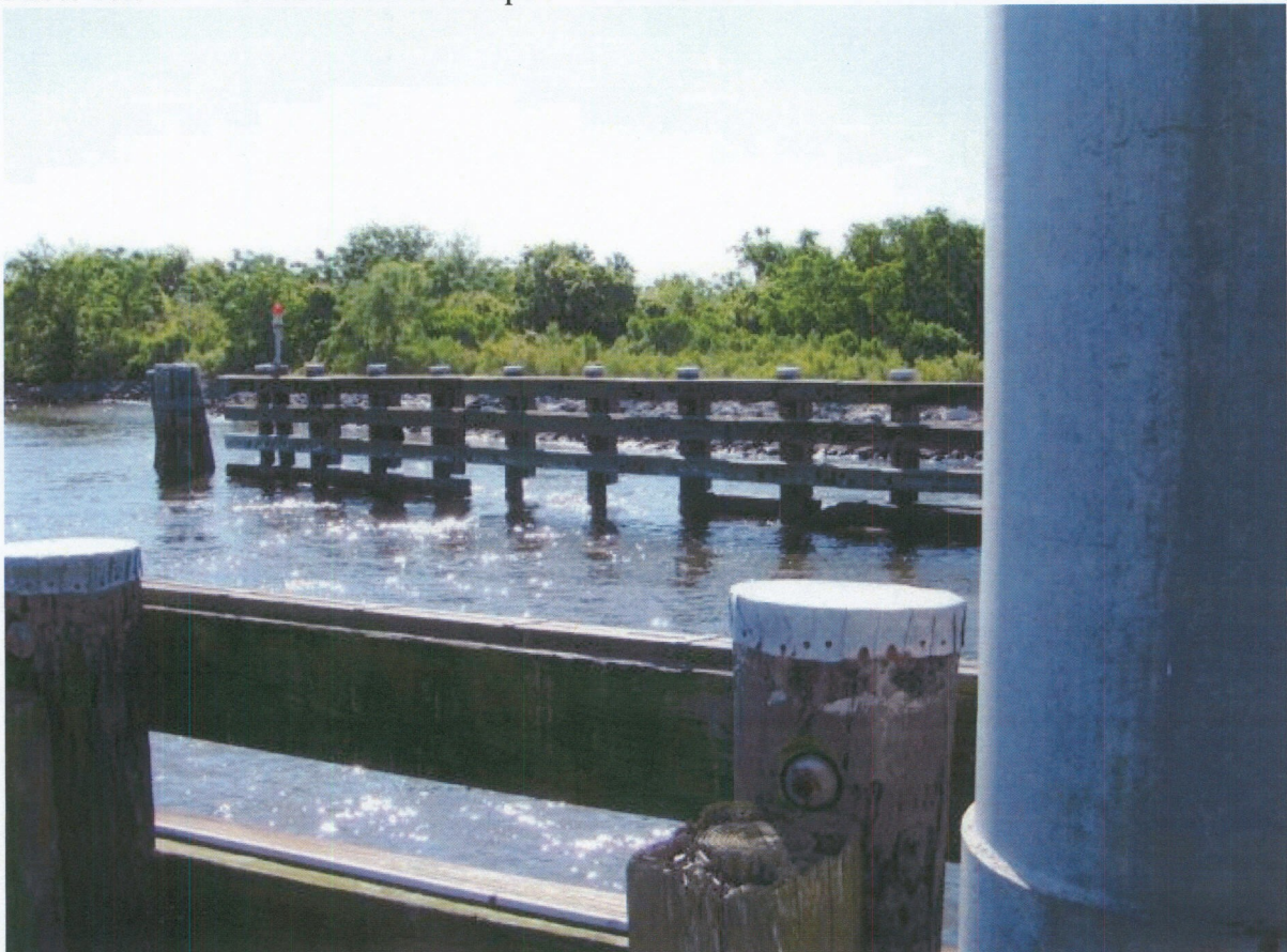
Photo No. 28 – Missing wales noted near the waterline of the northeast guidewall.
