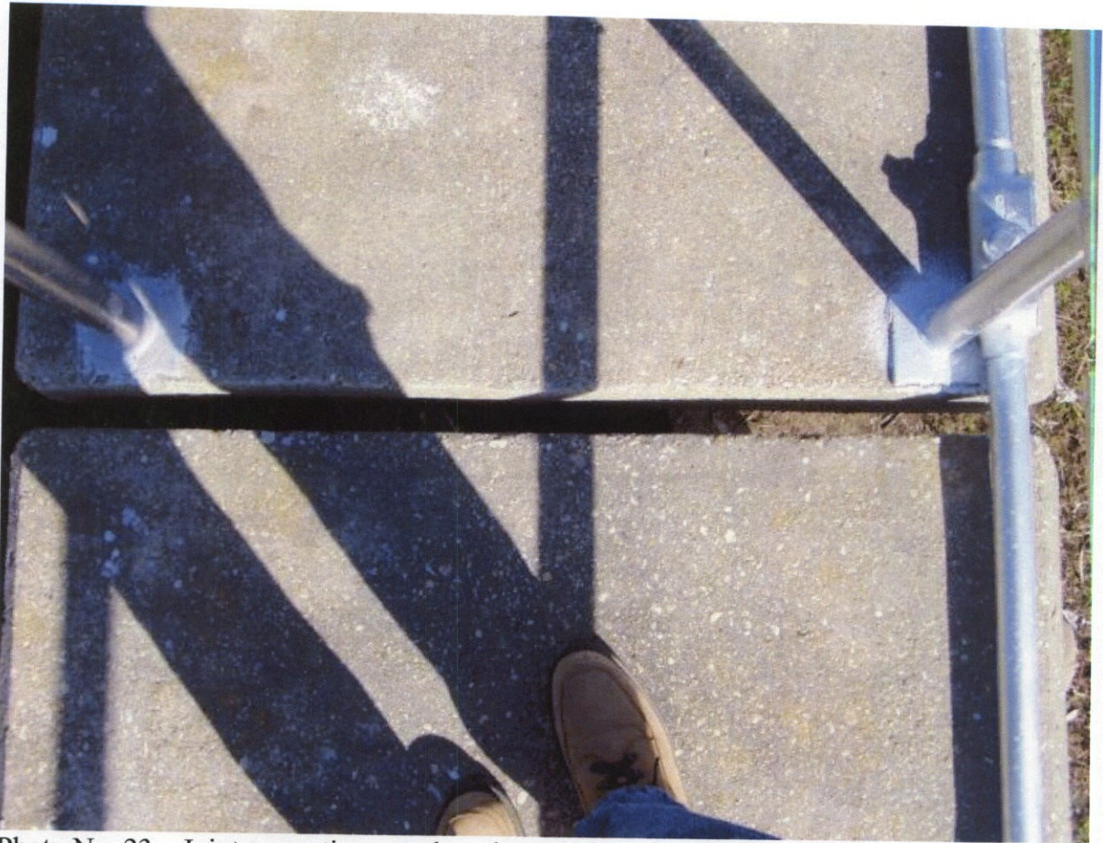
Photo No. 23 – Joint separation noted on the west inverted “T” floodwall.
