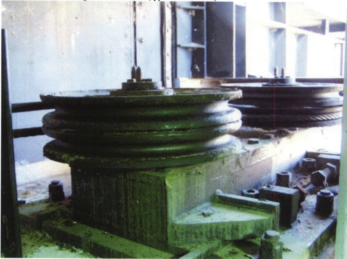
Photo No. 8 - Gate cable drives
