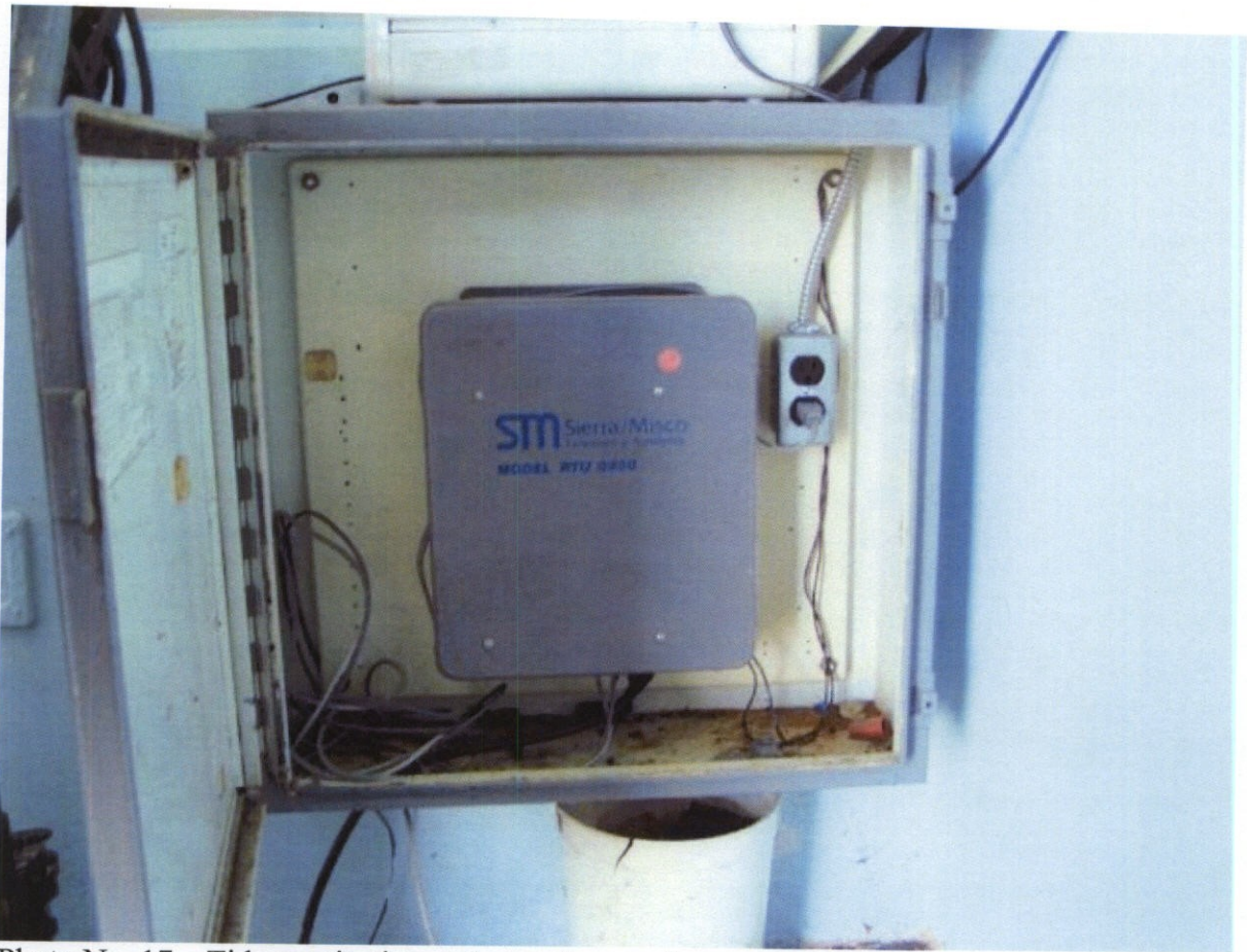
Photo No. 17 – Tide monitoring and reporting equipment.
