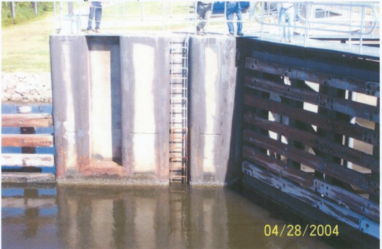
Photo No. 4 – Corrosion of the ladder, corner protection and needle beam recess noted.
