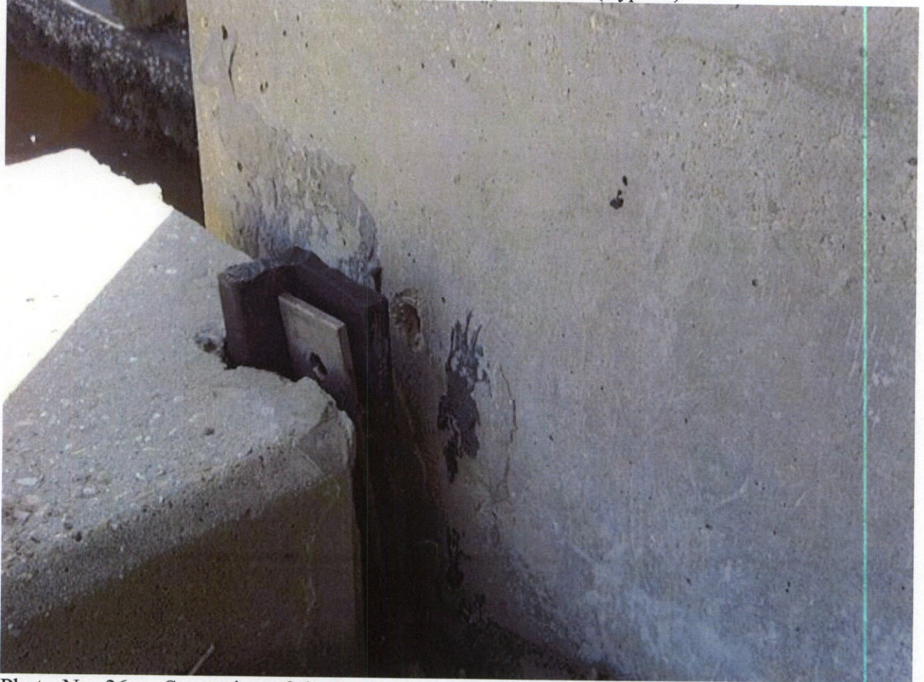
Photo No. 26 – Separation of the L-type waterstop between the west flood side wing wall and structure.
