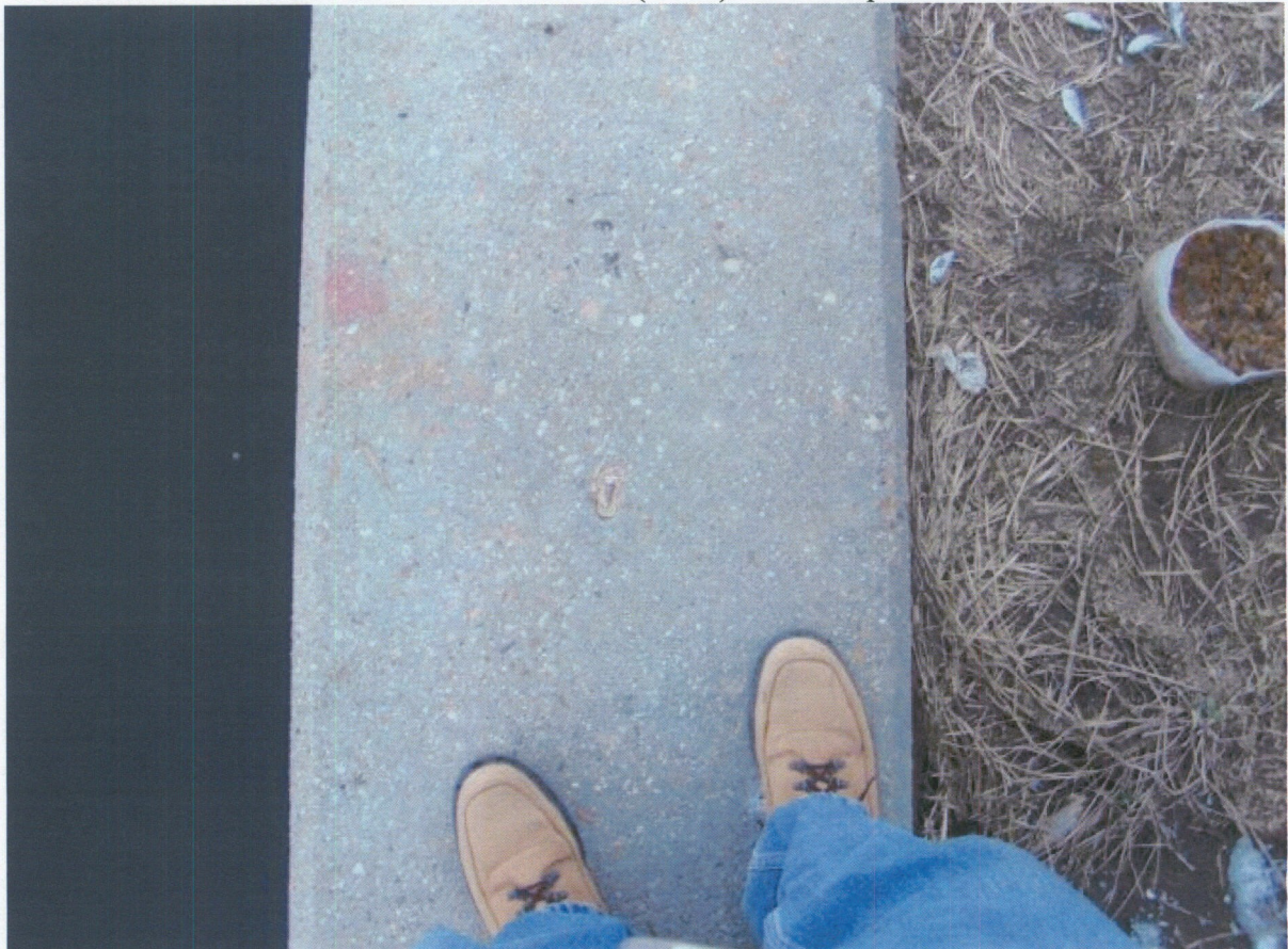
Photo No. 36 – Bent SRM noted on the southwest wing wall.
