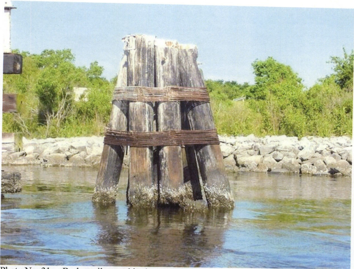
Photo No. 31 – Broken pile noted in the northwest dolphin.
