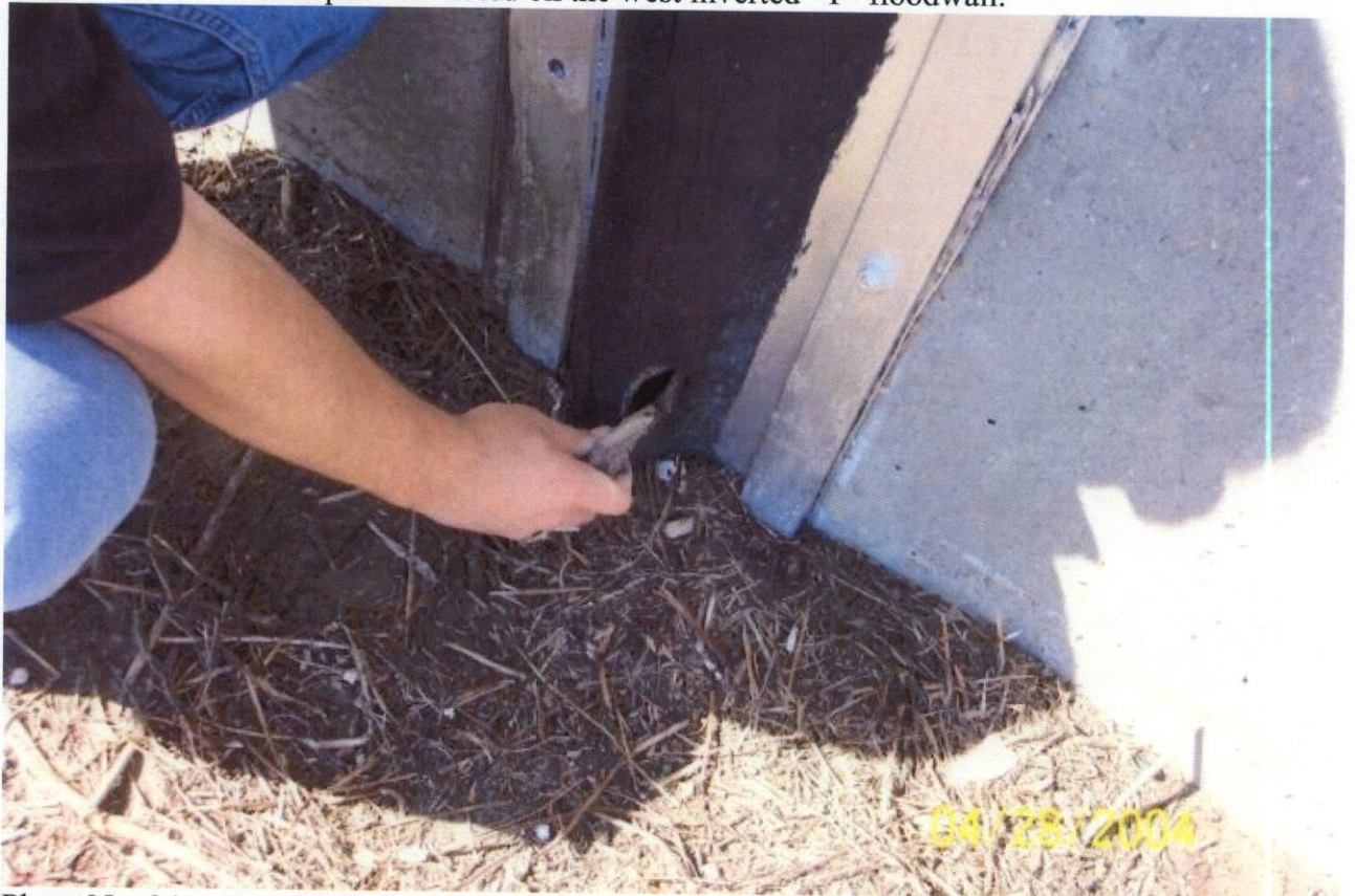
Photo No. 24 – Torn Monolith joint seal.
