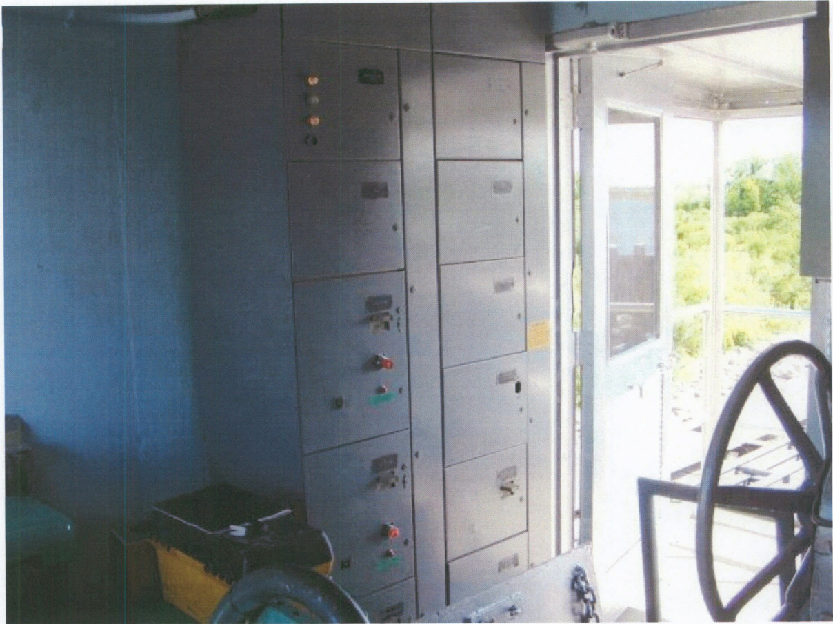
Photo No. 13 – Motor control center.
