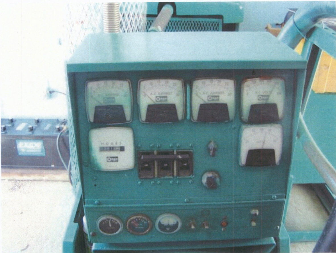
Photo No. 11 – Emergency generator set.
