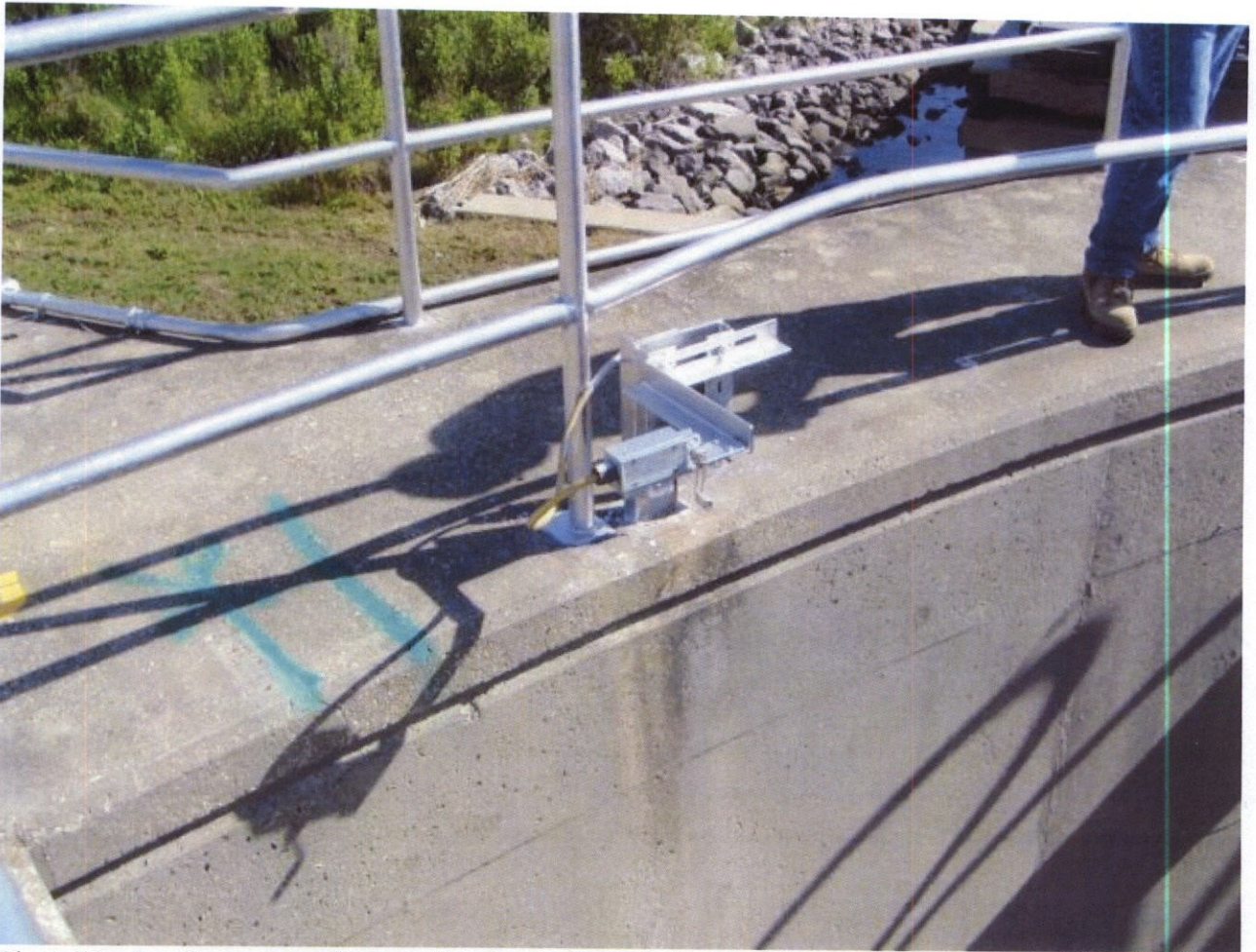
Photo No. 7 - Sector gate limit switch (typical condition).
