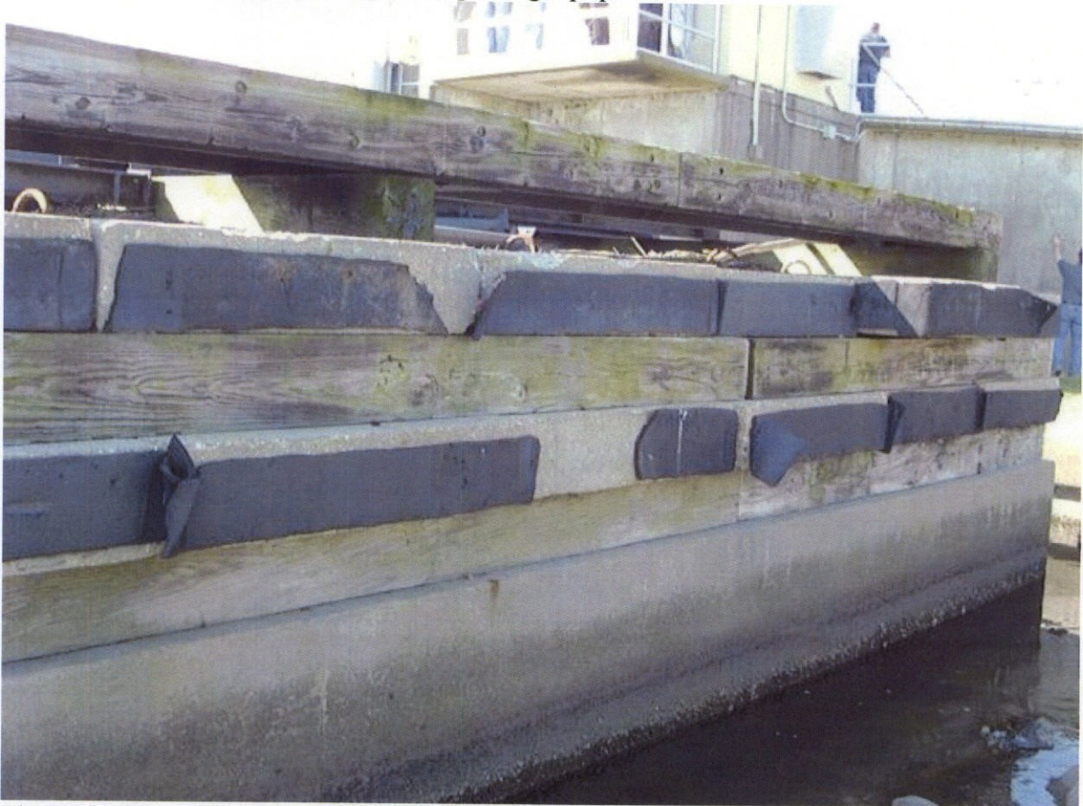
Photo No. 18 – Concrete needles with noted damage to the rubber seals.
