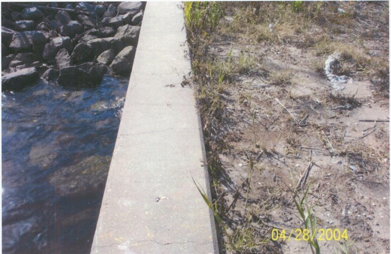
Photo No. 22 – Cracks observed on a wing wall. (Typical).
