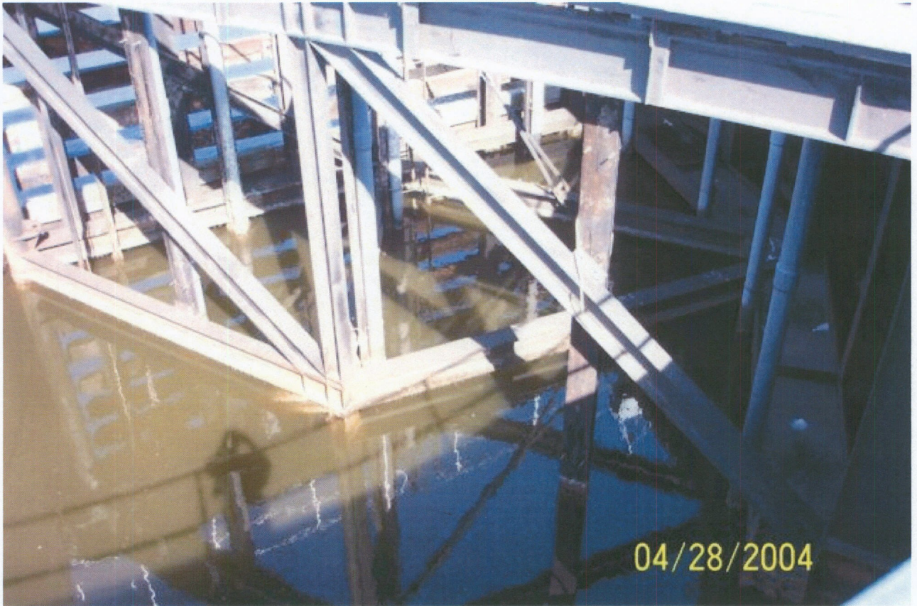
Photo No. 3 – Sector gate members; corrosion at waterline noted.
