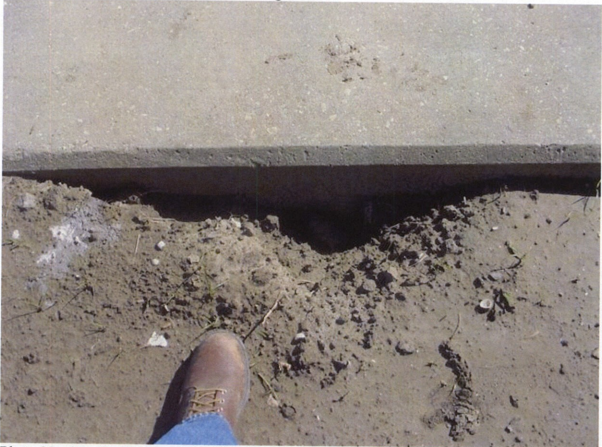
Photo No. 34 – Evidence of material loss noted adjacent to the wing walls.
