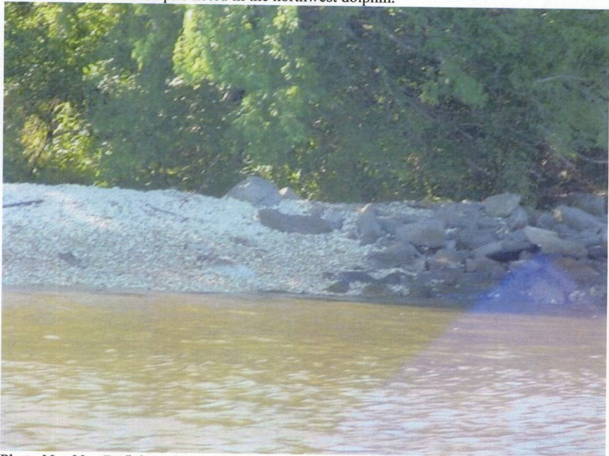
Photo No. 32 – Deficient rip rap slope protection noted on the east channel slope, floodside side of structure.
