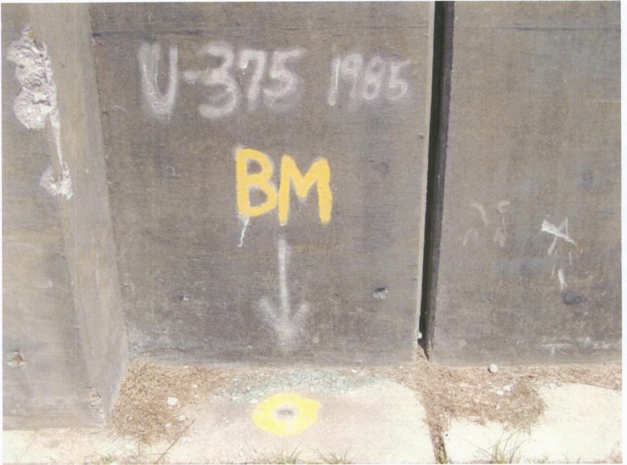
Photo No. 37 – PBM U-375 – located at the floodgate approximately 1 mile west of the structure along the levee alignment.
