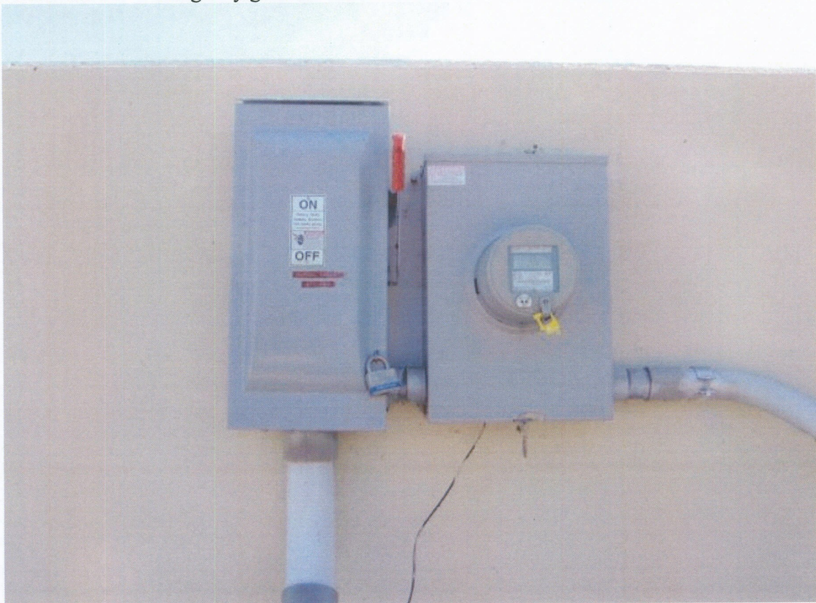
Photo No. 12 – Manual transfer switch for commercial to generator power.
