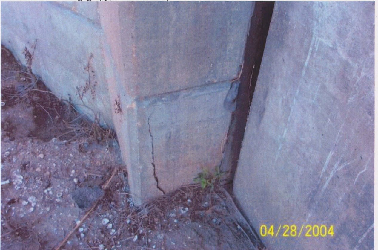
Photo No. 2 – Structural crack noted in the east gate bay monolith, just adjacent to the inverted “T” Floodwall.
