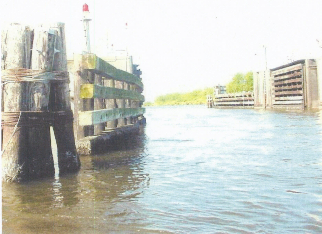
Photo No. 30 – Broken pile noted in the northeast dolphin.
