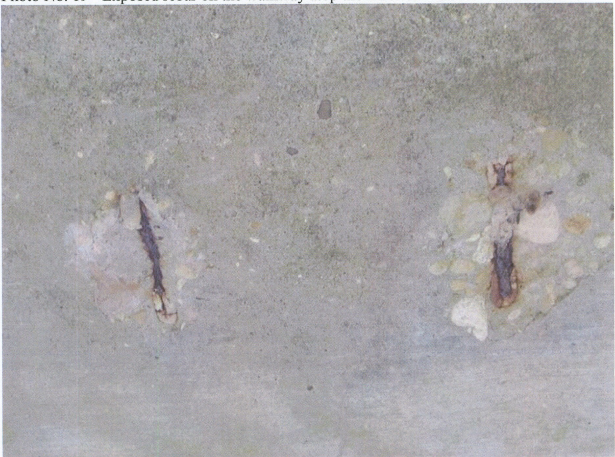
Photo No. 20 – Rebar chair corrosion noted on the inverted west "T" floodwall, flood side.
