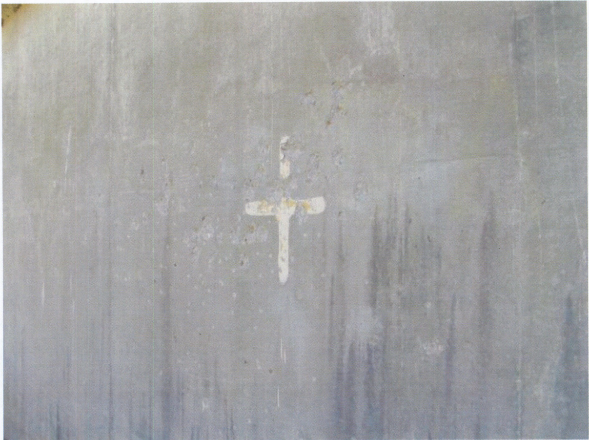
Photo No. 21 – Gunfire damage on the inverted east “T” floodwall, protected side.
