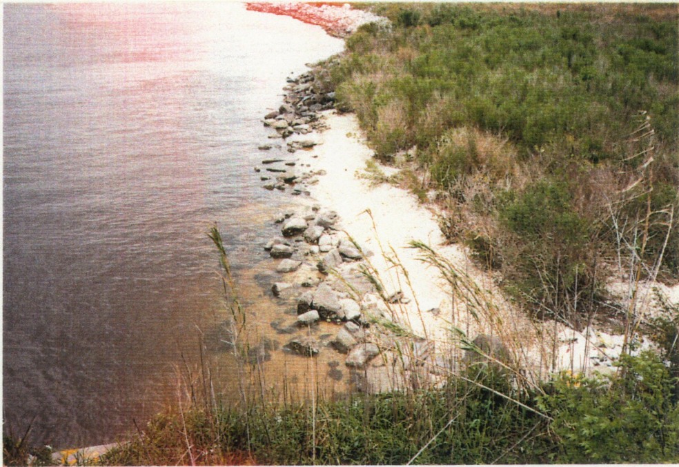
Photo 1-Deficient Riprap(Typical for the banks along the north and south approach channels)
