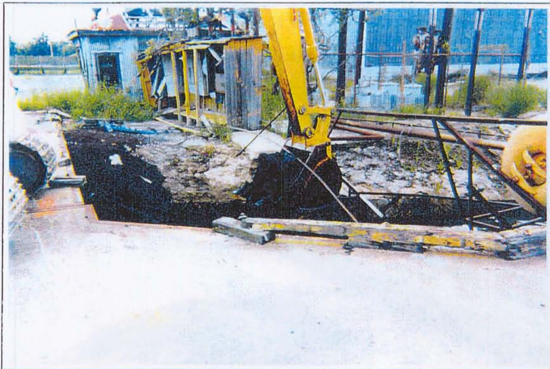
22. A view to the east of Sampling Location IEBS-16. Abandoned transformers can be observed in the background of the photograph.
