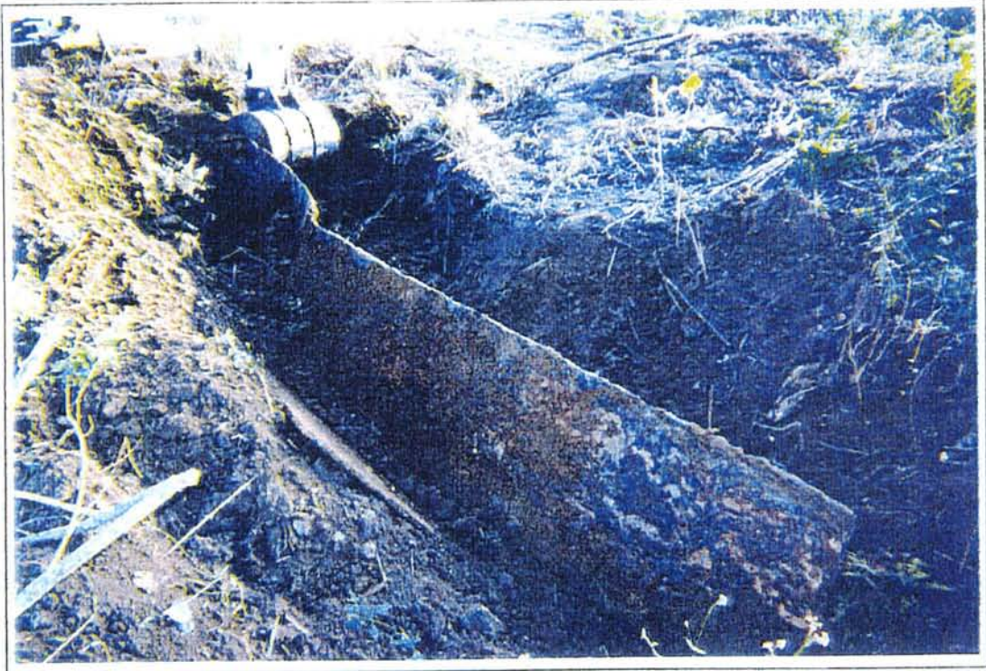
41. View of the metal plate in Test Pit TP-75-250-1.
