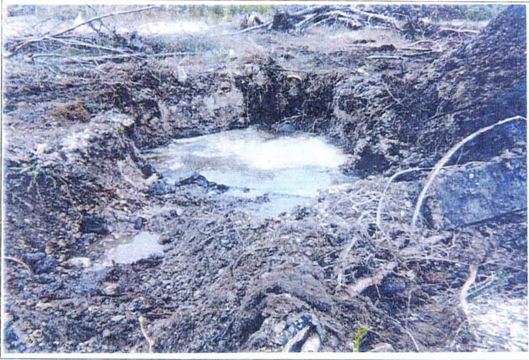
31. View to the northwest of TP 0-15-1 backfilled with water trapped under the large metal plate observed in test pit.
