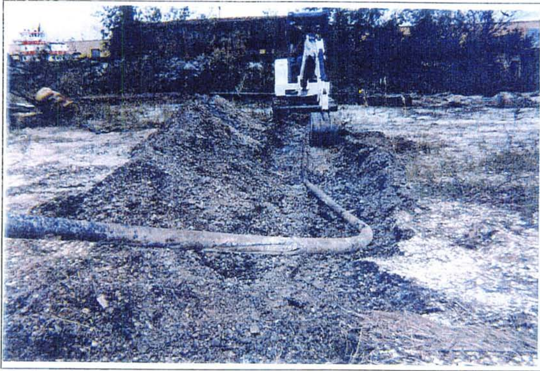
27 View to the west/southwest along the 6" line from the former AST pad area
