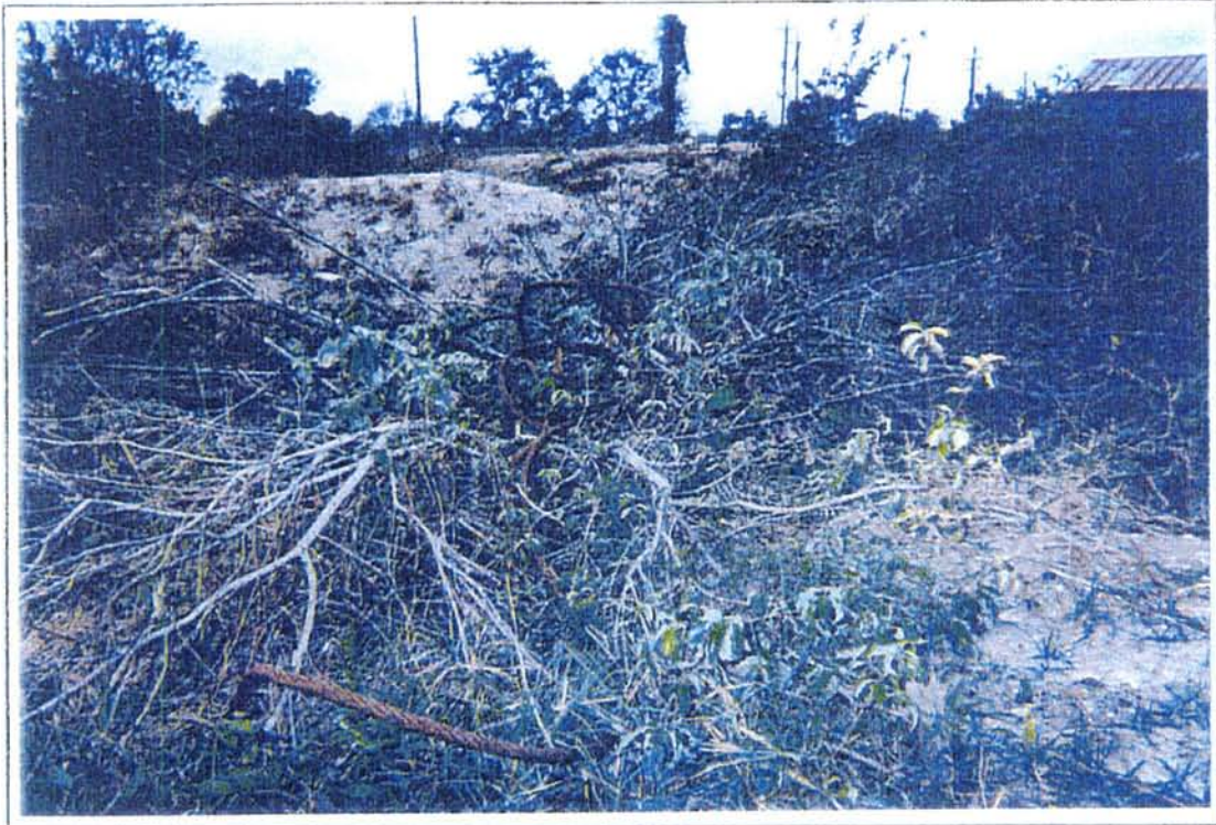
5 View to the south of a tangled wire rope observed on the north side of the small blast sand stockpile.
