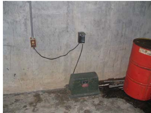
Sewage Aerator Motor
