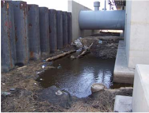
Erosion at Pump Station No. 7
