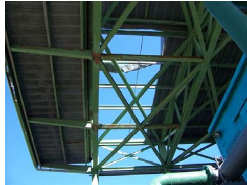
Damage to the Roof
