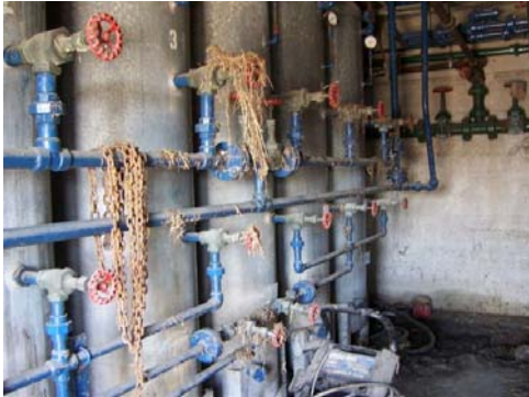
Equipment Room Air Compressors
