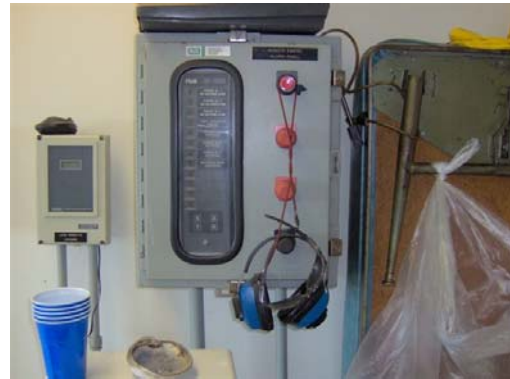
Remote Engine Alarm
