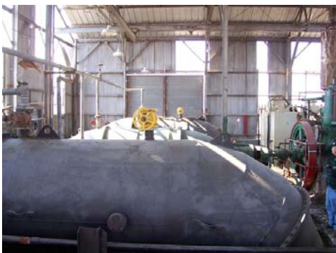
Flood Damaged Engine and Pump
