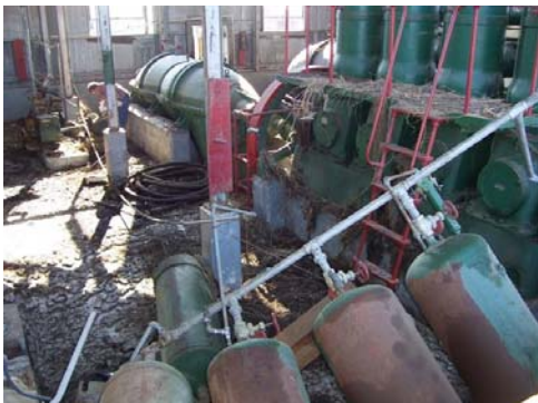
Flood Damaged Engine and Pump
