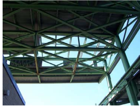
Pump Station No. 1 Roof Damage
