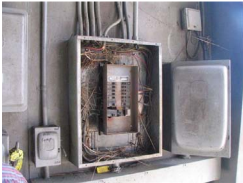
Electric Panel Box
