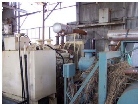
Flood Damaged Engine and Pump
