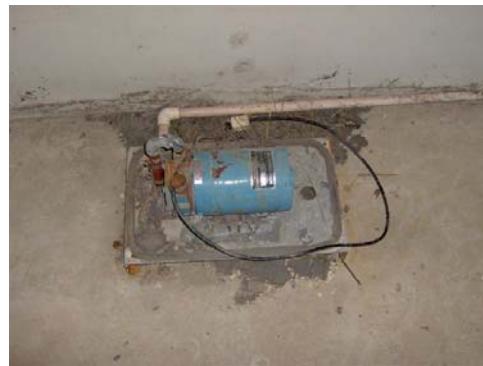
Sewage Aerator Motor
