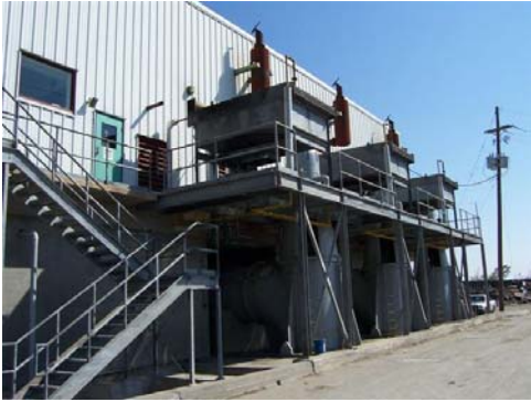
Pump Station No. 6
