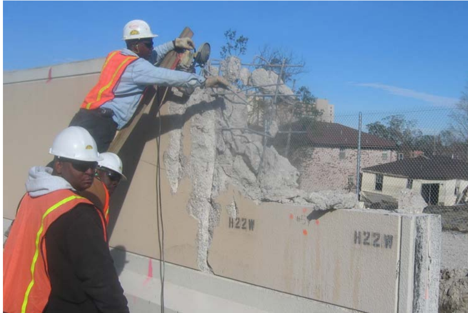
Figure K4-14. A portable electric bandsaw is used to cut rebar samples
