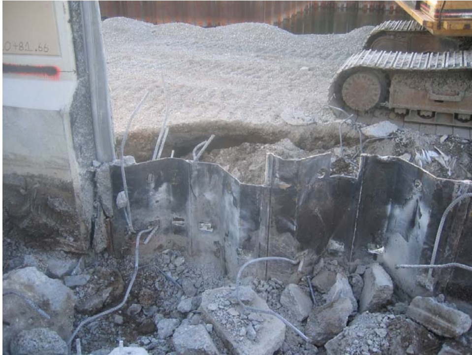
Figure K4-26. Lower top elevation of sheet piling at expansion joint
