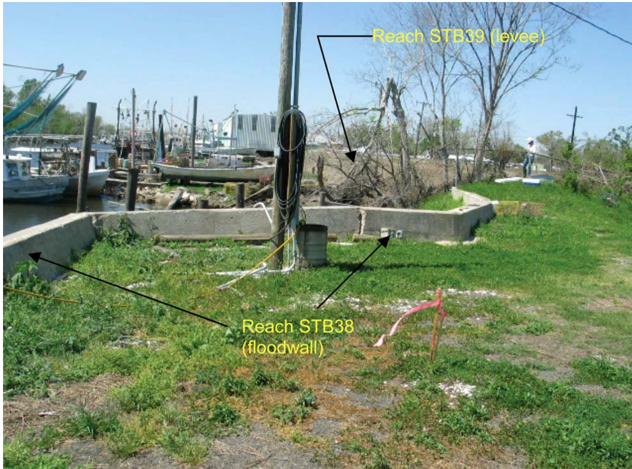
Figure STB 27. Floodwall Along the North Side of Violet Canal (This is Reach STB38 for the Risk Model, Violet Canal is to the left)
