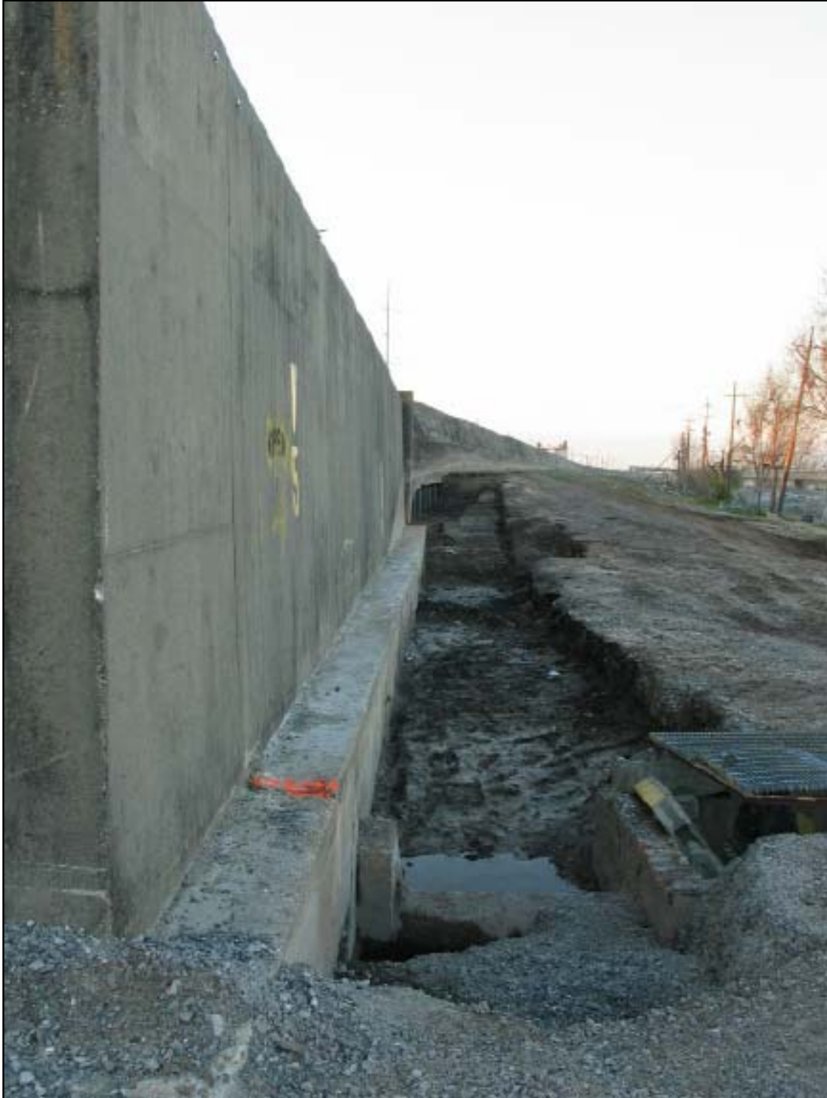
Figure NOE 21. Erosion Behind Floodwall Adjacent to Gate E-13 (IHNC East)
