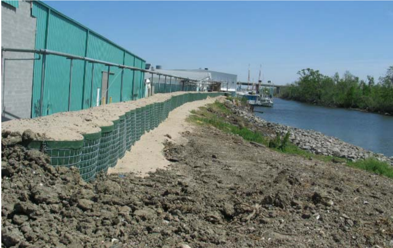
Figure STB 41. Gabion basket repairs to Reach STB40 (viewed from west side of reach)
