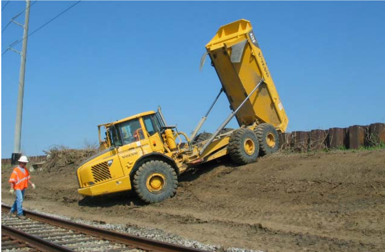
Figure STB 39. Repairs to interior local levee along Reach STB33 near parish border (Note: This section is being returned to pre-Katrina conditions)
