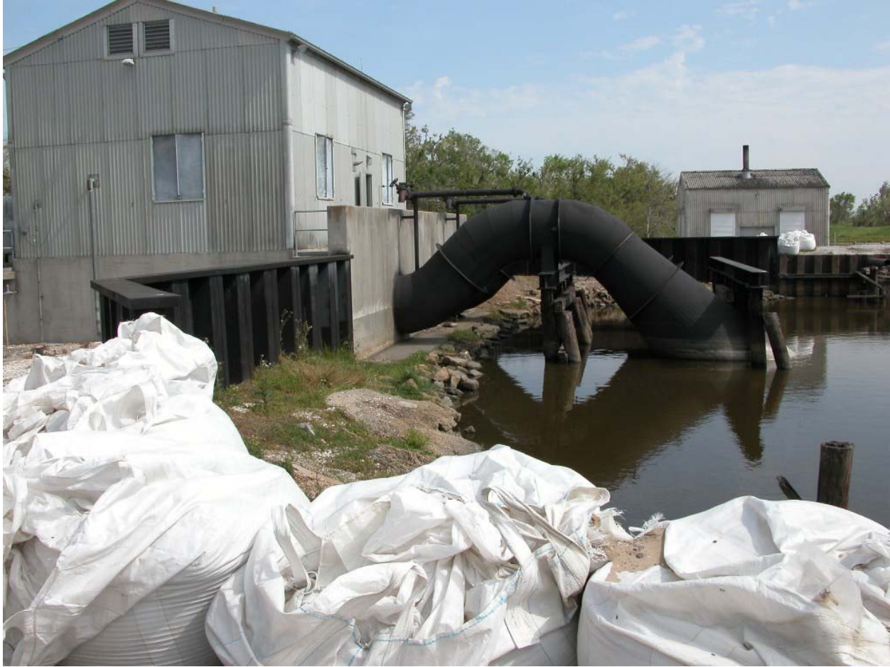
Ollie Pump Station
