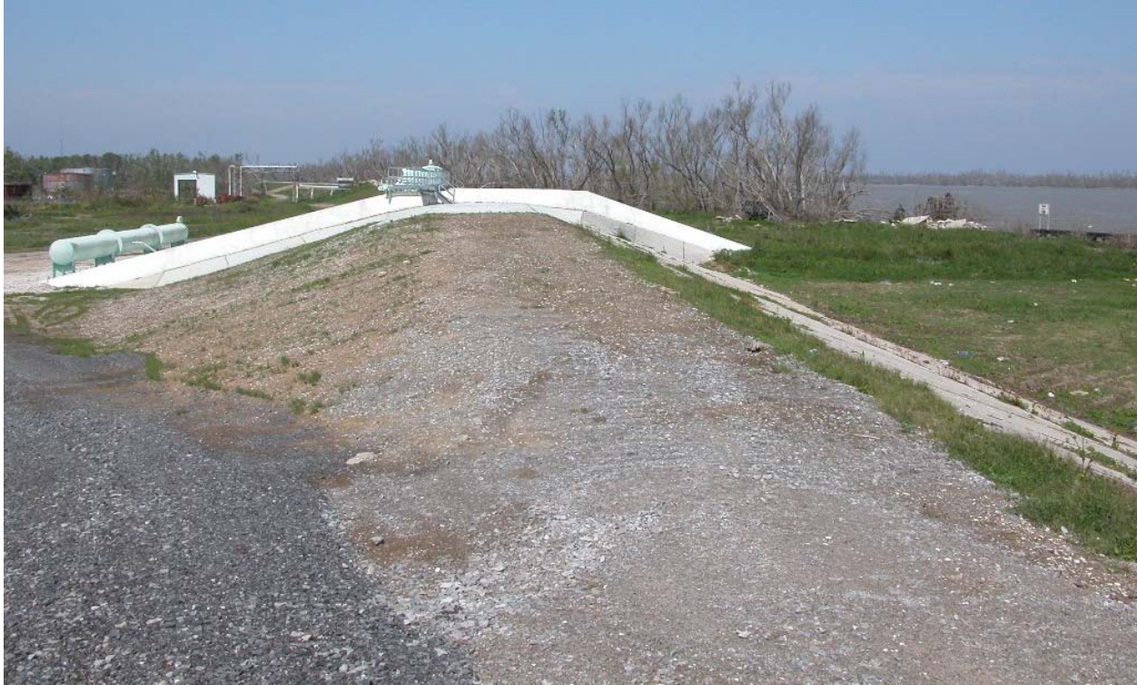
The crown of the levee is generally 10 feet wide, with most paved and some stretches gravel. Numerous pipes cross over the MRL in this area
