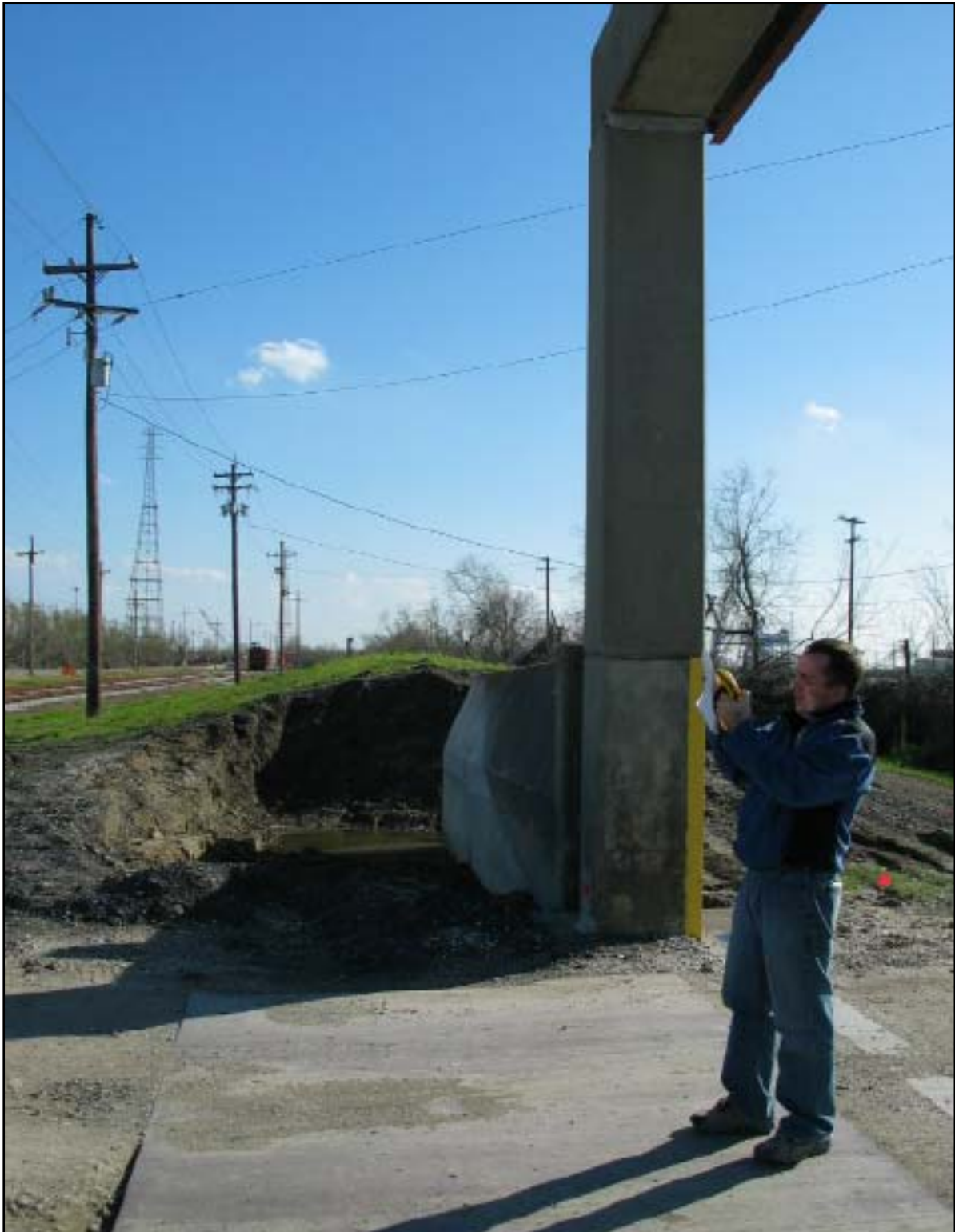
Figure NOE 18. Scour Damage around Gated Closure Along IHNC
