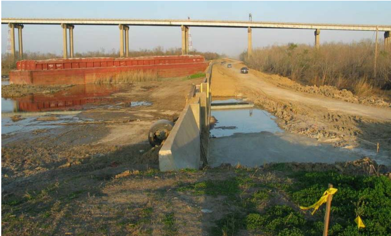
Figure STB 10. Paris Road Floodwall (Reach STB8) (looking east from the west end of the floodwall)
