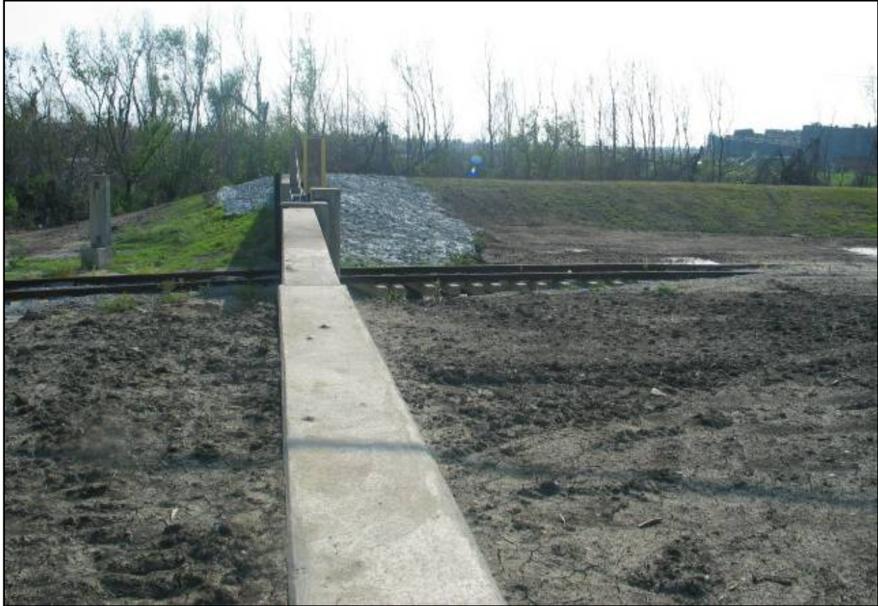
Figure NOE 36. TFG Repairs to RR Closure at the GIWW/IHNC Intersection (Note: repairs include new transition wall and grouted rock)
