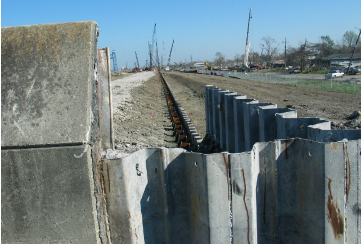
Figure STB 28. New T-wall being constructed along IHNC (Reach STB2) (looking north along the IHNC)
