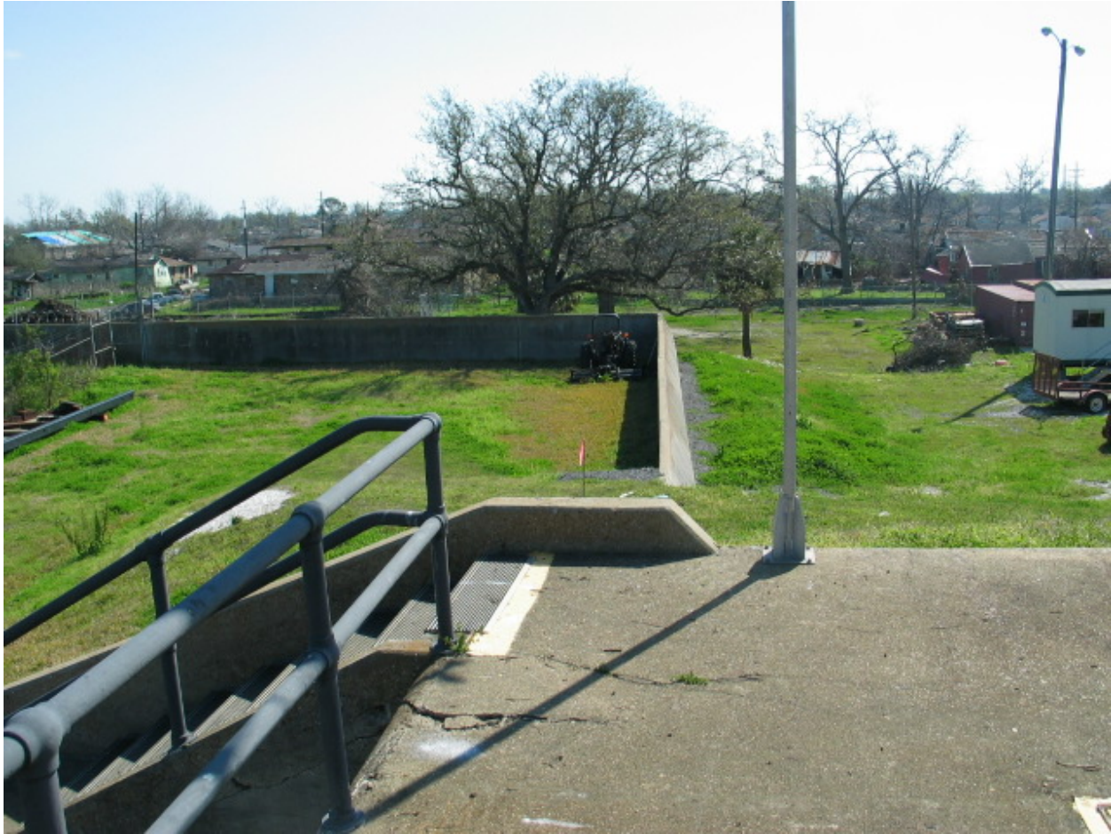
Figure STB 3. I-wall section tying into IHNC lock wall (standing on top of lock wall and looking away from IHNC)
