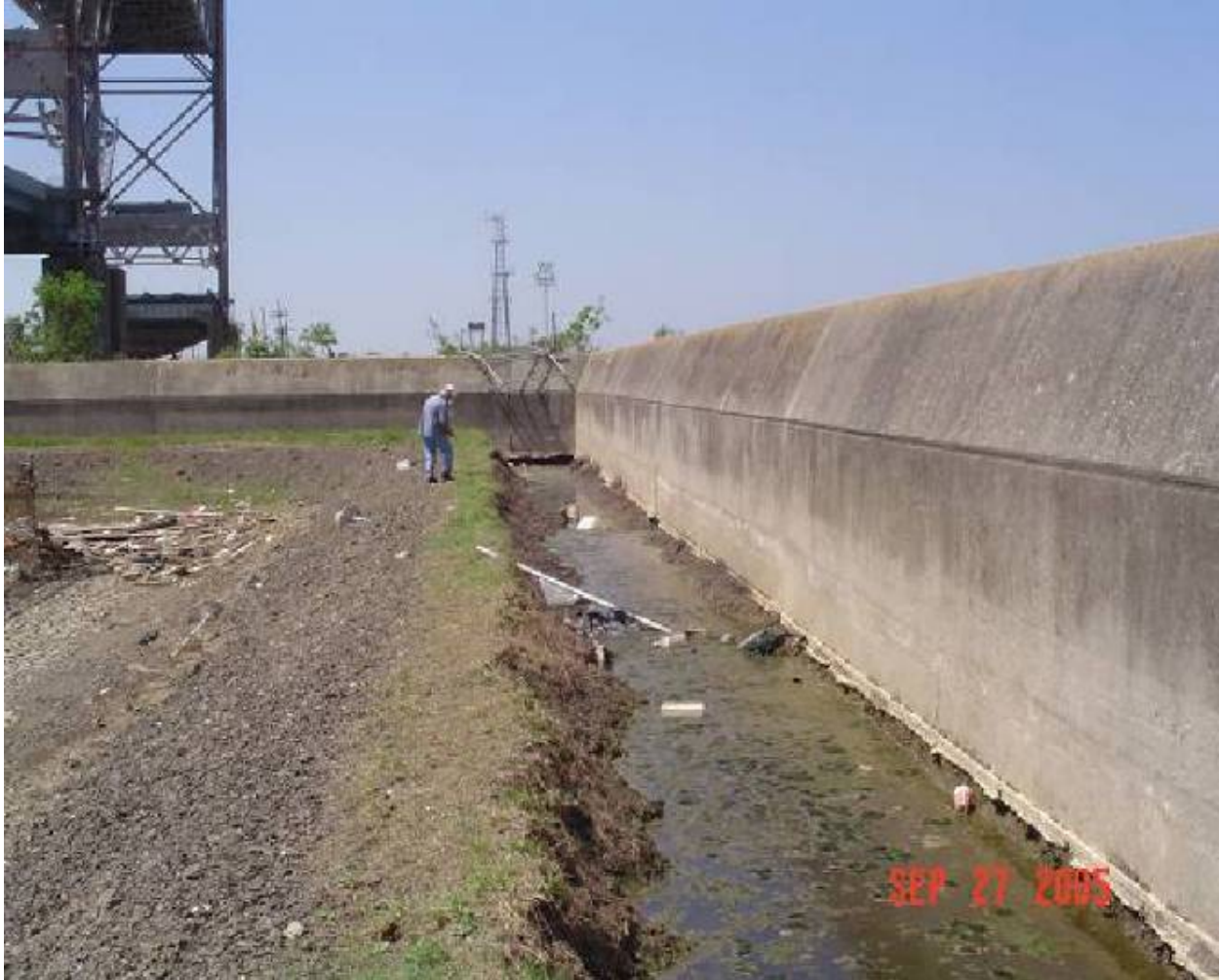
Figure STB 4. Section of Reach STB1 overtopped during Katrina (location is just north of Claiborne Avenue Bridge)
