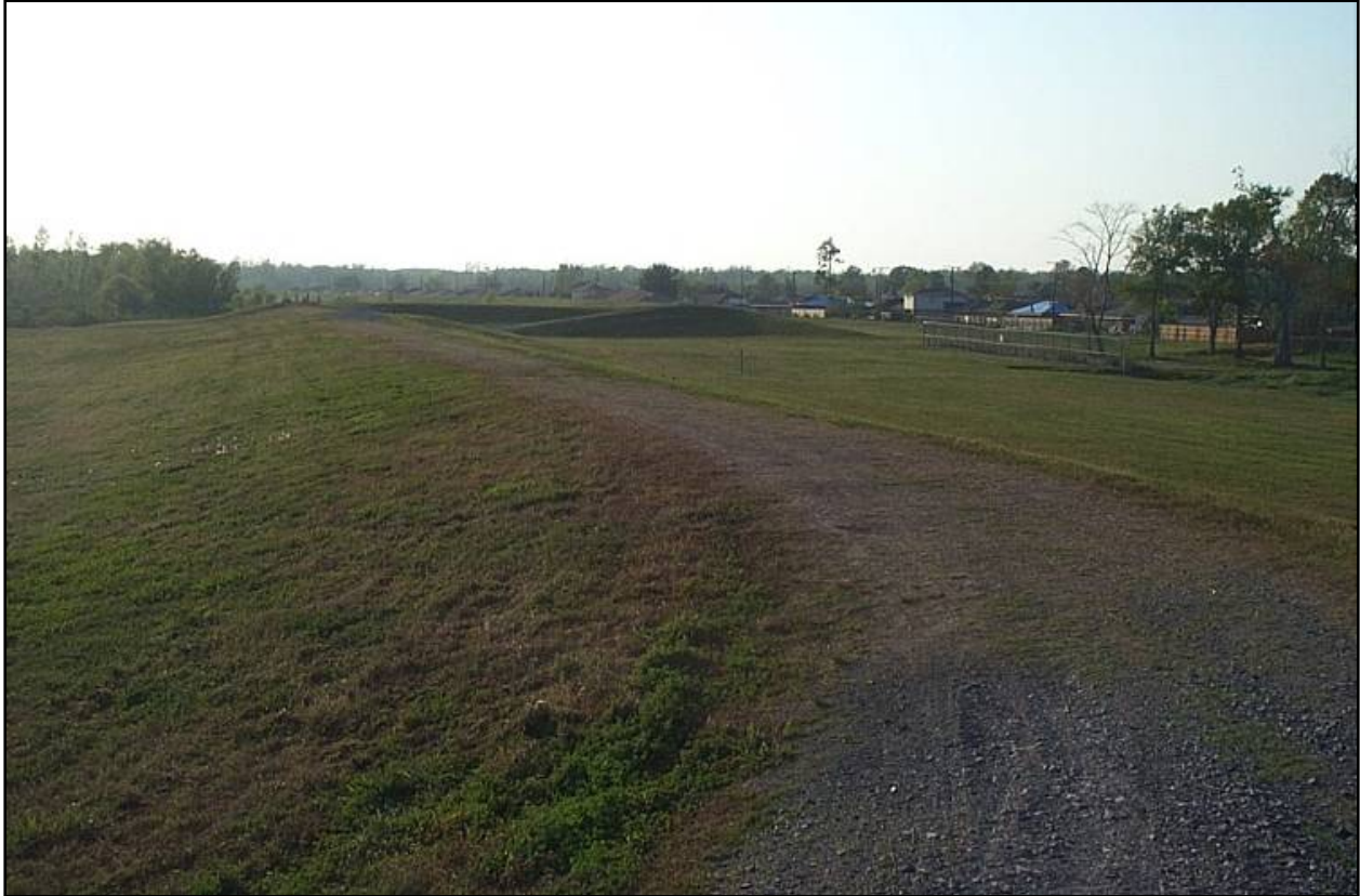
Southern tip of V-line levee
