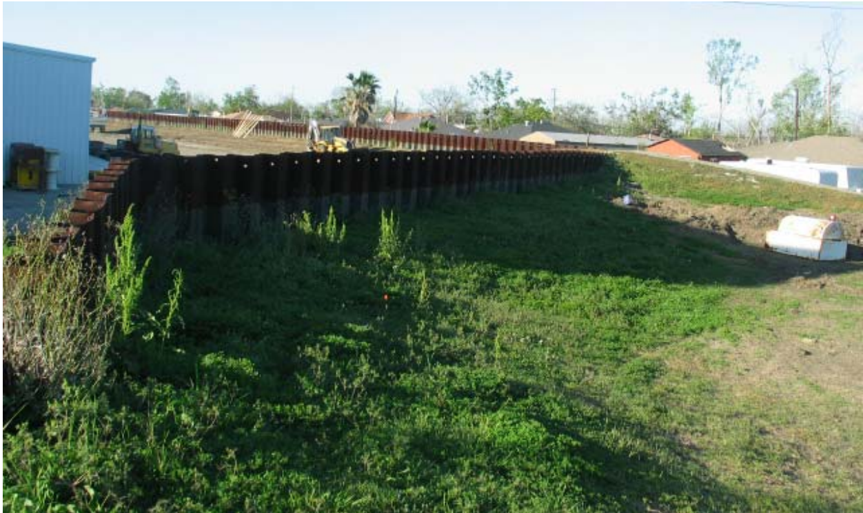
Figure STB 18. Uncapped Sheetpile I-wall near Caernarvon Canal (building on left side is on flood side)
