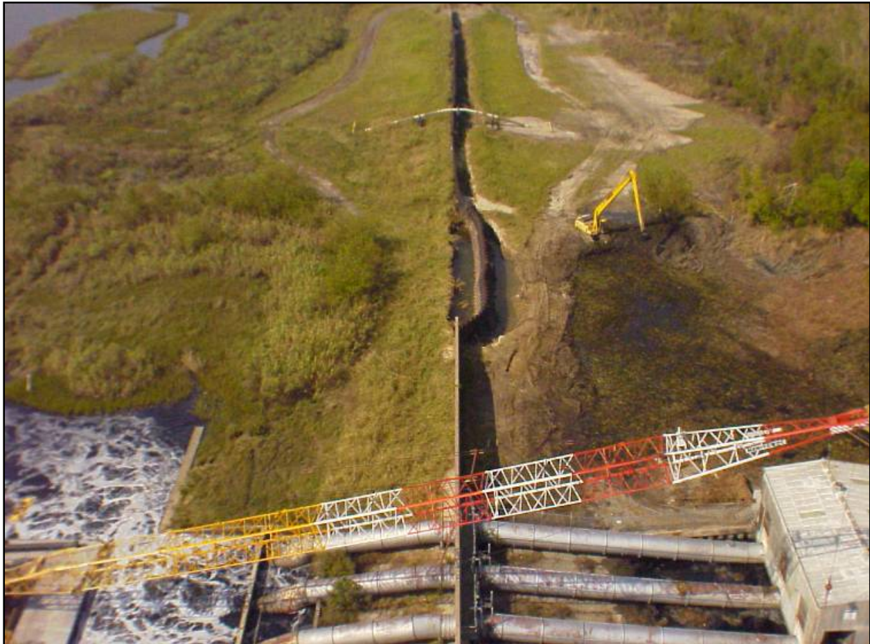
Figure NOE 12. Floodwall Failure Near Orleans Pump Station #15
