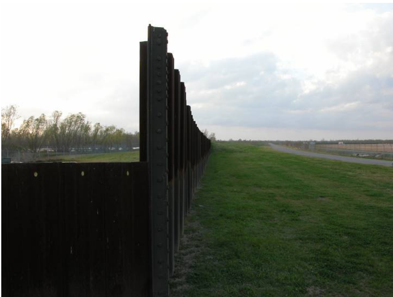
Corner of sheetpile floodwall as it turns south by the Airport runway extension (3 ft drop in elevation)
