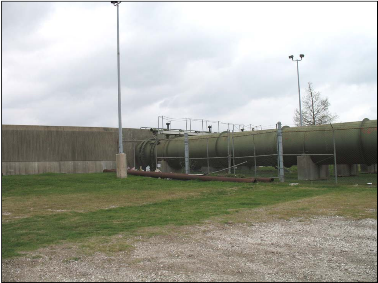
Parish Line Pump Station (Note: Pump discharge through T-wall)
