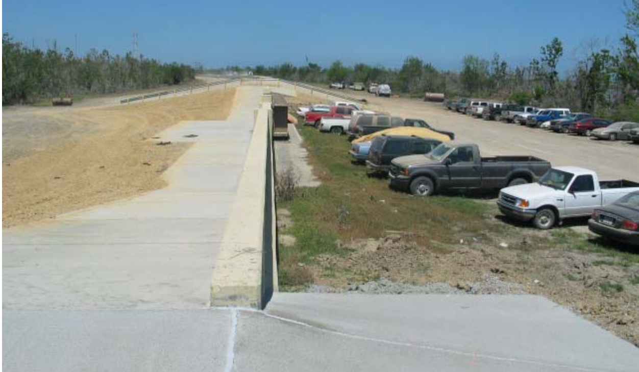
Figure STB 33. New scour protection around Reach STB10. (viewed from Bienvenue Control Structure side looking northwest)
