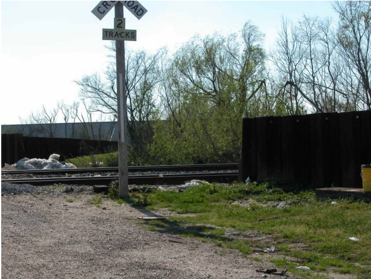
Railroad crossing has no closure gate. During Katrina it was sandbagged.
