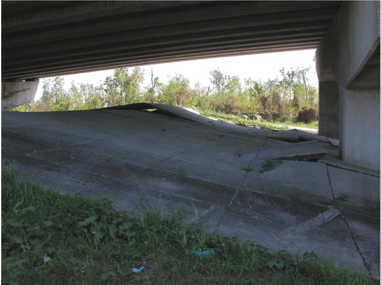
Back Levee passed under General De Gaulle onramp from Hwy 406. Buckling of concrete slab on levee under ramp.
