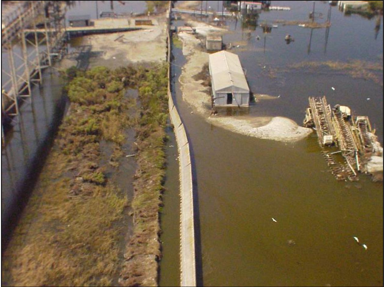
Figure NOE 16. Floodwall Failure at Bulk Loading Facility/Elaine PS
