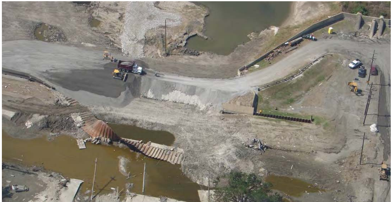
Figure STB 7. North I-wall failure within Lower 9th Ward (Reach STB2) (Note: pipes on right side of photo are associated with Pump Station #5)
