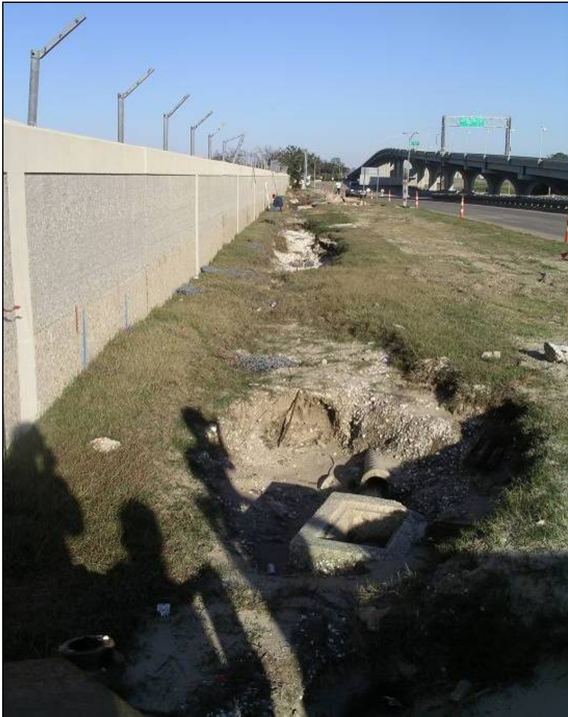
Figure NOE 4. Scour Behind Lakefront Airport FW from Overtopping
