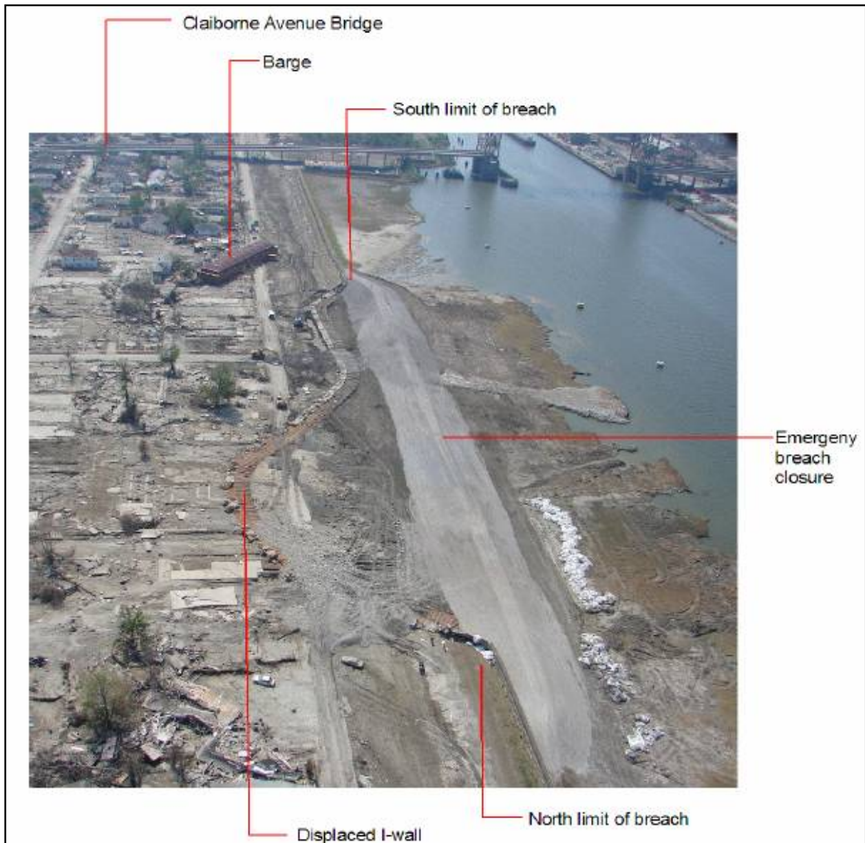
Figure STB 5. Failed I-wall section of Lower 9th Ward (Reach STB2) (looking south along IHNC)
