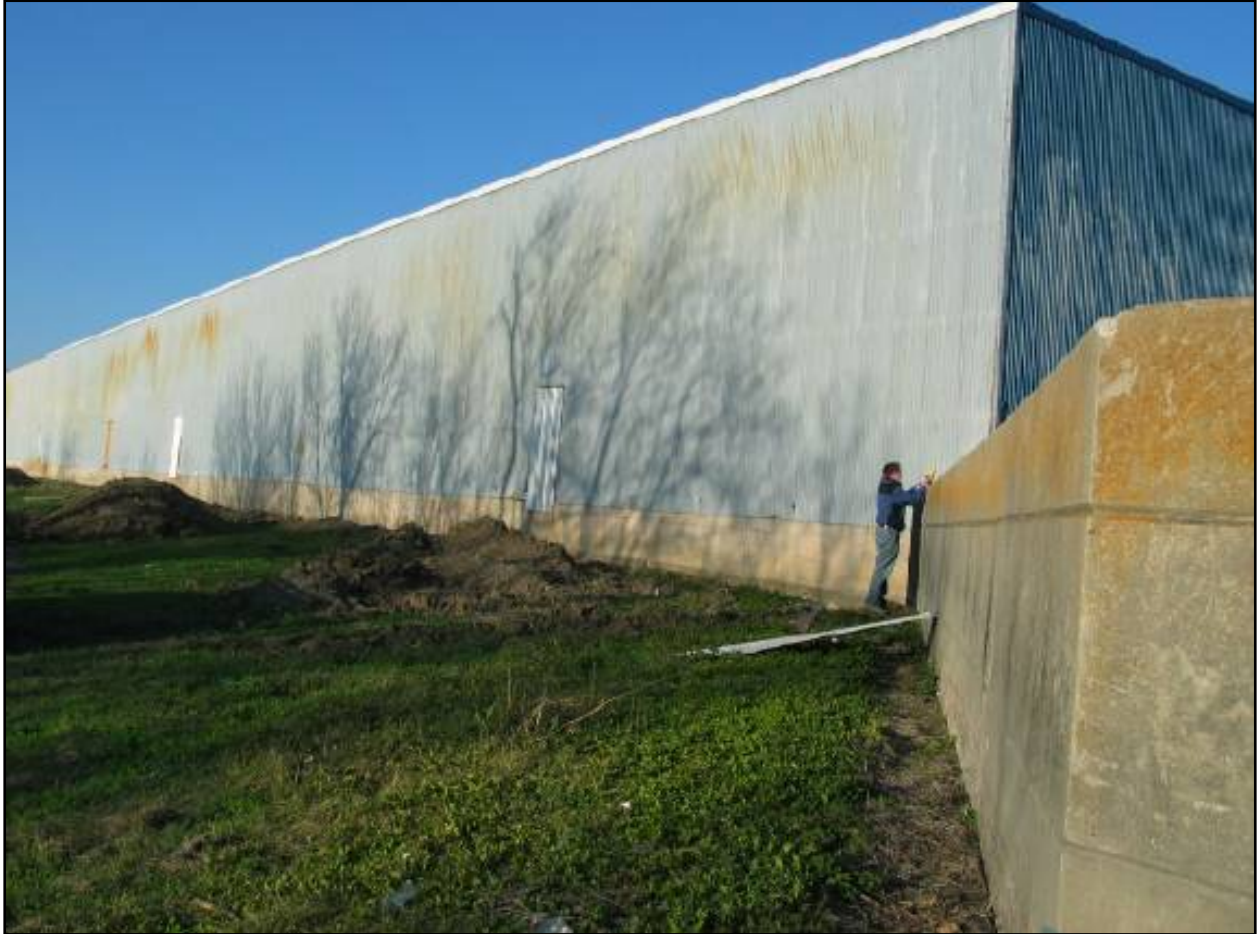
Figure NOE 20. Floodwall Serves as Building Foundation (Dupuy Storage Facility – IHNC East)
