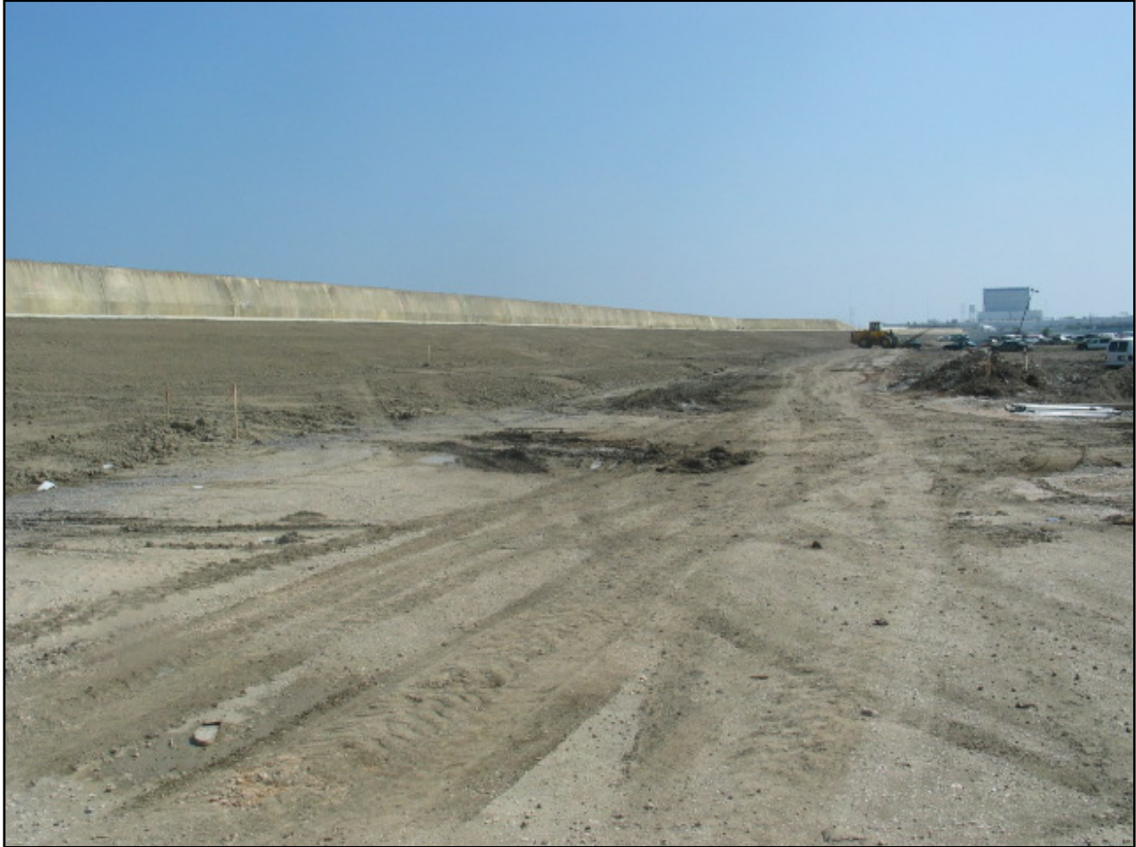
Figure NOE 32. West Floodwall Repairs around Michoud Canal (Note scour pad at base of wall and increased stability berm)
