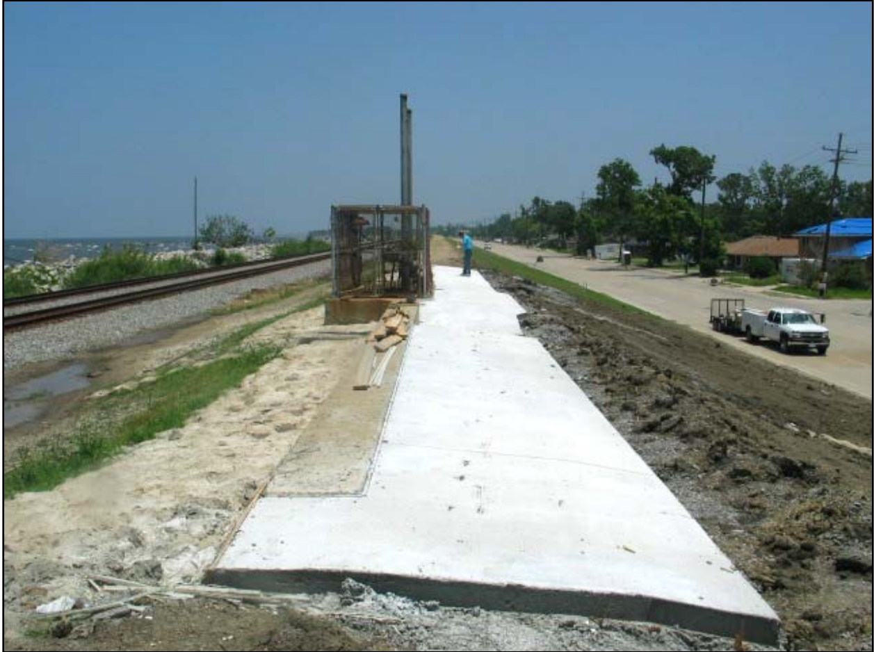
Figure NOE 25. Transition Improvements at Jahncke Pump Station (Note: refer back to Figure NOE 7 taken from same location)
