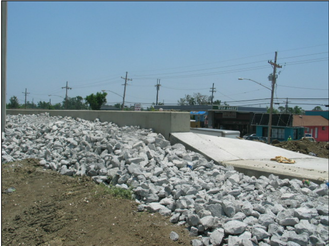
Figure NOE 24. Transition Improvements Between Reaches NOE 4&5 (Note: refer back to Figure NOE 6 taken from same location)
