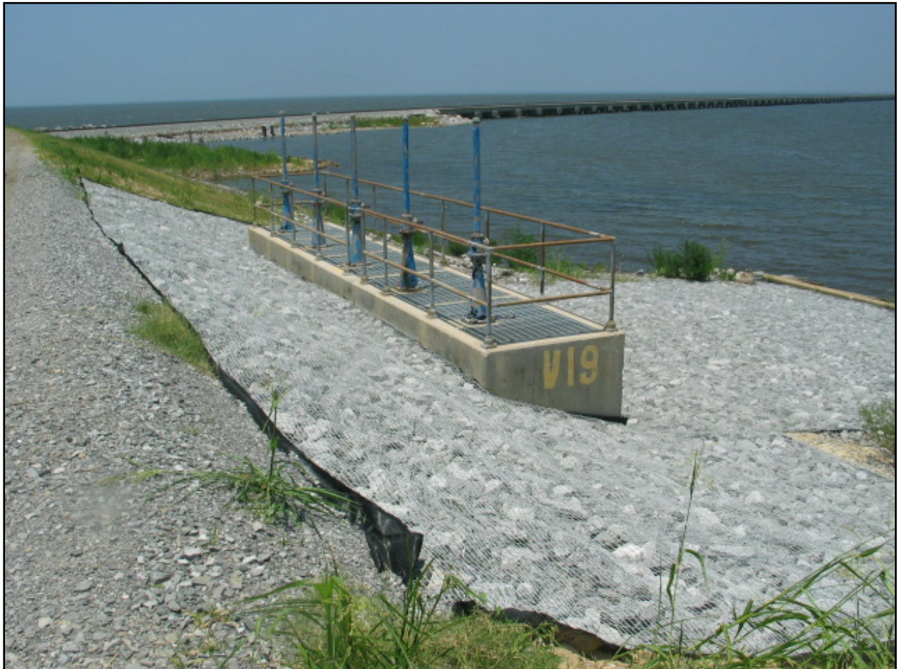
Figure NOE 27. Scour Repairs to Drainage Structure Headwalls (Note: Reach NOE10 drainage structure repairs – typical)
