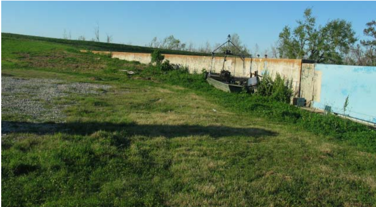
Figure STB 19. Caernarvon Canal Floodwall tie-in to higher MRL (gate is for Highway 39 closure)
