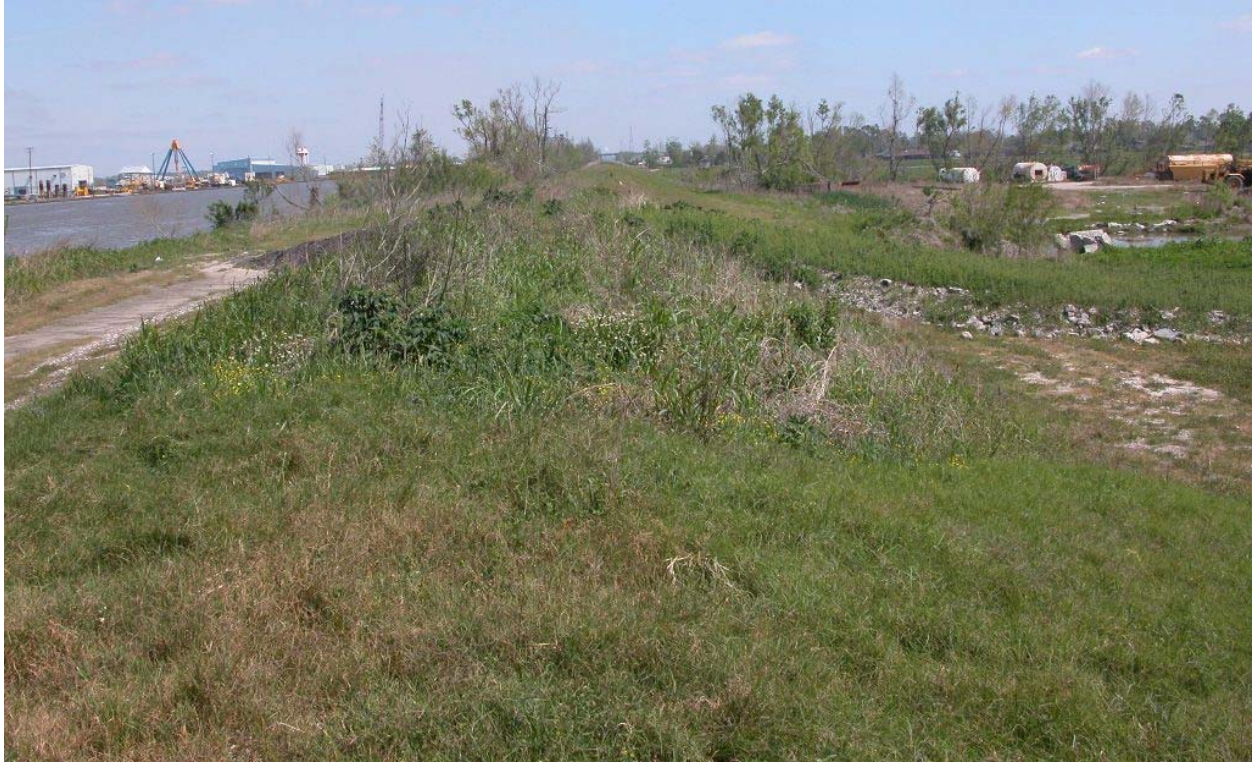
A point of levee erosion along the GIWW, however most is in good condition
