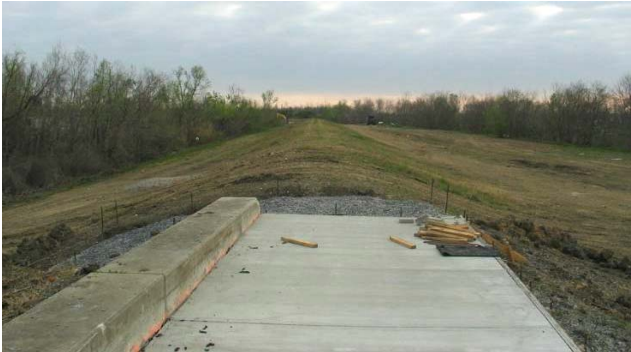
Figure STB 9. Beginning of Reach STB5 at end of I-wall (Note TFG improvements to Reach STB4 in foreground)
