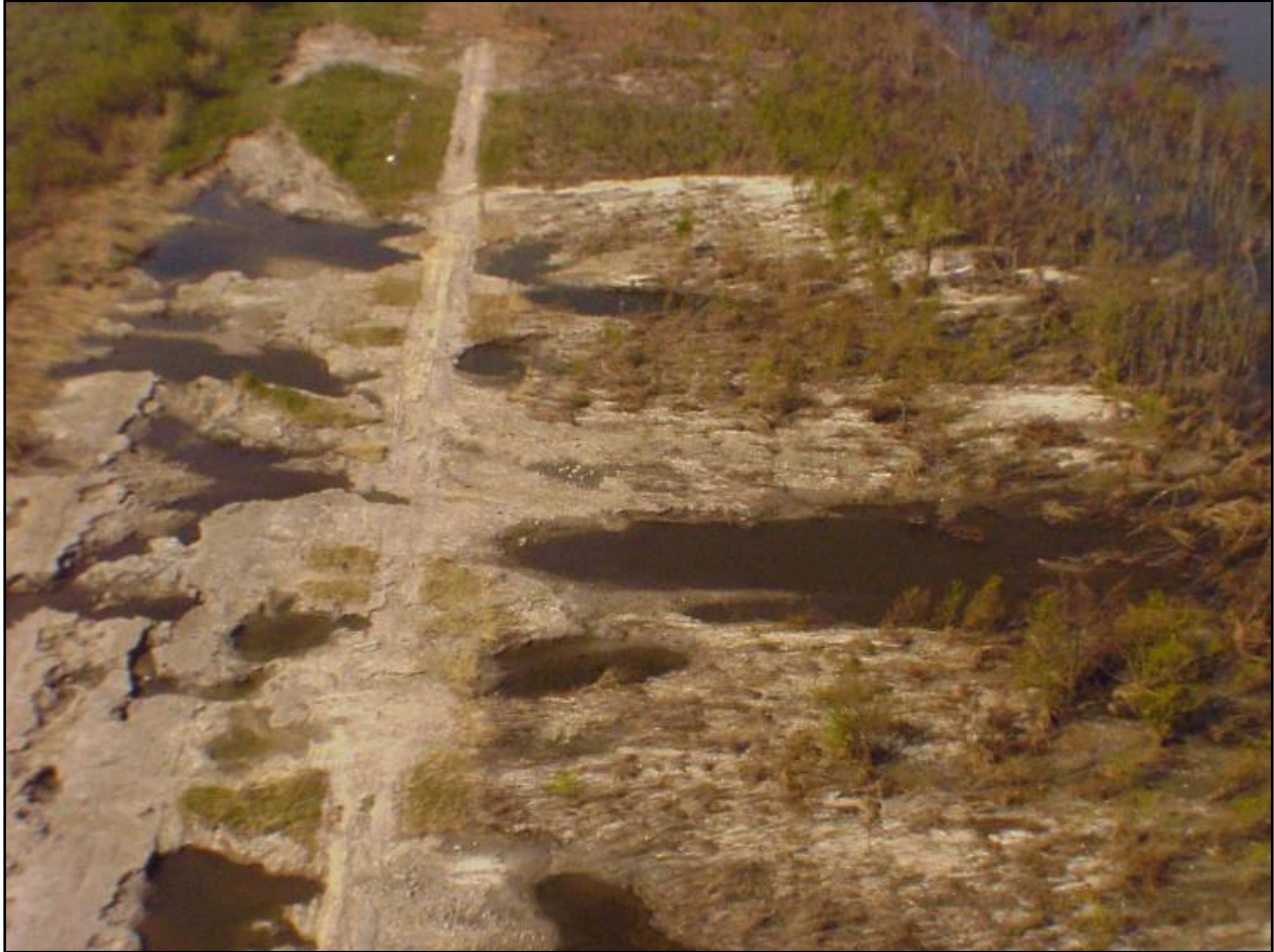
Figure NOE 11. Failure of Levee by Overtopping East of Pump Station #15 (East Back Levee)
