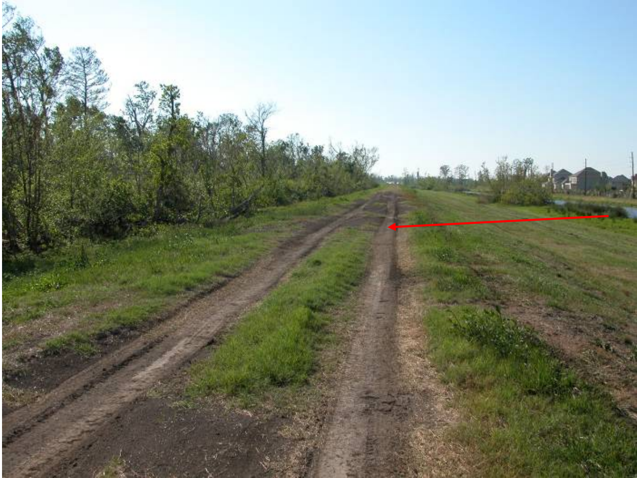
Back levee continues outside US Coast Guard toward GIWW Station. Crown is rutted
