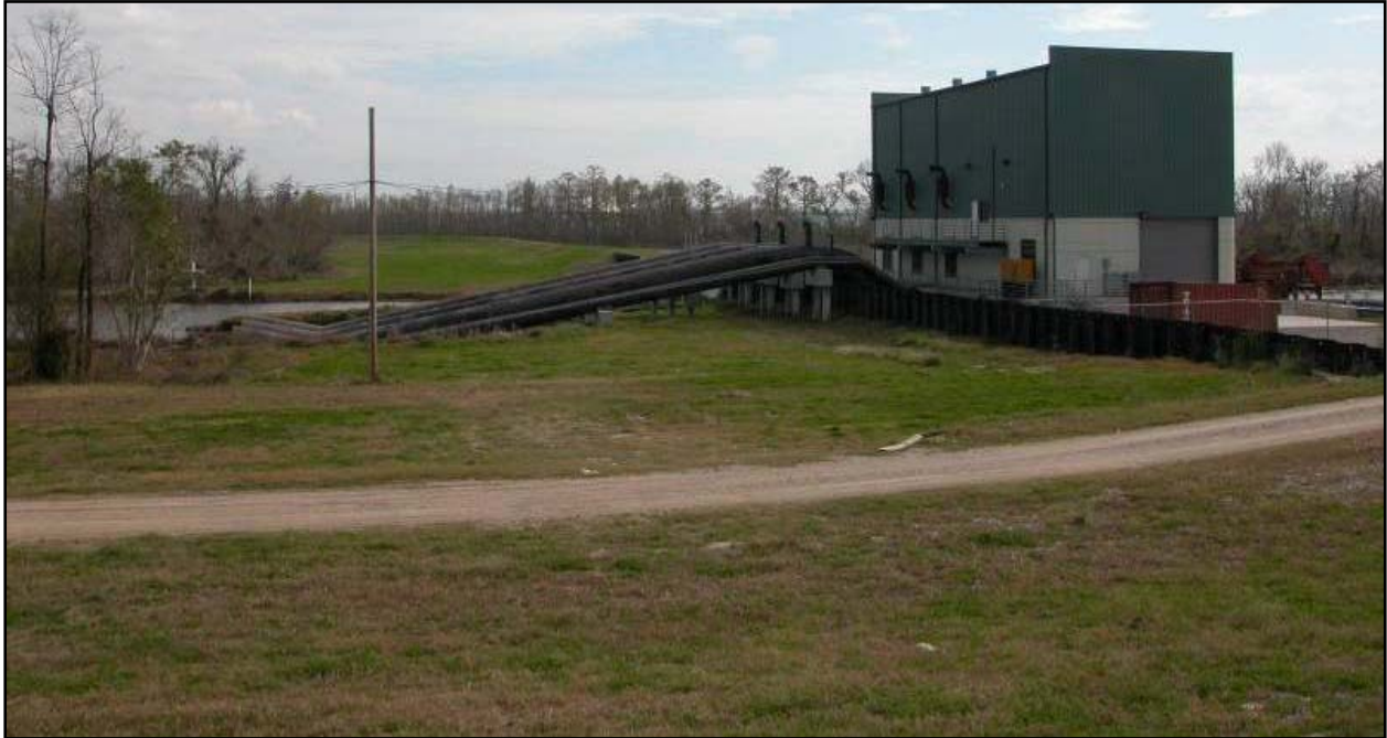
Figure 18. Local pump station.
