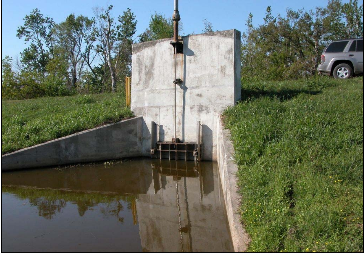
Figure 17. Local drainage structure.
