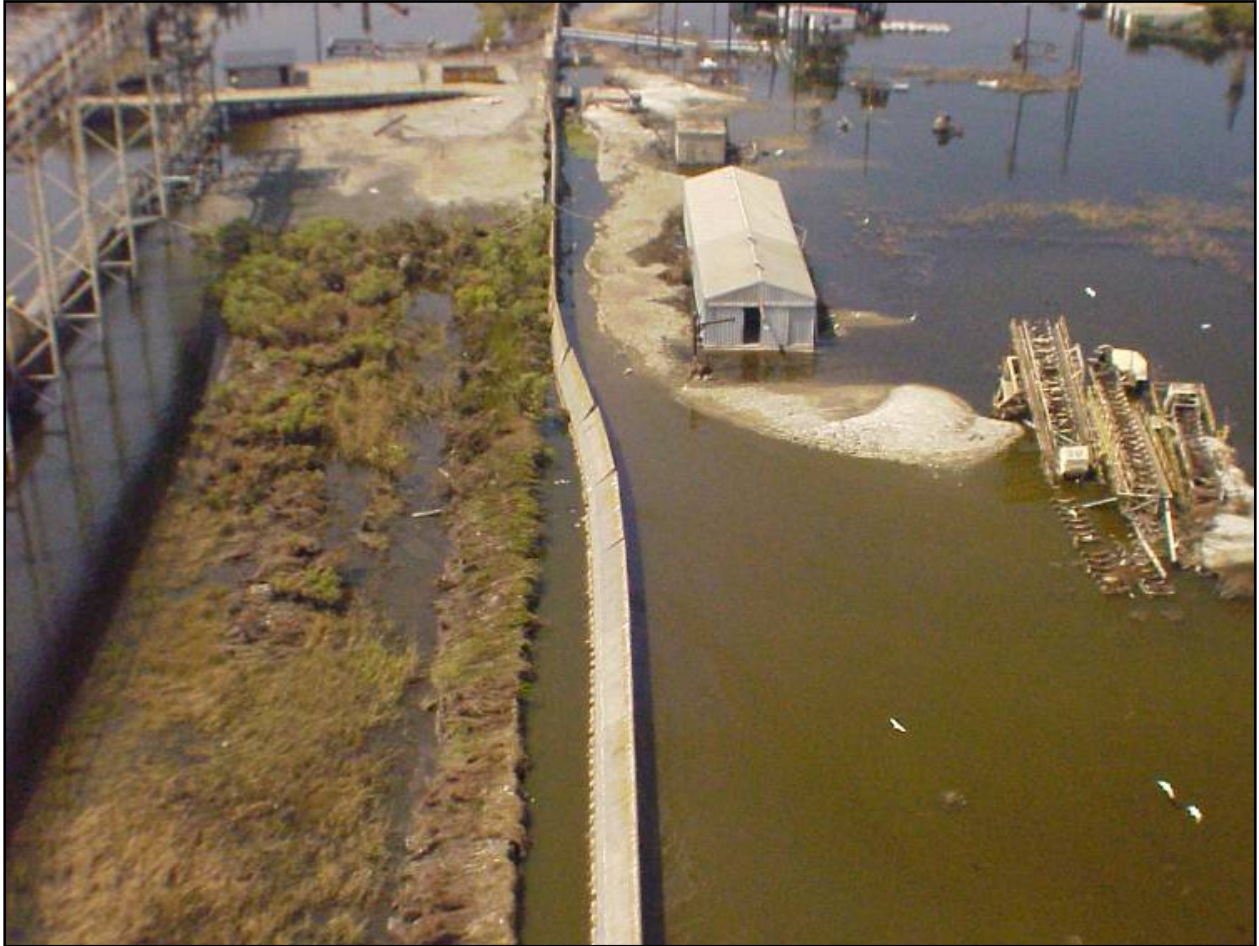
Figure 11. Katrina damaged I-wall.
