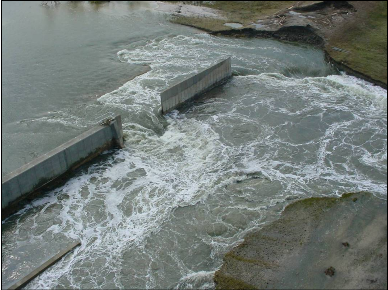
Figure 20. Katrina erosion at transition.
