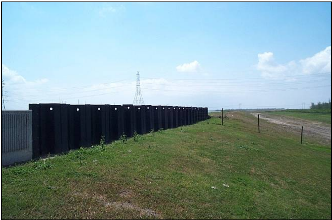
Sheetpile wall transition to concrete capped I-wall at the Segnette State Park
